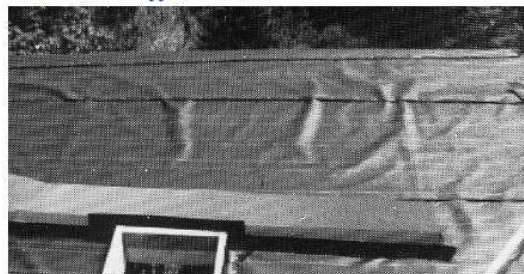
Conventional organic felts can absorb moisture, causing severe buckling and wrinkling.
