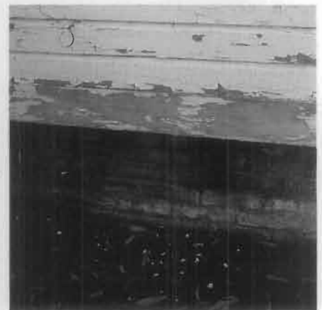
Figure 7. Chalking exterior paint can cause dangerous lead levels in soil around a house. Lead levels are usually highest in the one foot wide area adjacent to the building foundation. In these cases, the existing soil should be replaced with new soil or sod. This is particularly important if children and small pets play in contaminated areas, then inadvertently track the dirt inside.
