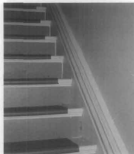
Figure 21. Painted stairs and floors can cause a problem because lead dust settles between the wooden boards. In this case, the steps were sanded, repainted, and covered with rubber stair treads. The floors could not be effectively cleaned and sealed so they were isolated with a new subflooring, and a washable tile finish installed.
