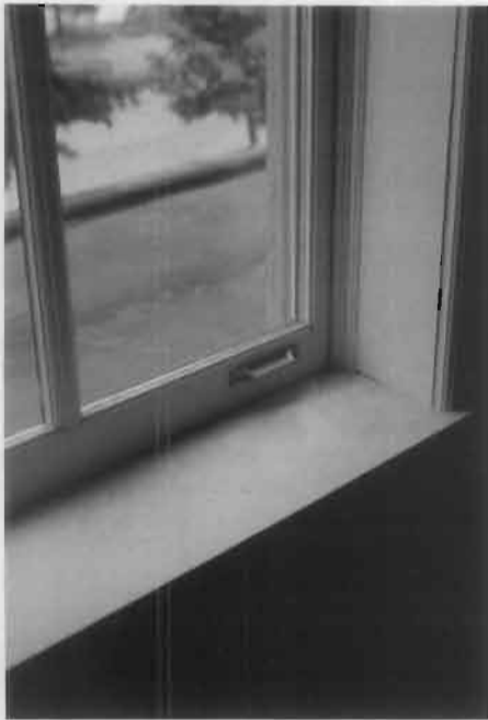
Figure 22. Research has shown that some small children will chew on projecting window sills while teething. As part of a lead hazard control project, the edge of the sill can be stripped to bare wood or an encapsulating paint applied. In this case, a new window sill was installed as part of a window upgrade that retained the historic trim and frame.
