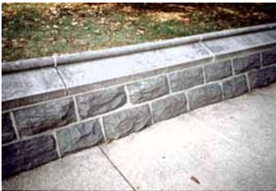
Caulking was inappropriately used here in place of mortar on the top of the wall. As a result, it has not been durable. Photo: NPS files.
