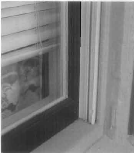
Figure 20. Operable windows have friction surfaces between the sash and the frames, which can be a source of fine lead dust. In this case, the deteriorated sash was replaced, but the historic frame remains in place, successfully isolated from the sash with a simple vinyl jamb liner that is part of the new sash operation.
