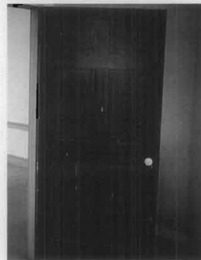
Figure 3. Significant architectural features and their finishes should not be removed during a project incorporating lead hazard controls. If the decorative stenciling above, or hand grained doors below, or painted murals need repair, then a paint conservator should be consulted. Once loose paint is consolidated or otherwise stabilized, a clear finish or other reversible clear protective surface or coating can be added to areas subject to impact or abrasion. Photos: NPS Files.
