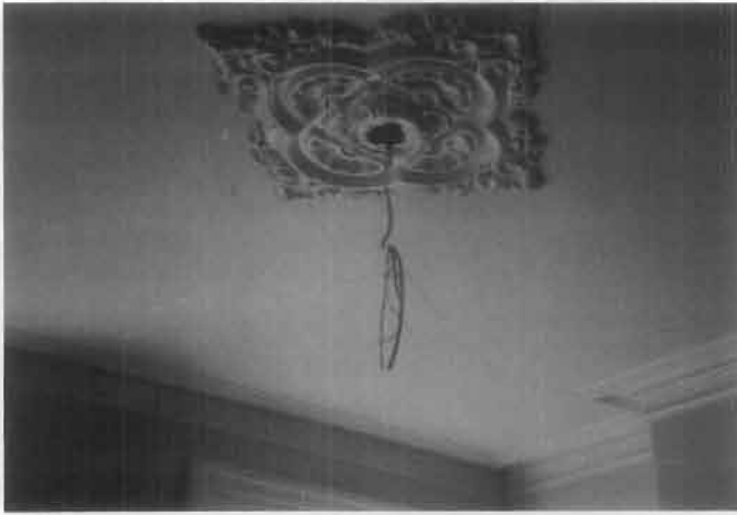
Figure 26. Deteriorated ceiling plaster was removed and a new drywall ceiling installed. The historic ceiling medallion was preserved, and the plaster cornices repaired in place. Photo: Landmarks Design Associates.
