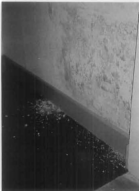
Figure 27. Wall leaks can cause historic surfaces to deteriorate, thereby exposing underlayers of lead-based paint. If painted surfaces show signs of deterioration, they should be repaired as soon as possible.
