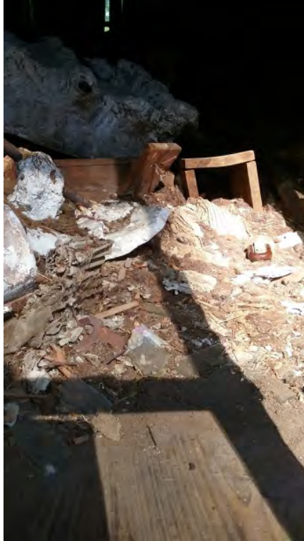
Pipe Insulation Debris at the Barn Attic
