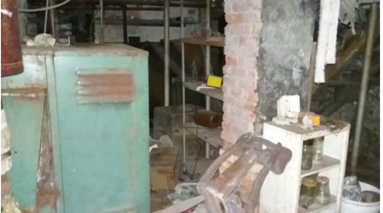
Damaged Basement Pipe Insulation Hanging and Drop on Floors
