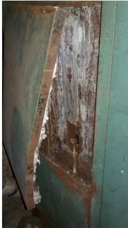
Basement Boiler Interior
