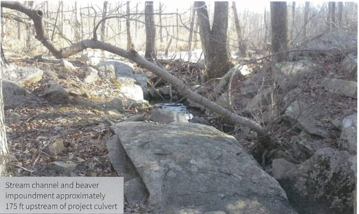
Culvert inlet and vicinity, area upstream was flooded due to a beaver impoundment
