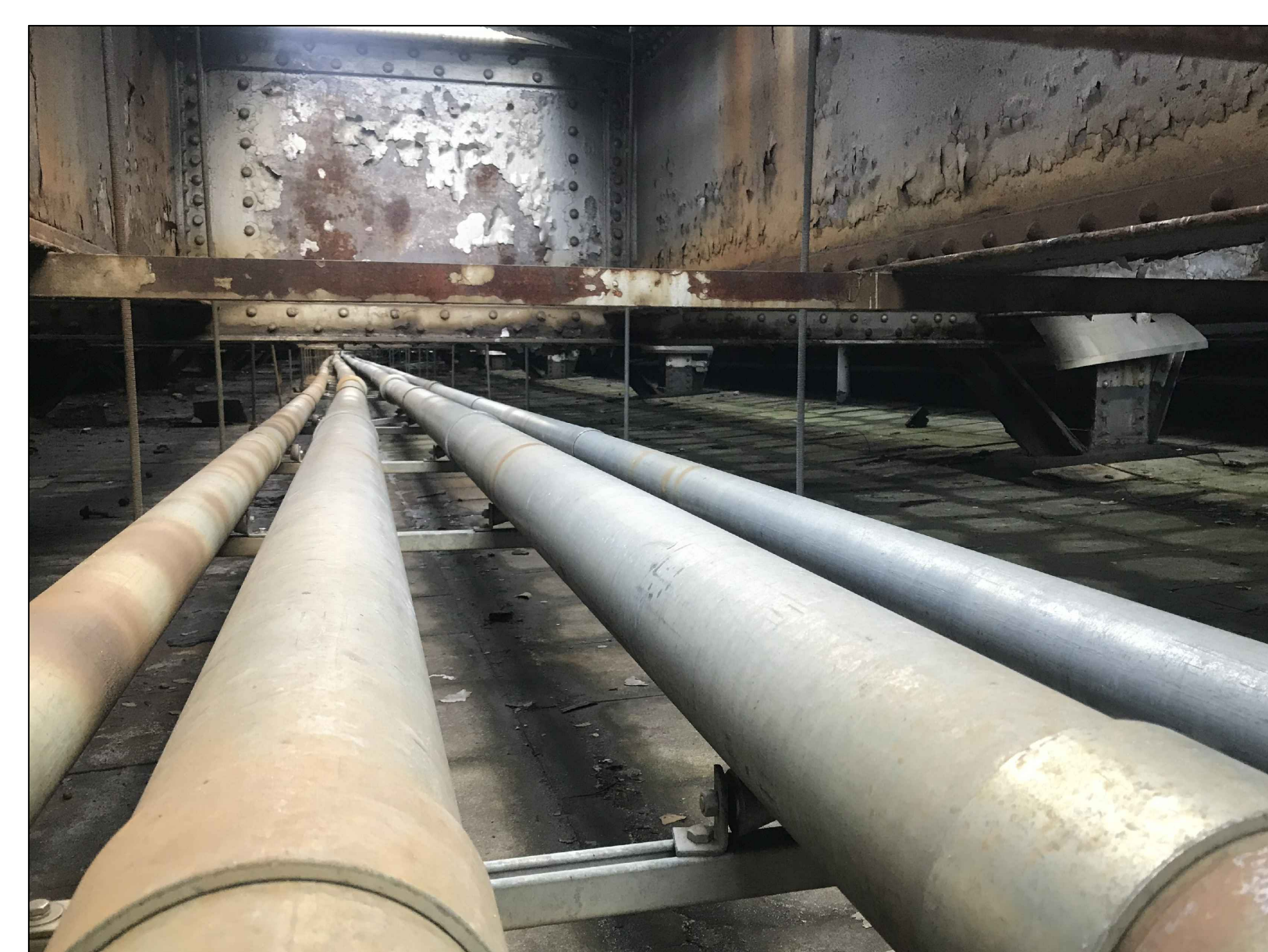
OVERVIEW OF ROOF SHOWING LOW-HANGING PIPES BENEATH TRAIN TRACKS
