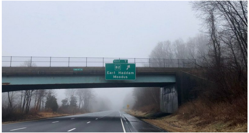
009S-026-10.68A bridge mounted
