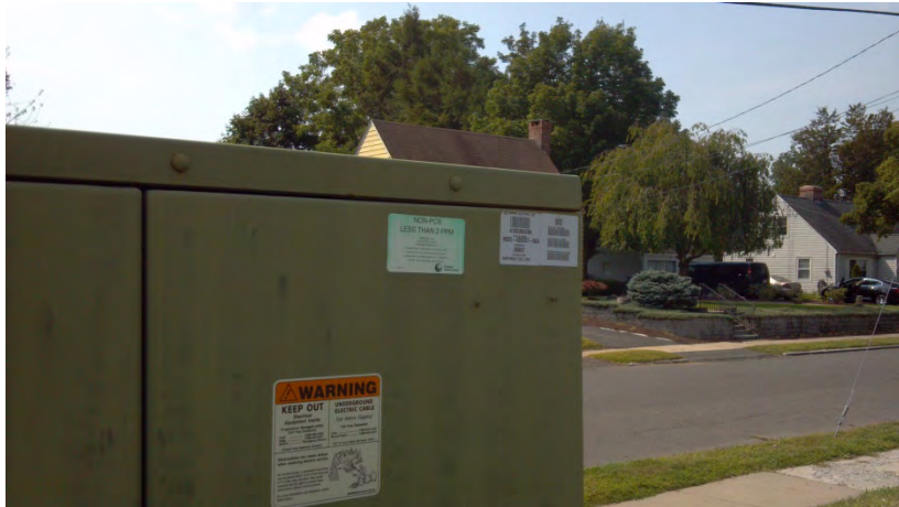
Photo 6: Transformer showing non-PCB label
