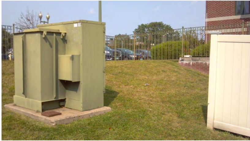
Photo 5: Transformer, looking northwest
