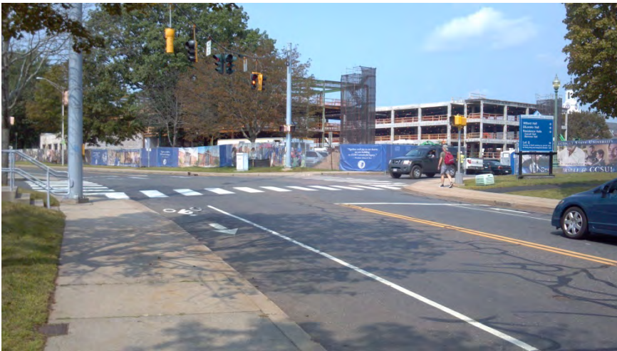
Photo 9: View of construction on CCSU campus, looking northwest along Paul Manafort Drive
