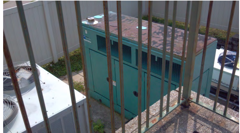
Photo 7: Stand-by generator within enclosure
