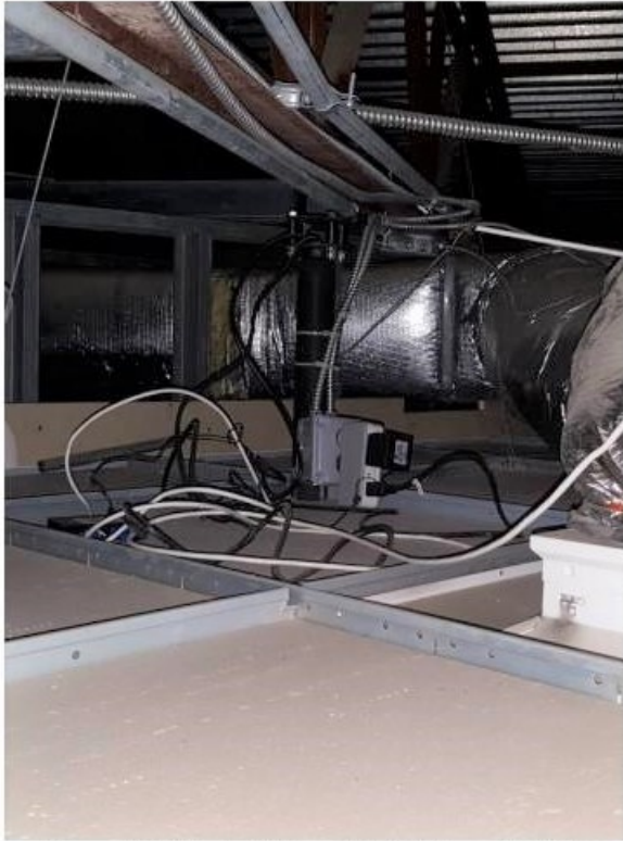
Figure 11: Typical Receptacle Above Ceiling
