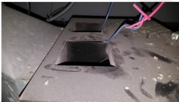
Figure 9: Exhaust Fan Exhausting into Ceiling Plenum
