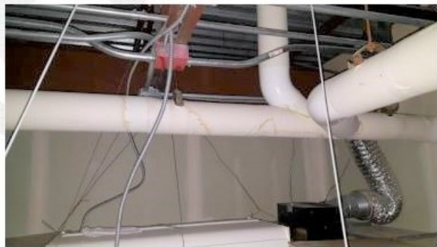
Figure 14: Storm Piping Water Damage in Employee Men's Room
