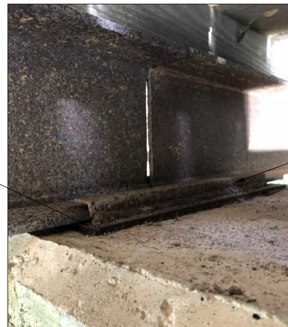
BEAM BEARING CONDITION
