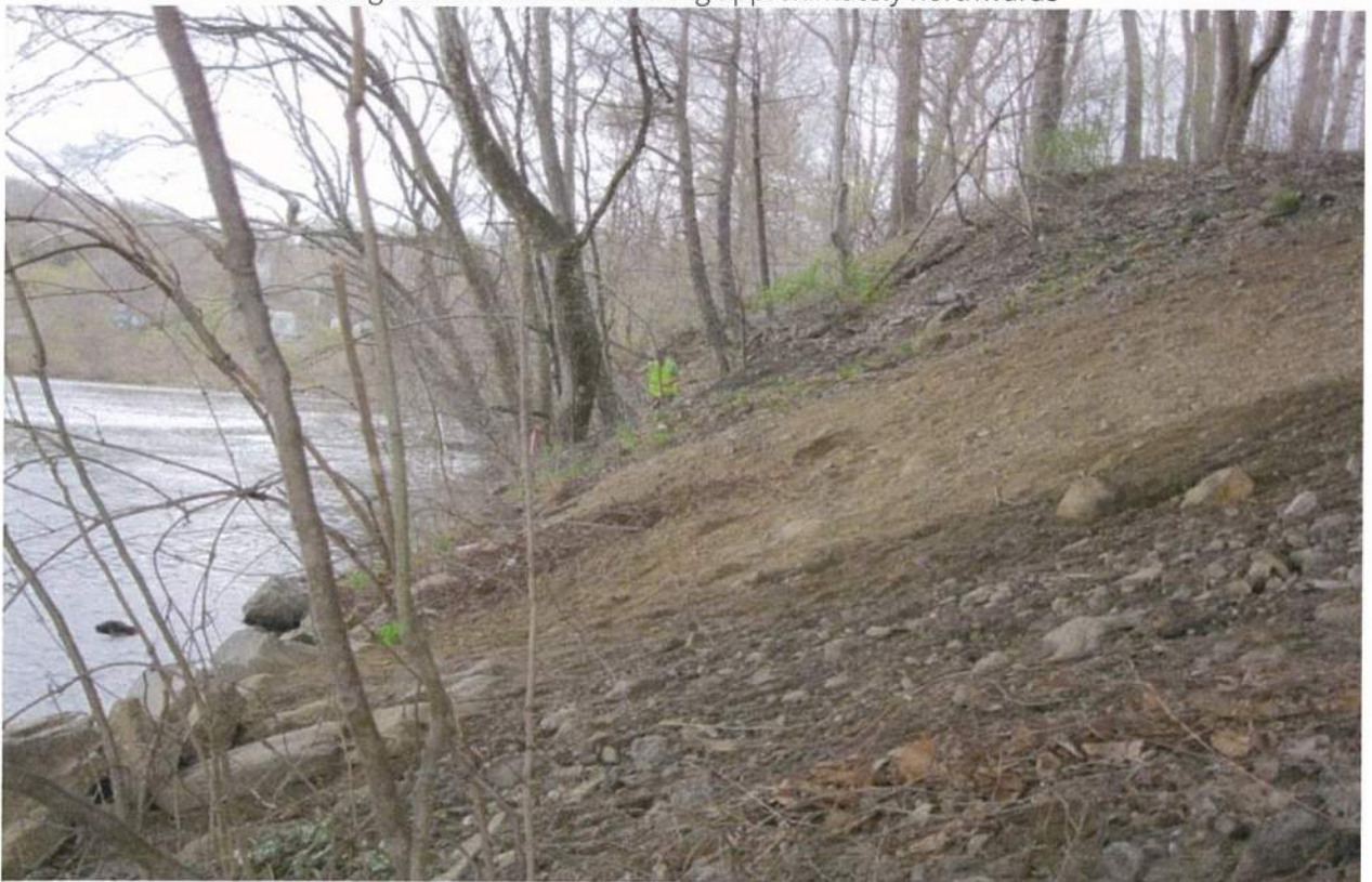
The edge of the Housatonic River (Lake Zoar) under Bridge 01218. Some areas include stone stabilization and others do not.
