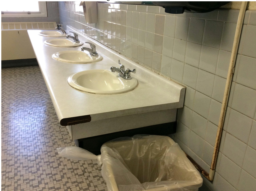
Asbestos-containing white caulking at sink unit counter in Boys' Lavatory
