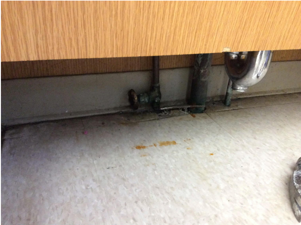
Assumed asbestos-containing air cell at concrete floor plumbing penetration
