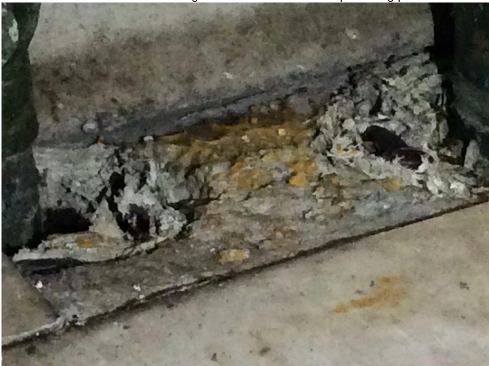
Assumed air cell pipe insulation at concrete floor pipe penetration (close up)
