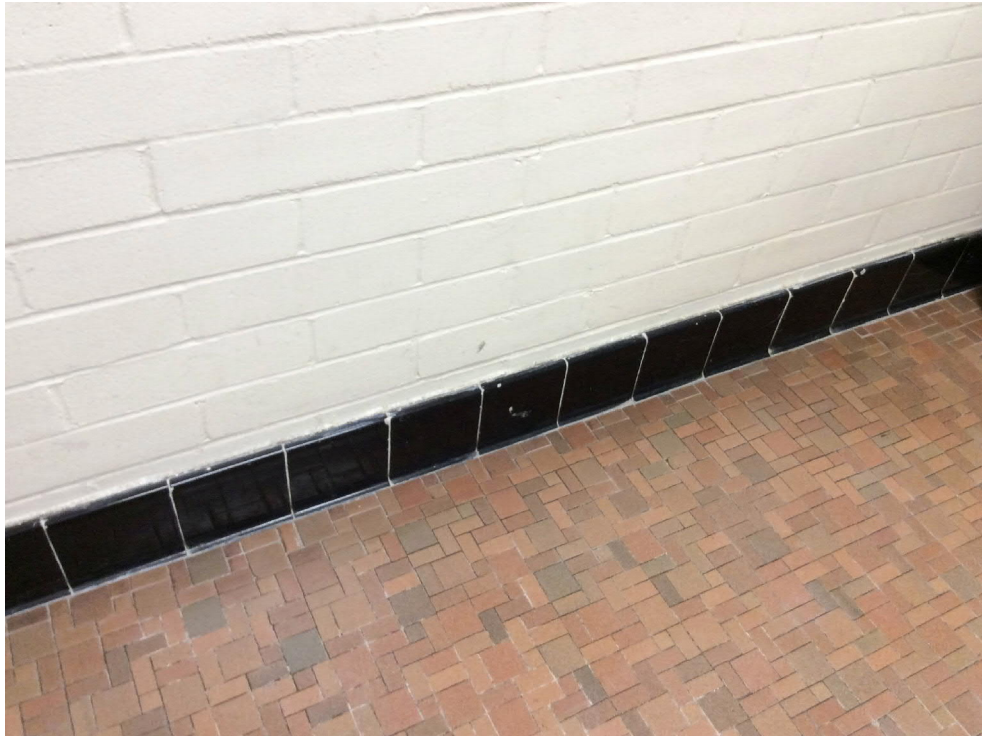
Lead containing black ceramic cove base tiles
