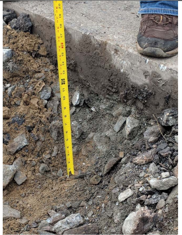
Bridge 02932, T-1-2, facing southeast Thickness of existing asphalt and soil above bridge deck
