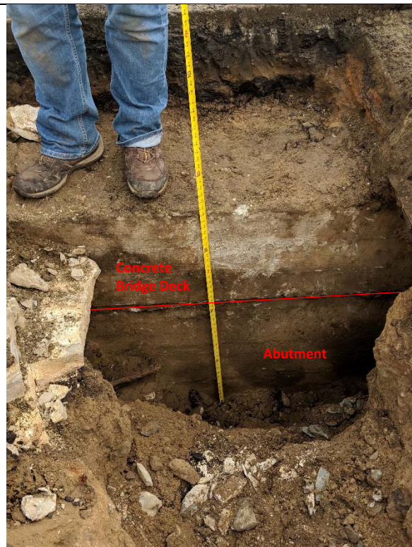
Bridge 02931, Test Pit T-2-1, facing east. Thickness of bridge deck and depth of test pit.
