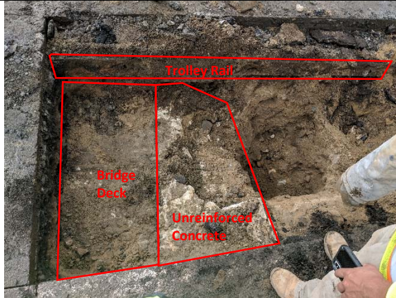
Bridge 02931, Test Pit T-2-1, facing south, looking down. Top of exposed bridge deck, unreinforced concrete behind bridge deck, trolley rail exposed.
