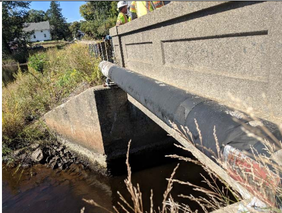
Bridge 02931, facing west Cracks along western face of bridge
