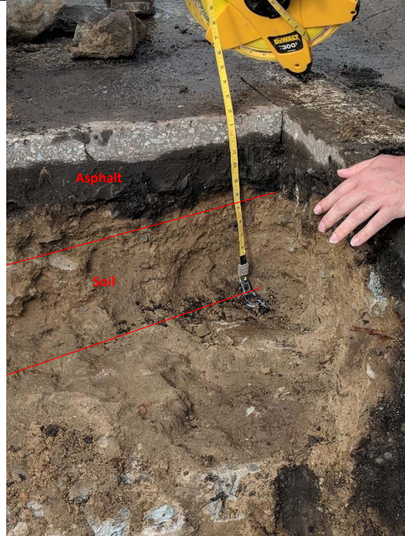
Bridge 02931, Test Pit T-2-2, facing west. Thickness of asphalt and soil above bridge deck.
