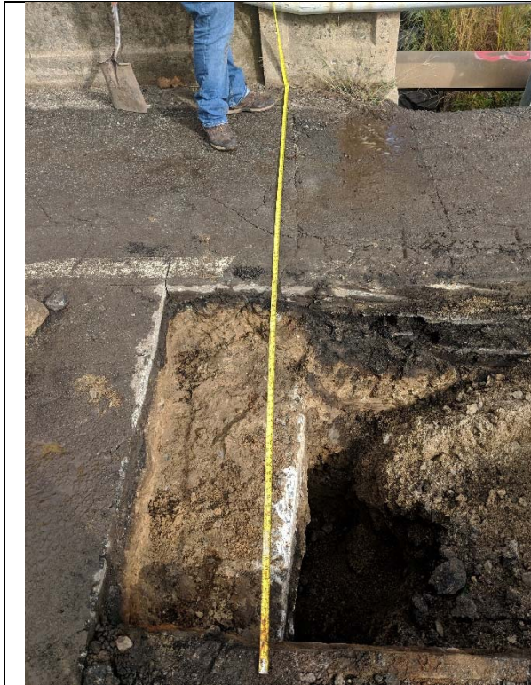
Bridge 02931, Test Pit T-2-2, facing north, looking down. Test pit during excavation.
