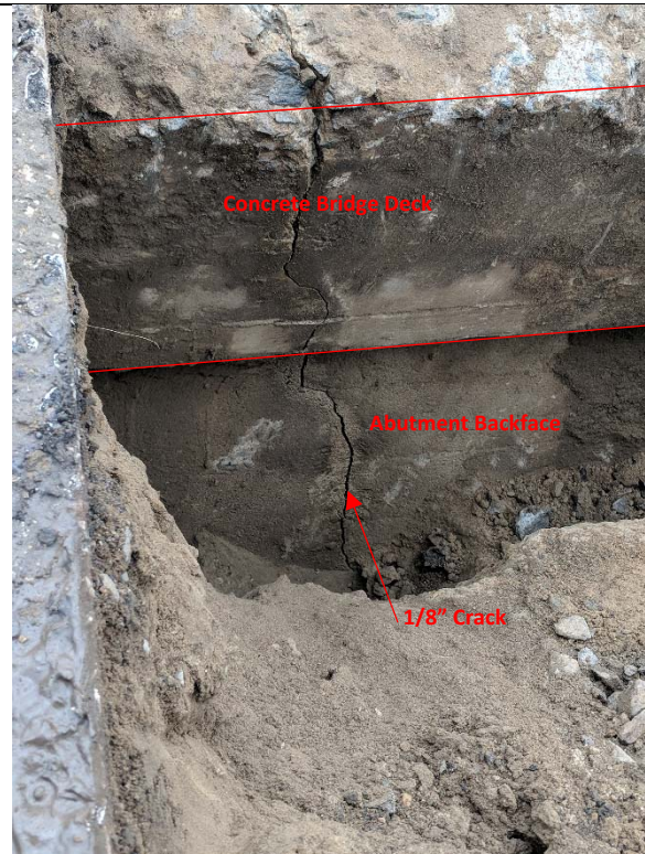
Bridge 02931, Test Pit T-2-4, facing west, looking down. Crack running from bridge deck and through abutment.
