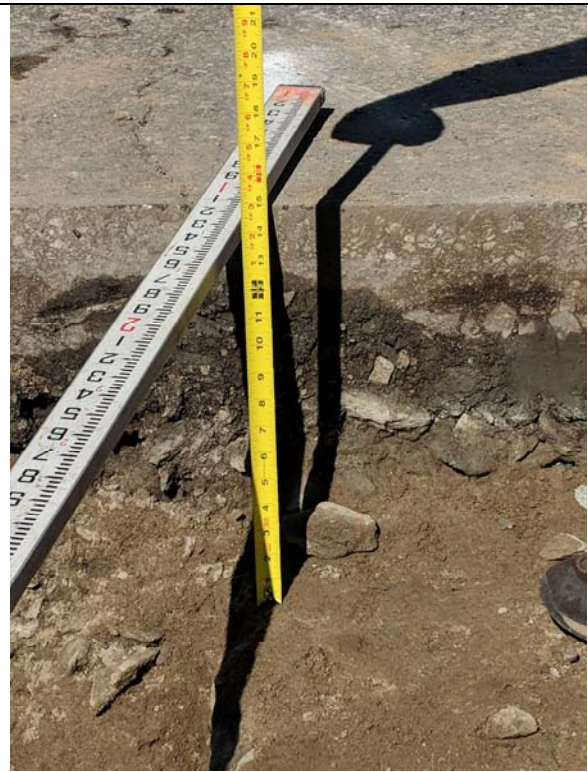
Bridge 02931, T-2-3, facing north Thickness of existing asphalt and soil above bridge deck
