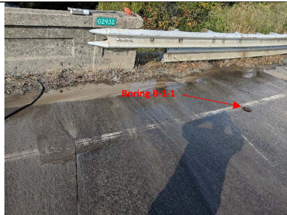
Bridge 02932, Test Pit T-1-2, facing north, looking down. General view of asphalt cut in relation to boring B-1-1.
