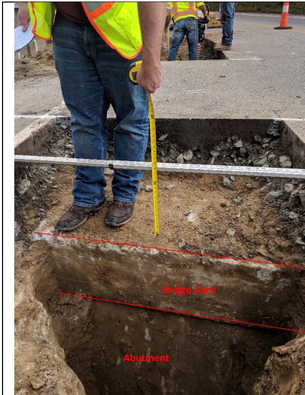
Bridge 02932, T-1-1, facing east Thickness of existing asphalt and soil above bridge deck
