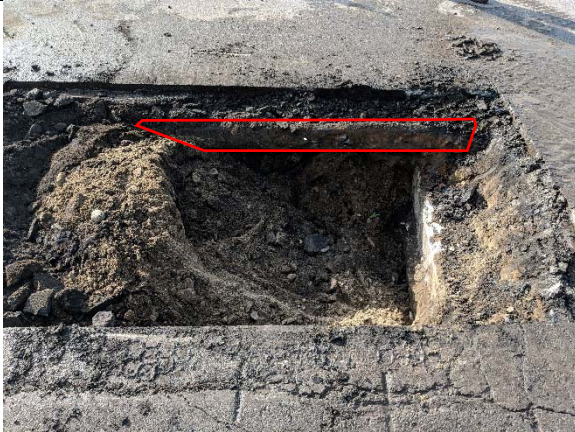
Bridge 02931, Test Pit T-2-2, facing south, looking down. Back of the abutment and exposed rail line.
