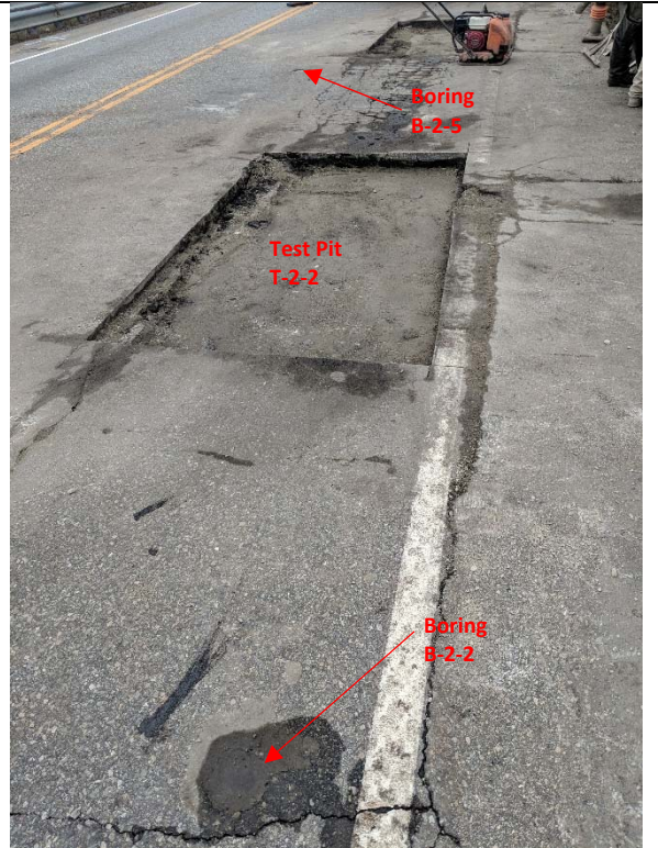
Bridge 02931, Test Pit T-2-2 (foreground) and T- 2-1 (background), facing west, looking down. Test pits in relation to borings B-2-3 (foreground) and B-2-5 (to the left of T-2-1).
