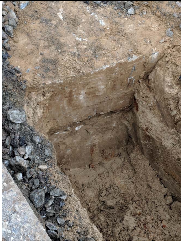
Bridge 02932, T-1-2, facing northwest General view of exposed bridge abutment and deck
