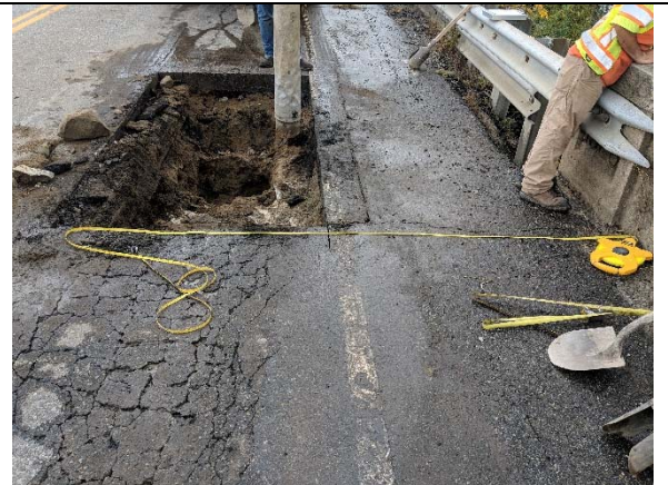
Bridge 02931, Test Pit T-2-1, facing west, looking down. Test pit during vacuum excavation.
