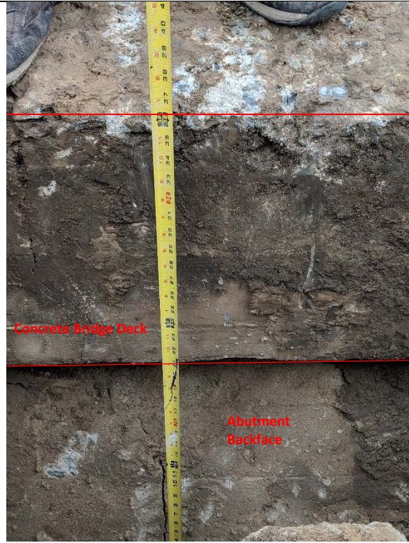
Bridge 02931, Test Pit T-2-4, facing west. Depth from bottom of test pit to the top of the concrete deck.
