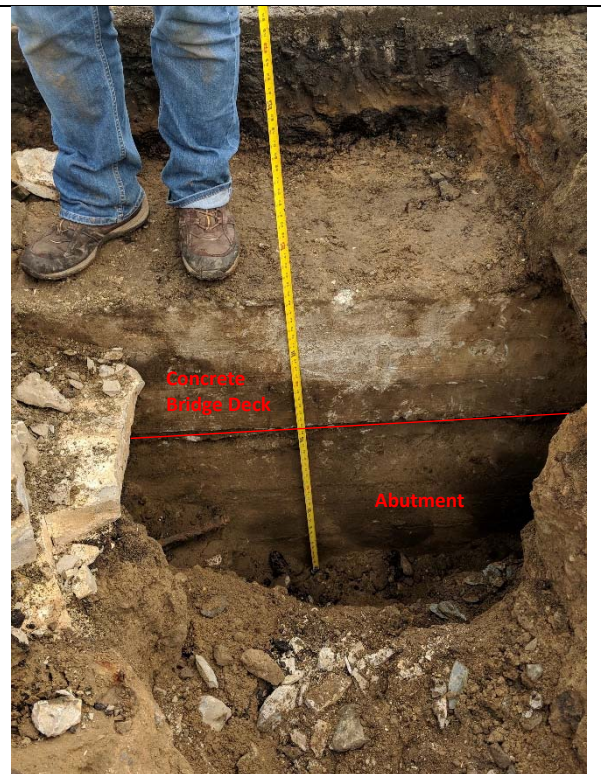
Bridge 02931, Test Pit T-2-1, facing east. Thickness of bridge deck and depth of test pit.
