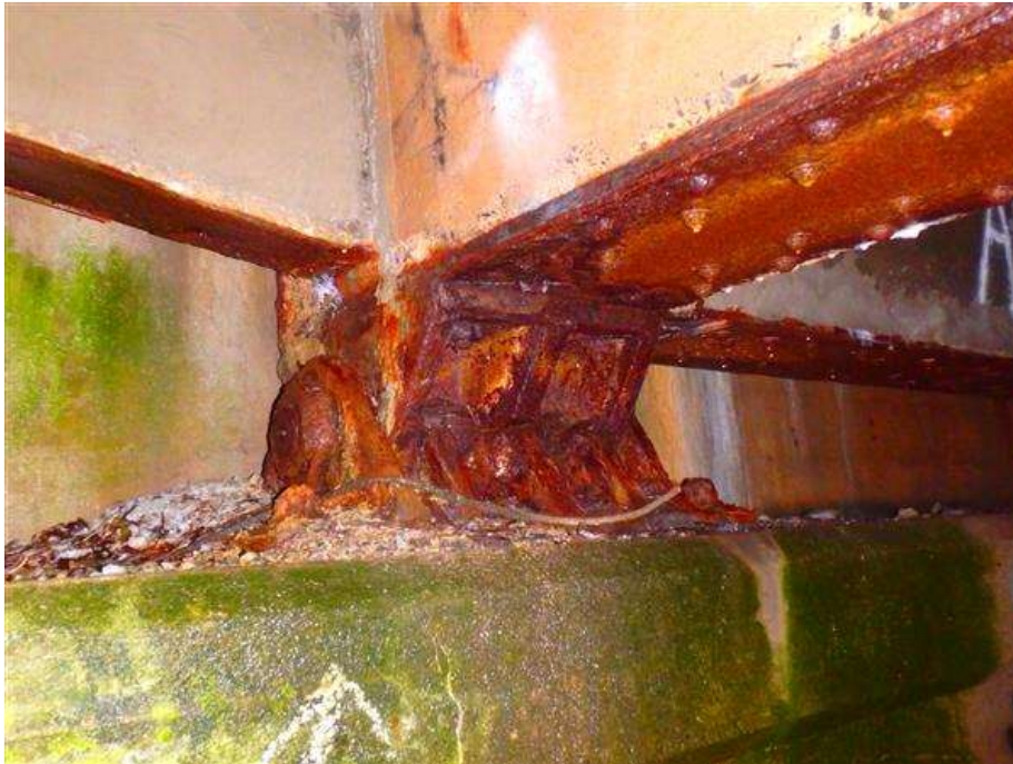
Girder G1 fixed bearing at abutment 2. Note the laminated rust and section loss at the bearing components. Also, note debris on the abutment seat.
