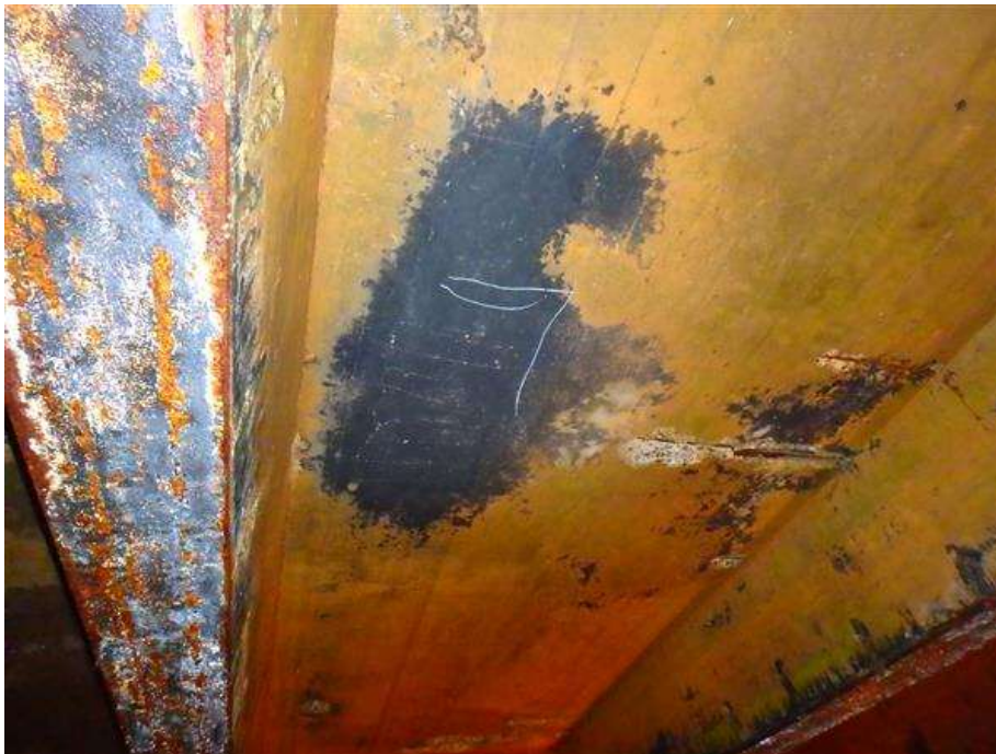
Underside of deck between floorbeams 3 and 4. Note the hollow area.
