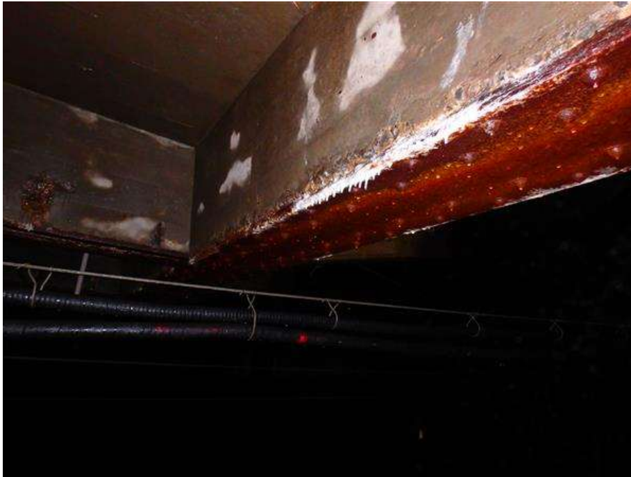
Girder G2 bottom flange near abutment 1. Note the efflorescence and the pack rust between plates.
