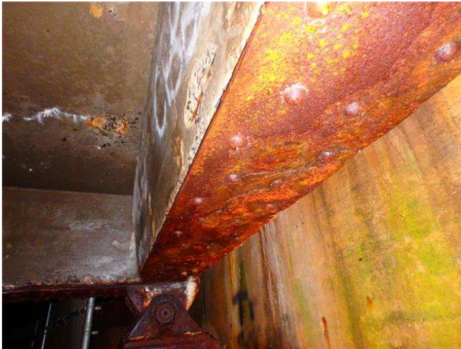
Underside of floorbeam 0. Note the section loss to the bottom flange and the rivets.
