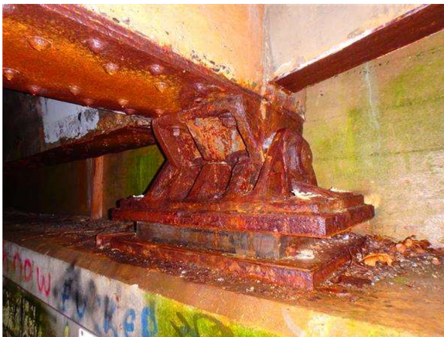
Girder G1 expansion bearing at abutment 1. Note the heavy rust and section loss at bearing components.
