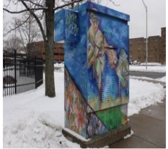
This traffic box is located on the corner of Franklin and Pearl Street.
