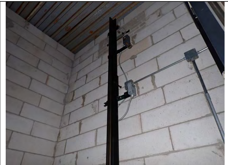
19 Elevator Guild Rails and Upper Limit Switches
