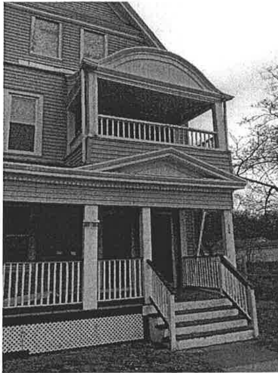
House street side exterior view. Roofing above ground level porch is asbestos containing.
