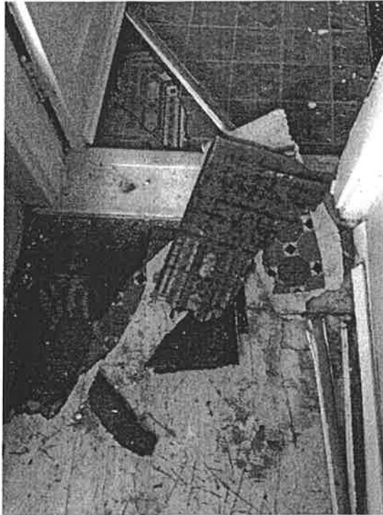
Multiple layers of sheet flooring over asbestos containing black adhesive in third floor storage room off kitchen
