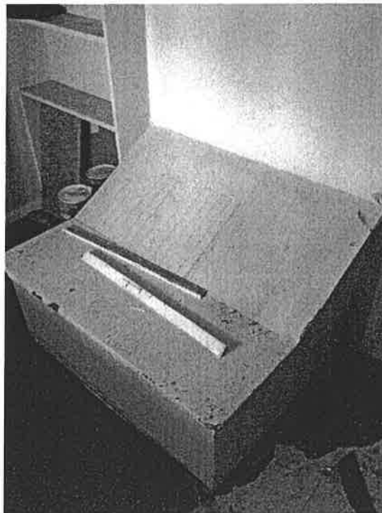
Third floor storage room cover of back stairway. Paint contains lead.
