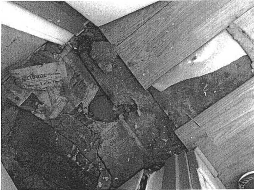
Many closets off bedrooms had multiple layers of sheet flooring and sometimes old newspapers as insulation
