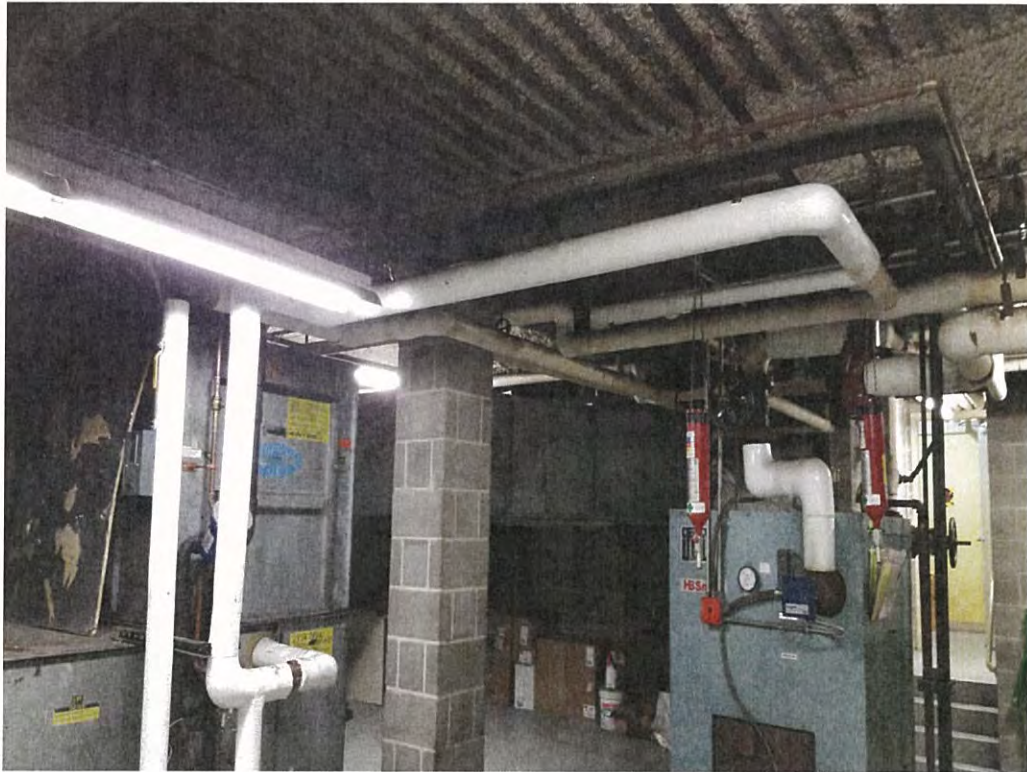
1977 Addition Boiler Room
