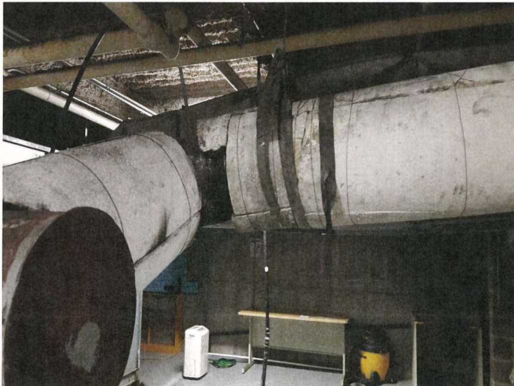
1977 Addition Old Boiler Line
