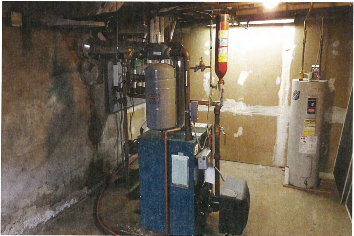
1837 House Boiler Room
