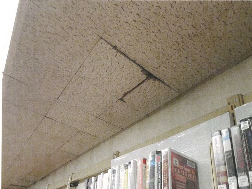
1977 Addition Ceiling Tile
