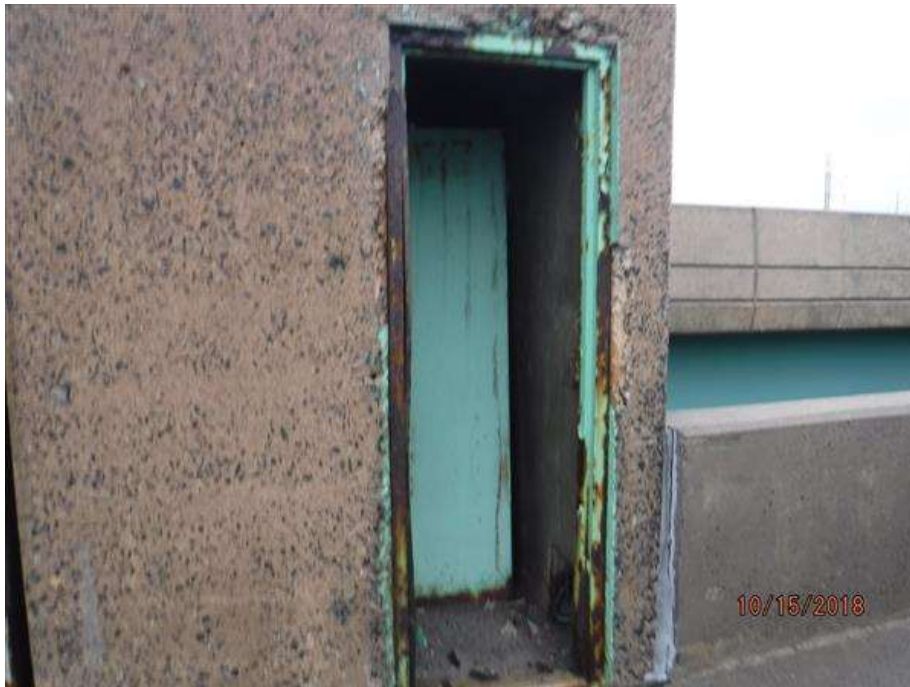
Girder 1 at the north end of span 7 with a broken access door.
