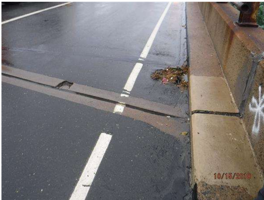
Clogged drain at pier 1 in span 2 along the east parapet and spall in concrete header.
