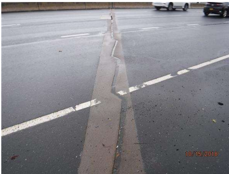
Pier 16 deck joint with missing joint material on the northbound side.
