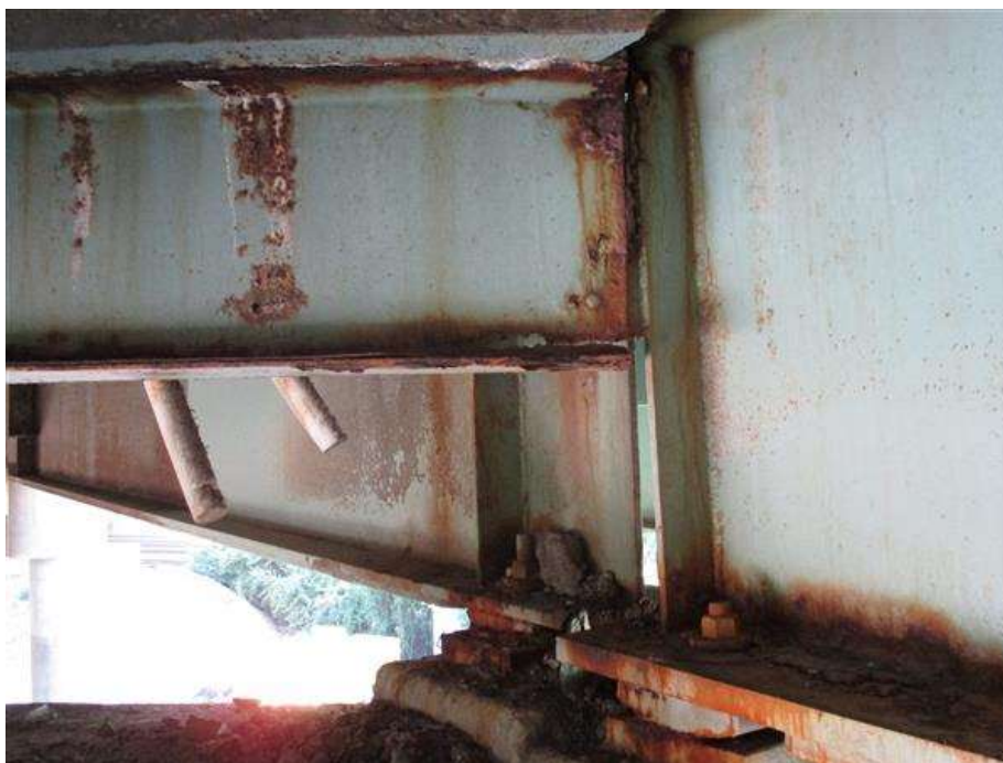
Span 16, bay 2 at pier 15 end diaphragm with areas of heavy rust and perforations in the bottom flange and web. Note the short weeps draining onto the pier cap.
