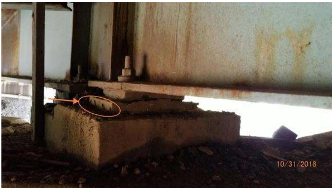
Girder 11 at pier 15 in span 15 with a gap under the bearing.
