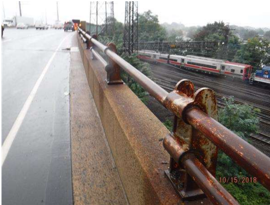
East parapet in span 1 with missing bottom rails.
