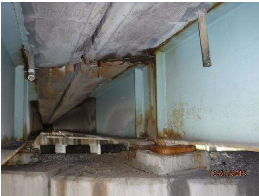
Short weeps in span 15, bay 7. Note the leakage from the median joint onto the superstructure and substructure.
