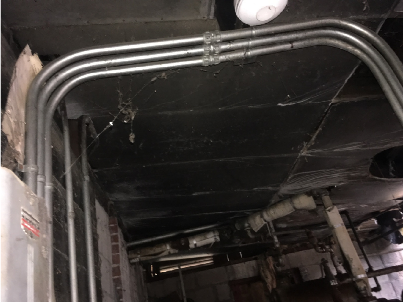
Asbestos containing ceiling and Pipe Wrap
