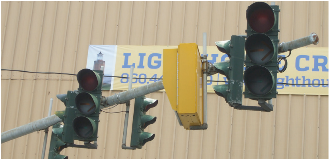
Traffic signal equipment on Ferry Street near the entrance to the Cross Sound Ferry facilities.
