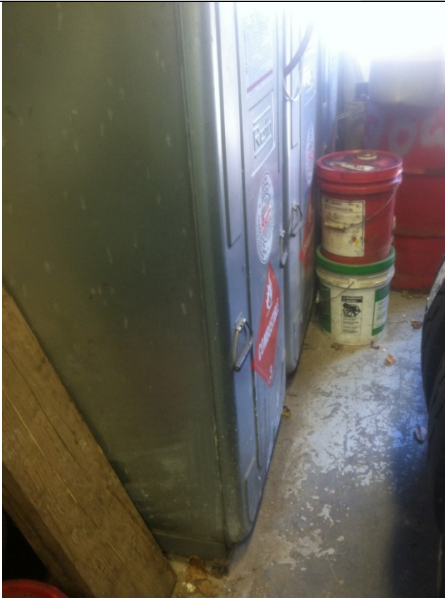
Photo Description: 275-gallon double walled AST in Oil Storage Room
