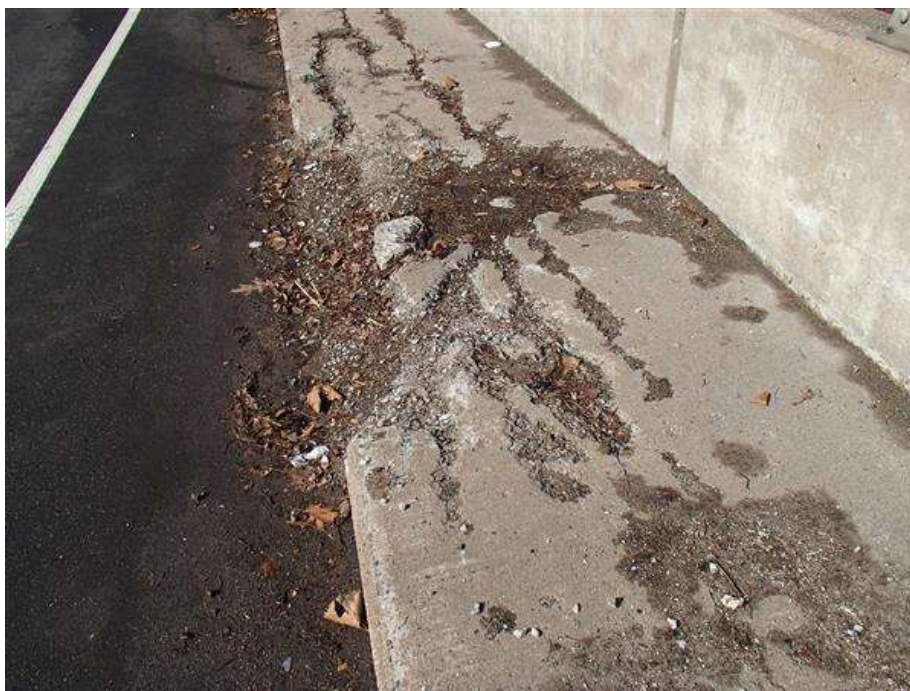
North sidewalk at the pier joint exhibits area of plow damage with longitudinal cracks, spalls, scale, loose concrete, and hollow areas.
