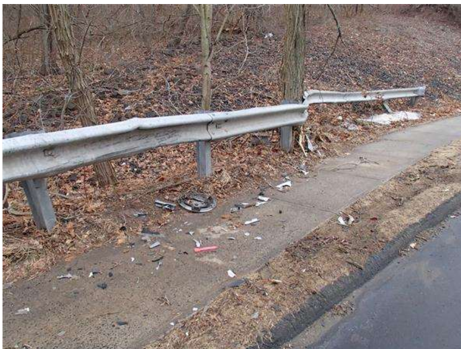
Metal beam guide rail at southwest approach corner exhibits collision damage with bent rail and broken/disconnected posts.
