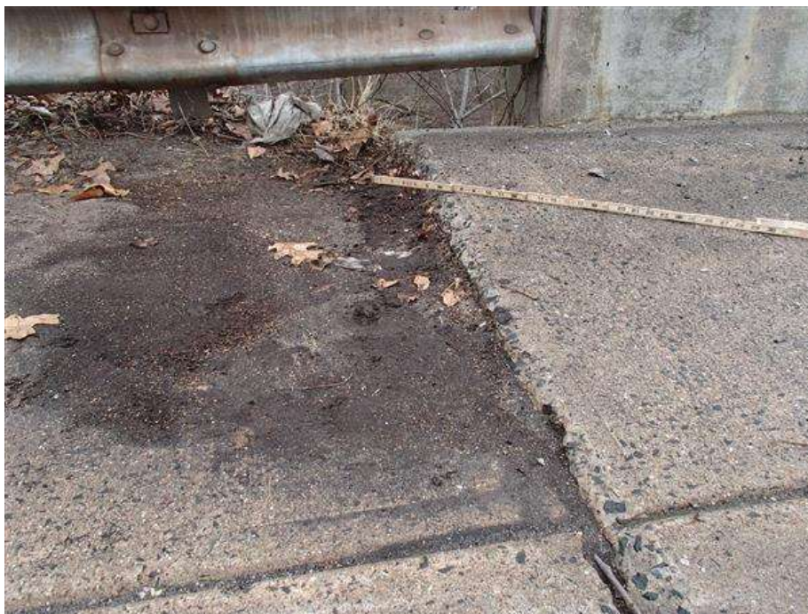
Southeast approach sidewalk exhibits vertical mis-alignment between segments (pedestrian tripping hazard).
