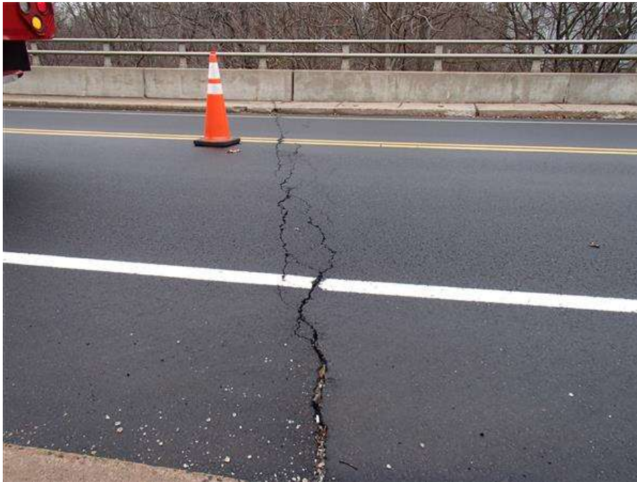
Bituminous concrete overlay (new since last inspection) over the abutment 2 joint exhibits transverse cracks.
