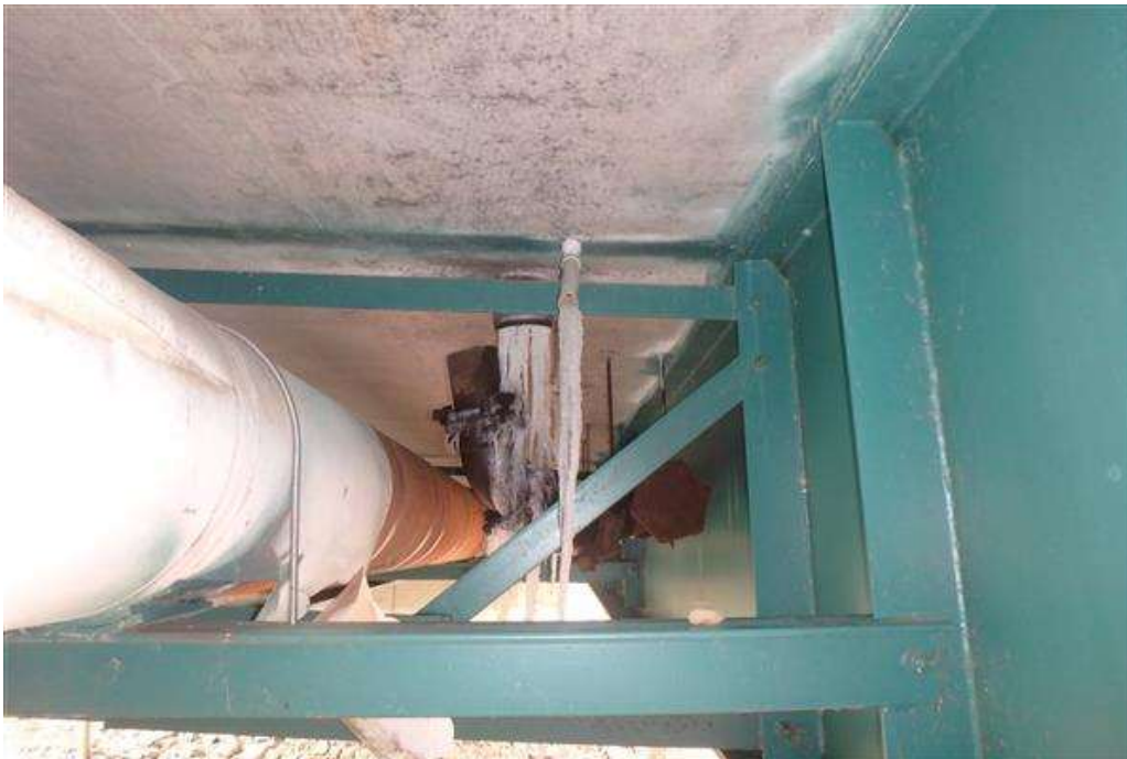
Scupper pipe with heavy surface rust and is disconnected from the coupling in span 1, bay 1. Note PVC weep with missing extension.
