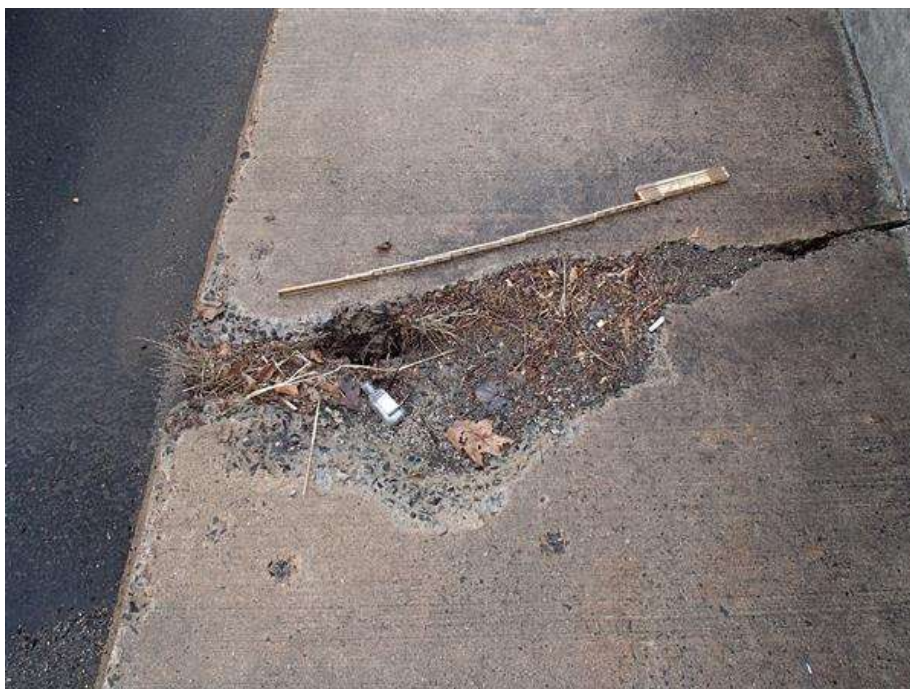
South sidewalk at the pier joint exhibits spall with hole through joint.
