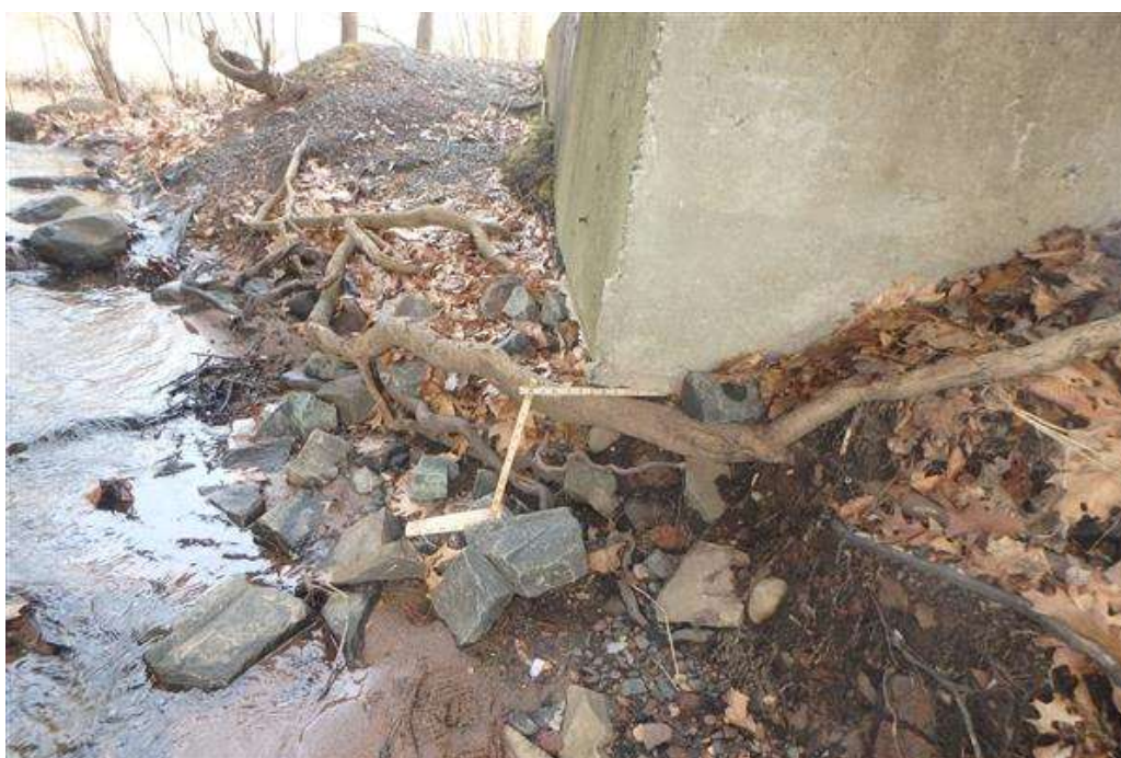
Pier, west elevation at the north exposed footing, exhibits area of scour causing undermining of the footing with tree root growth below (re-occurring condition; previously placed rip rap displaced).
