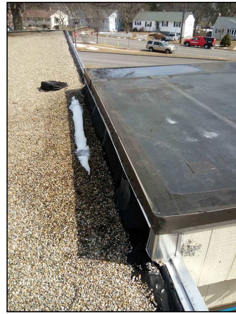
PHOTO B EXISTING RAISED ROOF AT PORTABLE CLASSROOM CONNECTOR TO EXISTING MAIN BUILDING LOCATION
