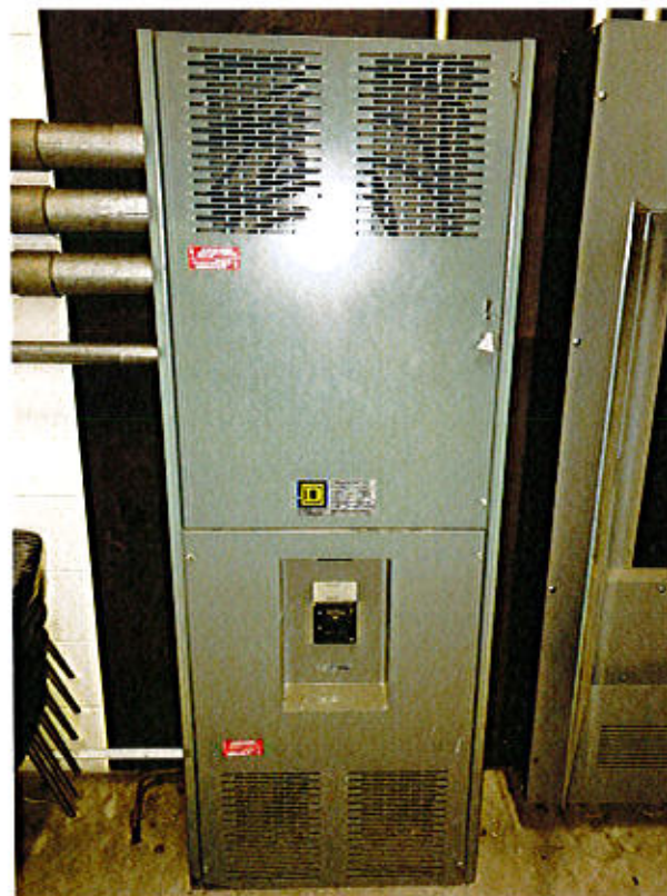
Generator room panel
