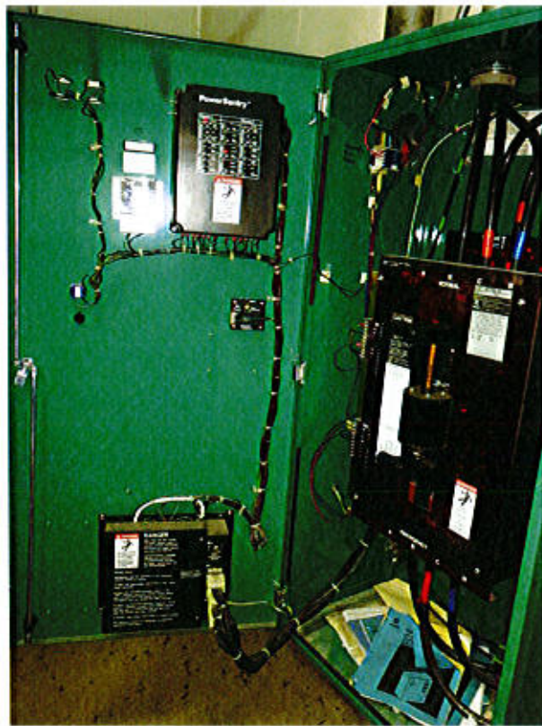
Inside generator control
