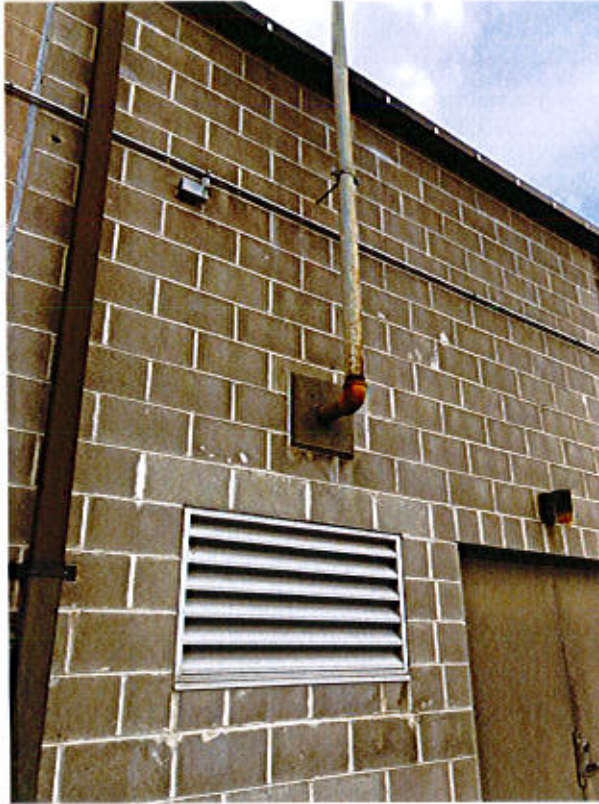
Generator room vent and generator exhaust
