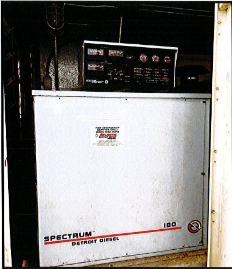
Photo 57. Hartford Bridge & Electrical Maintenance Facility – 49 Jennings Road, Hartford, CT Inside Generator.
