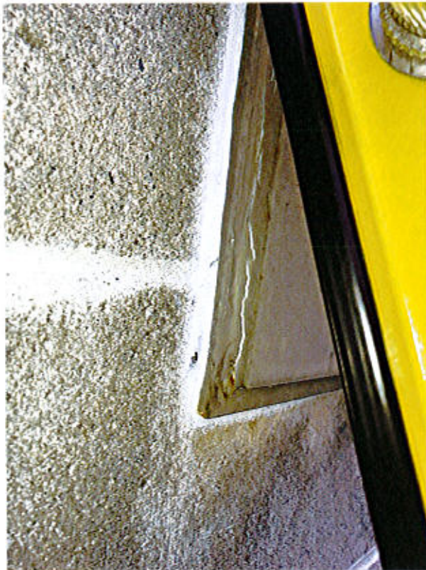
Generator exhaust caulk
