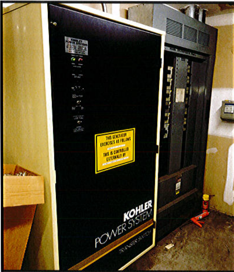
Photo 83. Rocky Hill Central Warehouse Facility – 600 Broad Street, Rocky Hill, CT. Generator Transfer.
