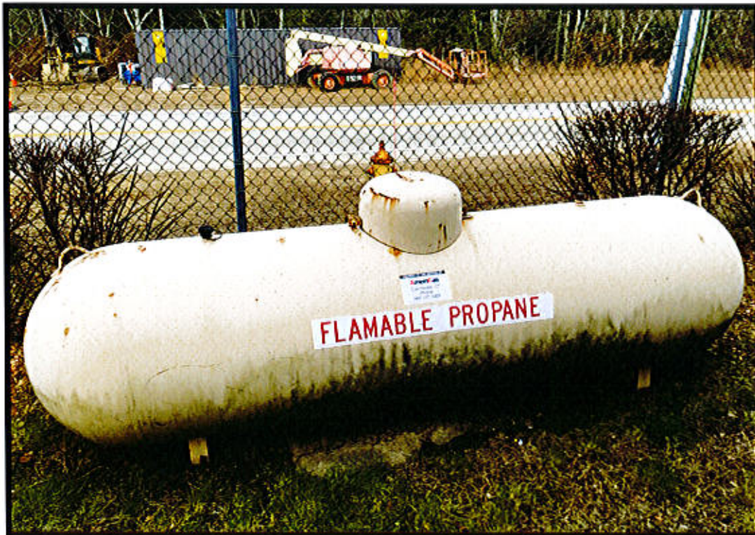
Photo 70. Mansfield Maintenance Facility – 100 N. Frontage Road, Mansfield, CT. Propane Tank.
