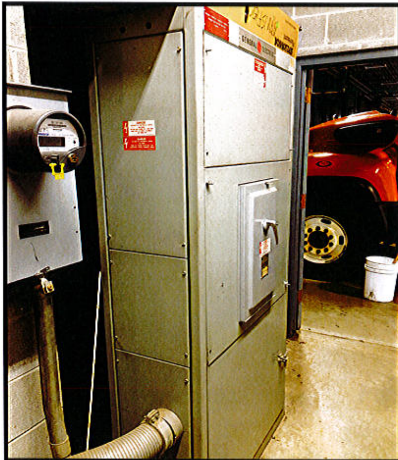
Photo 66. Mansfield Maintenance Facility – 100 N. Frontage Road, Mansfield, CT. Transfer switch Q.
