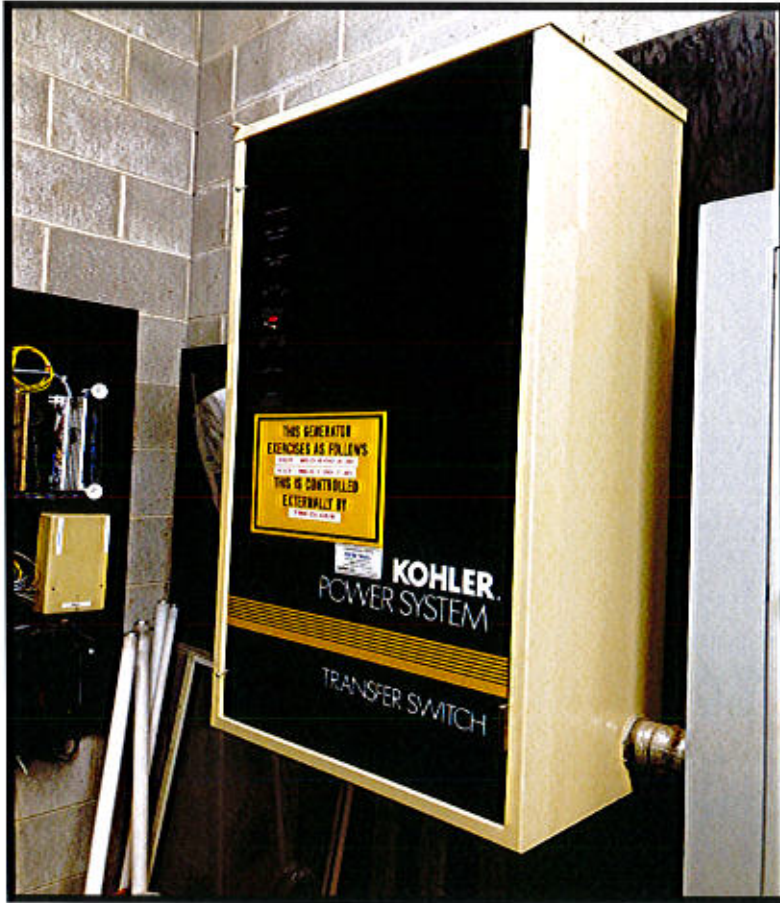
Photo 61. Mansfield Maintenance Facility – 100 N. Frontage Road, Mansfield, CT. Generator Transfer Switch.
