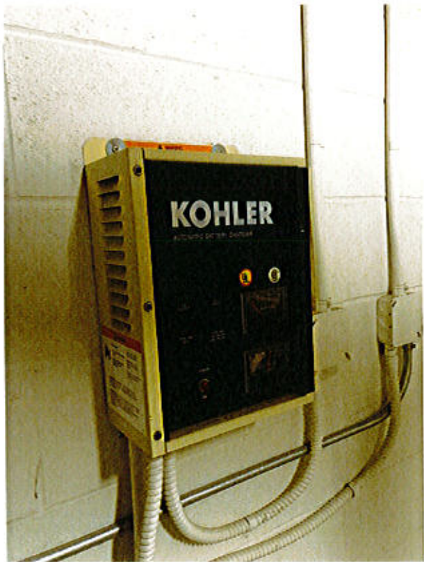
Generator battery charger
