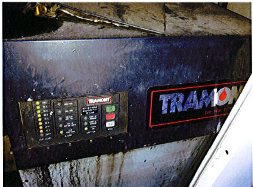
Inside generator control
