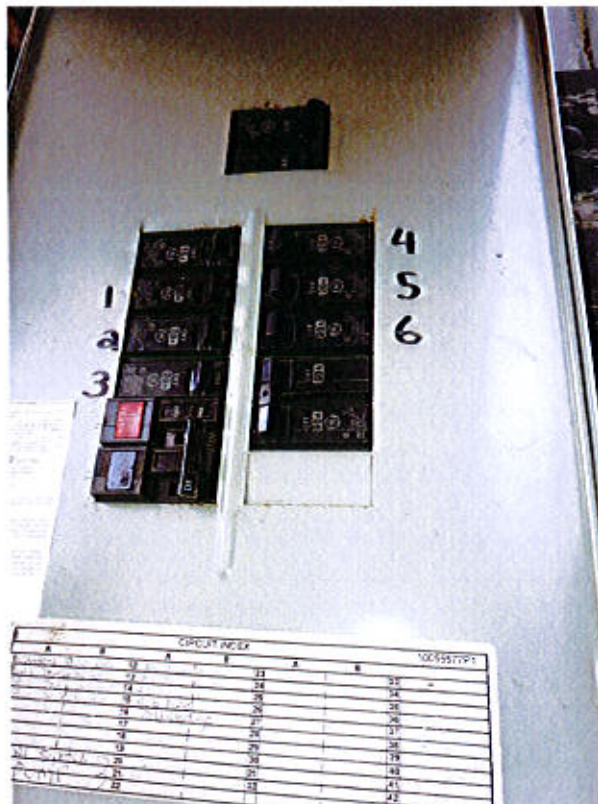
Generator electrical panel
