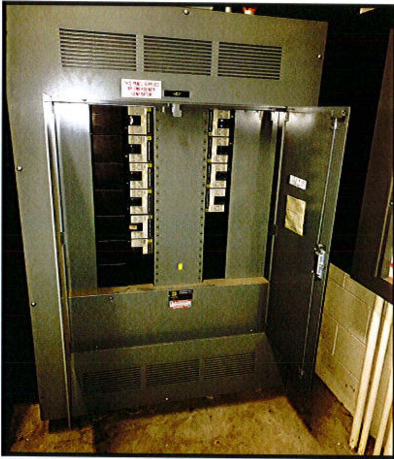
Photo 47. Hartford Bridge & Electrical Maintenance Facility – 49 Jennings Road, Hartford, CT Generator Panel.
