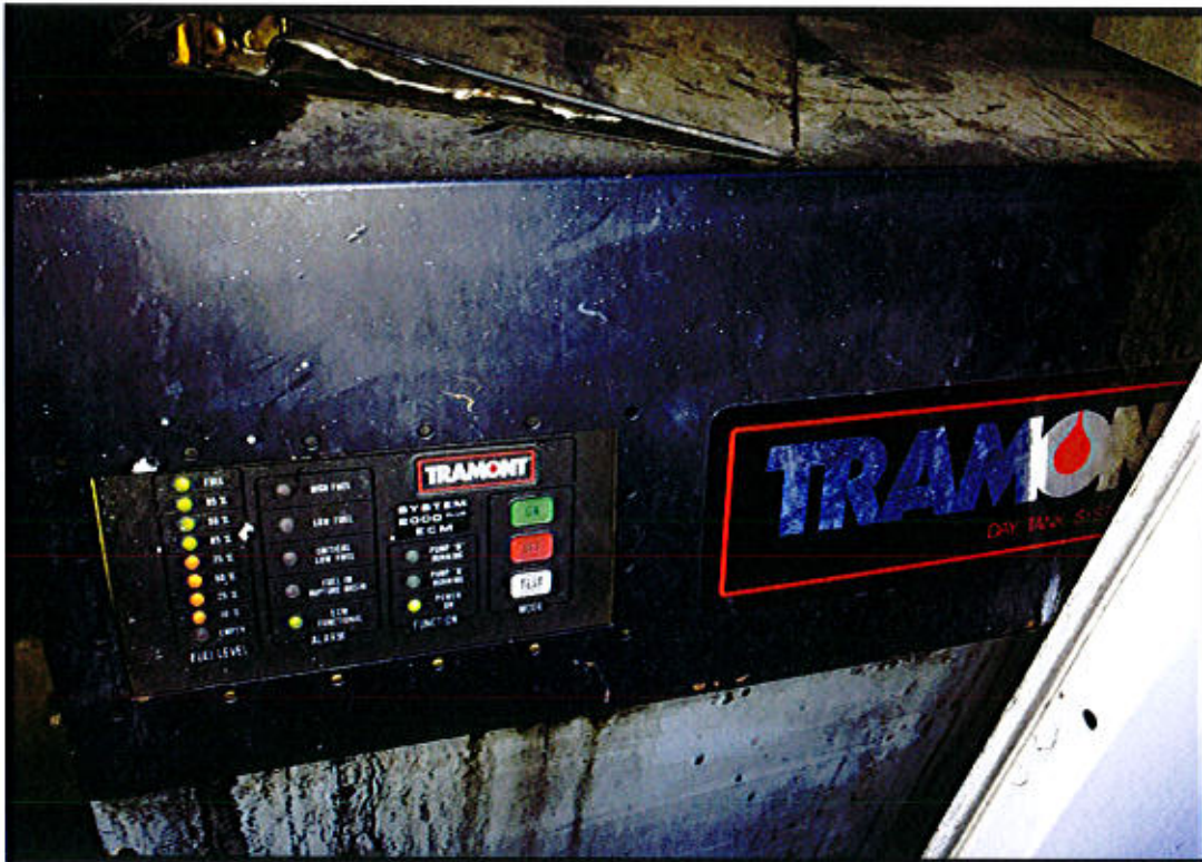
Photo 77. Mansfield Maintenance Facility – 100 N. Frontage Road, Mansfield, CT. Inside Generator Control.
