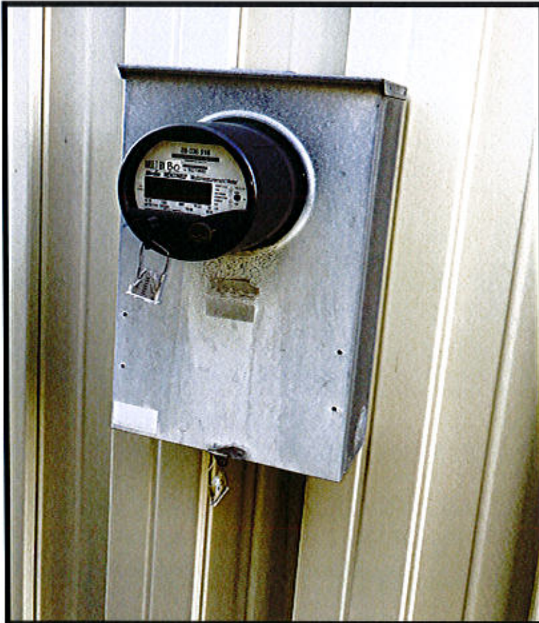
Photo 58. Hartford Bridge & Electrical Maintenance Facility – 49 Jennings Road, Hartford, CT Electrical Meter.
