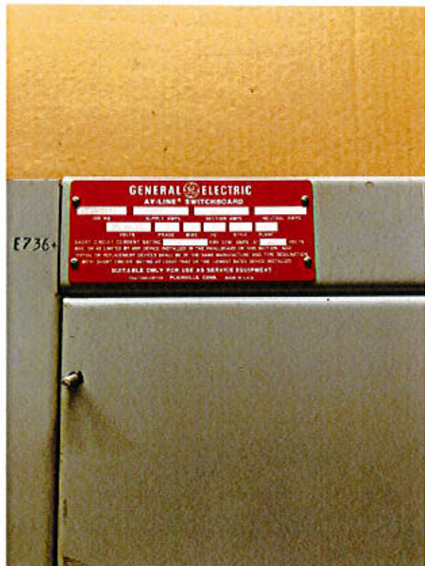
Electrical panel label
