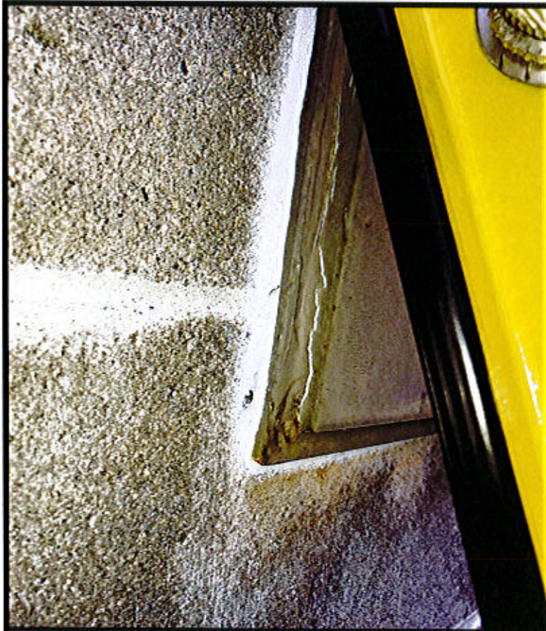
Photo 34. East Windsor Maintenance Facility – Prospect Hill Road, East Windsor, CT. Generator Exhaust Caulk.
