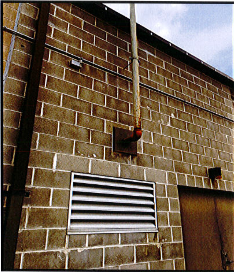
Photo 33. East Windsor Maintenance Facility – Prospect Hill Road, East Windsor, CT. Generator Room Vent and Generator Exhaust.
