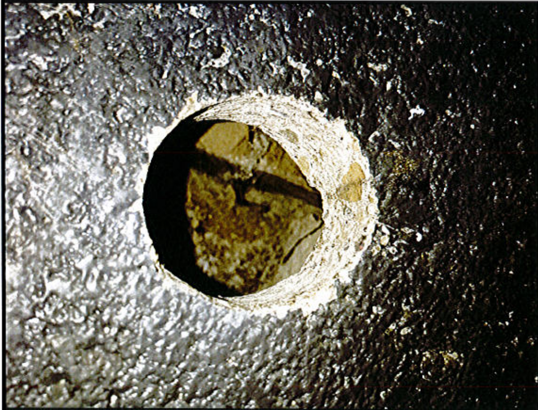
Photo 14. East Lyme Property & Facilities Region 2 Facility – Rt. 156, East Lyme, CT. Wall Penetration.
