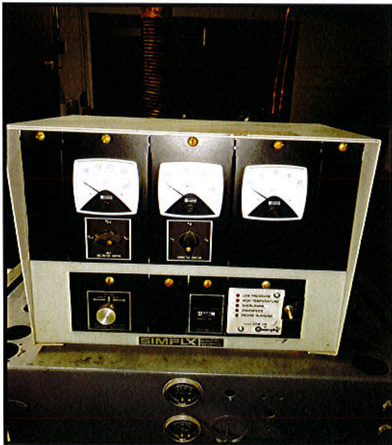
Photo 4. East Haven Repair Facility – 2100 N. High Street, East Haven, CT. Generator Control.
