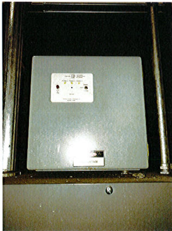
Generator room panel
