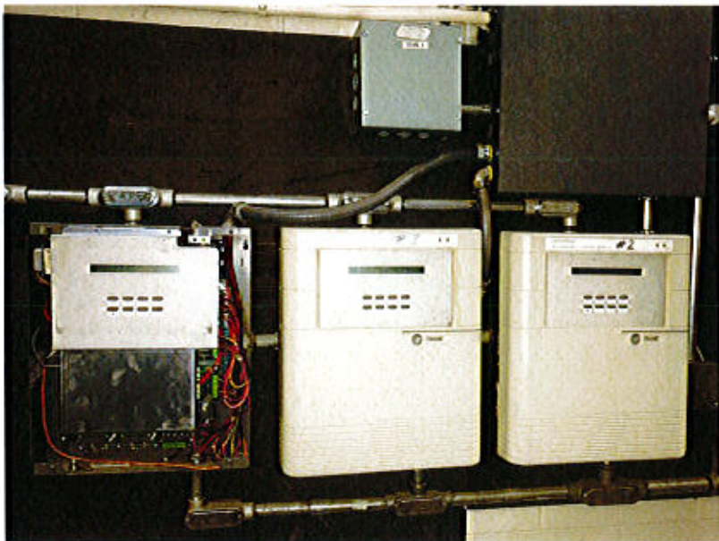
Trane Control boxes
