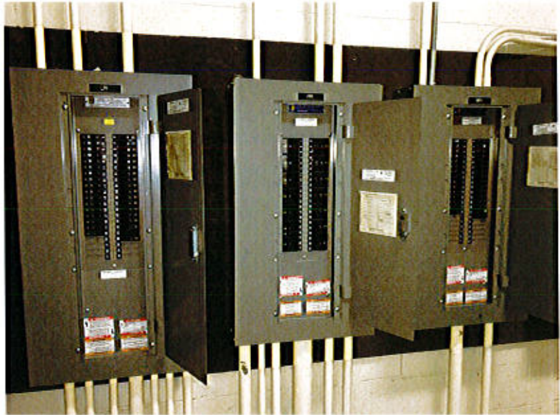
Generator room electrical panel
