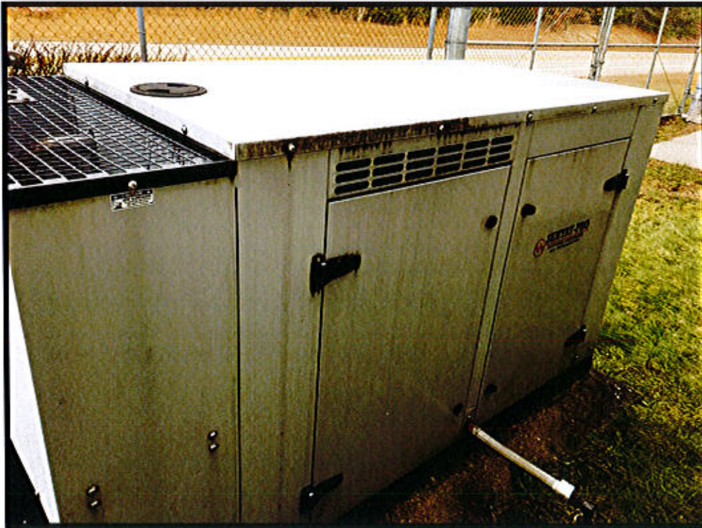
Photo 71. Mansfield Maintenance Facility – 100 N. Frontage Road, Mansfield, CT. Generator.
