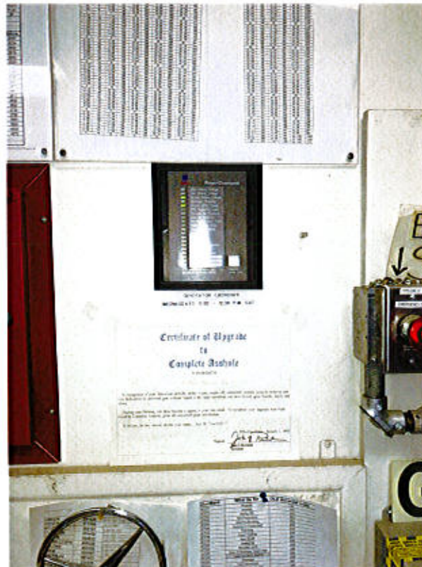
Tank monitoring system
