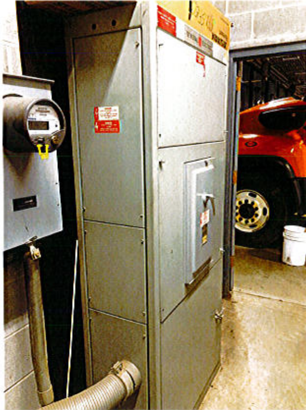
Transfer switch q
