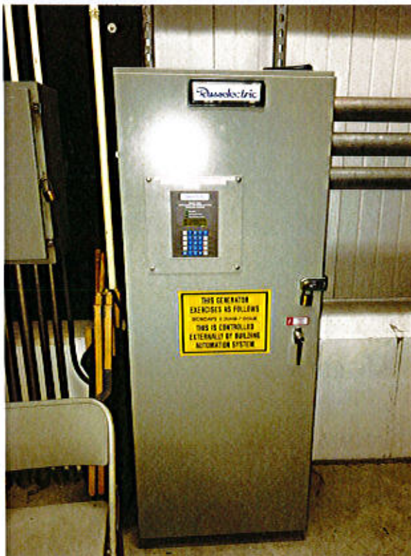
Generator Control box
