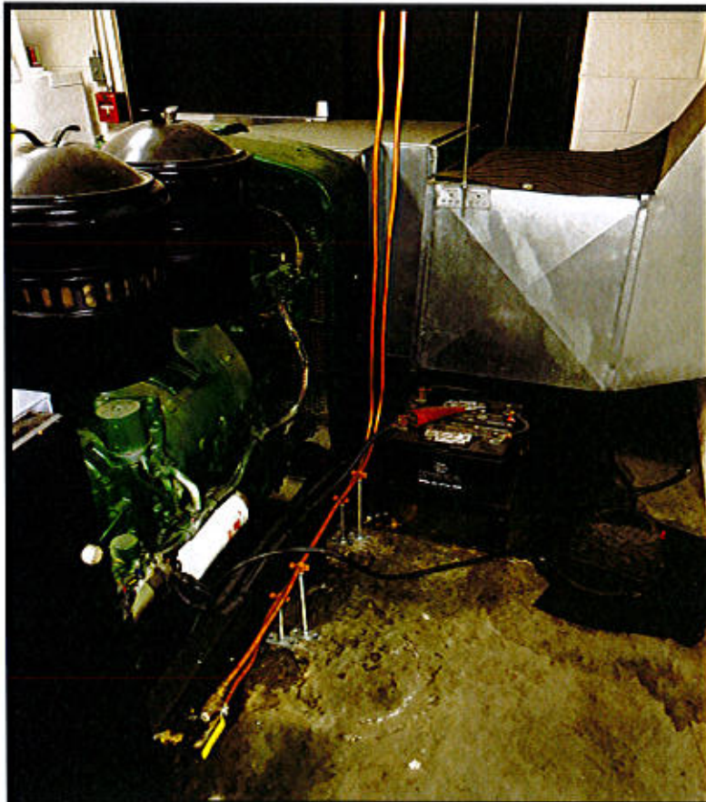
Photo 6. East Haven Repair Facility – 2100 N. High Street, East Haven, CT. Generator.
