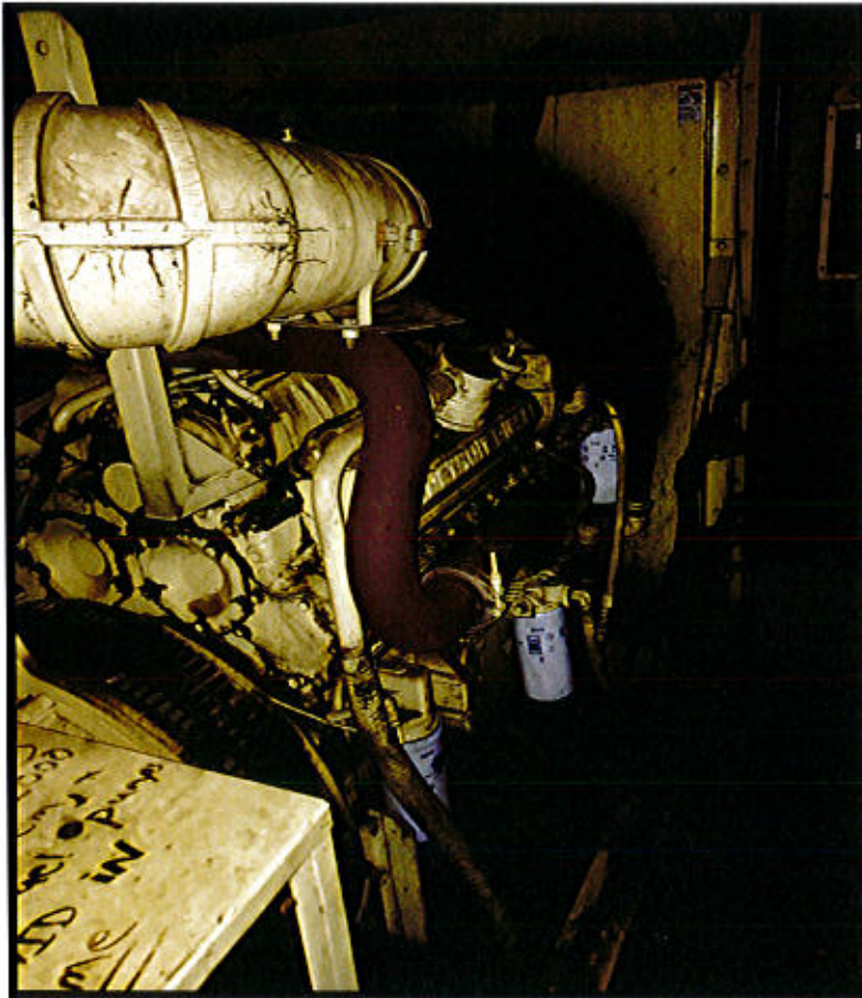
Photo 75. Mansfield Maintenance Facility – 100 N. Frontage Road, Mansfield, CT. Inside Generator.
