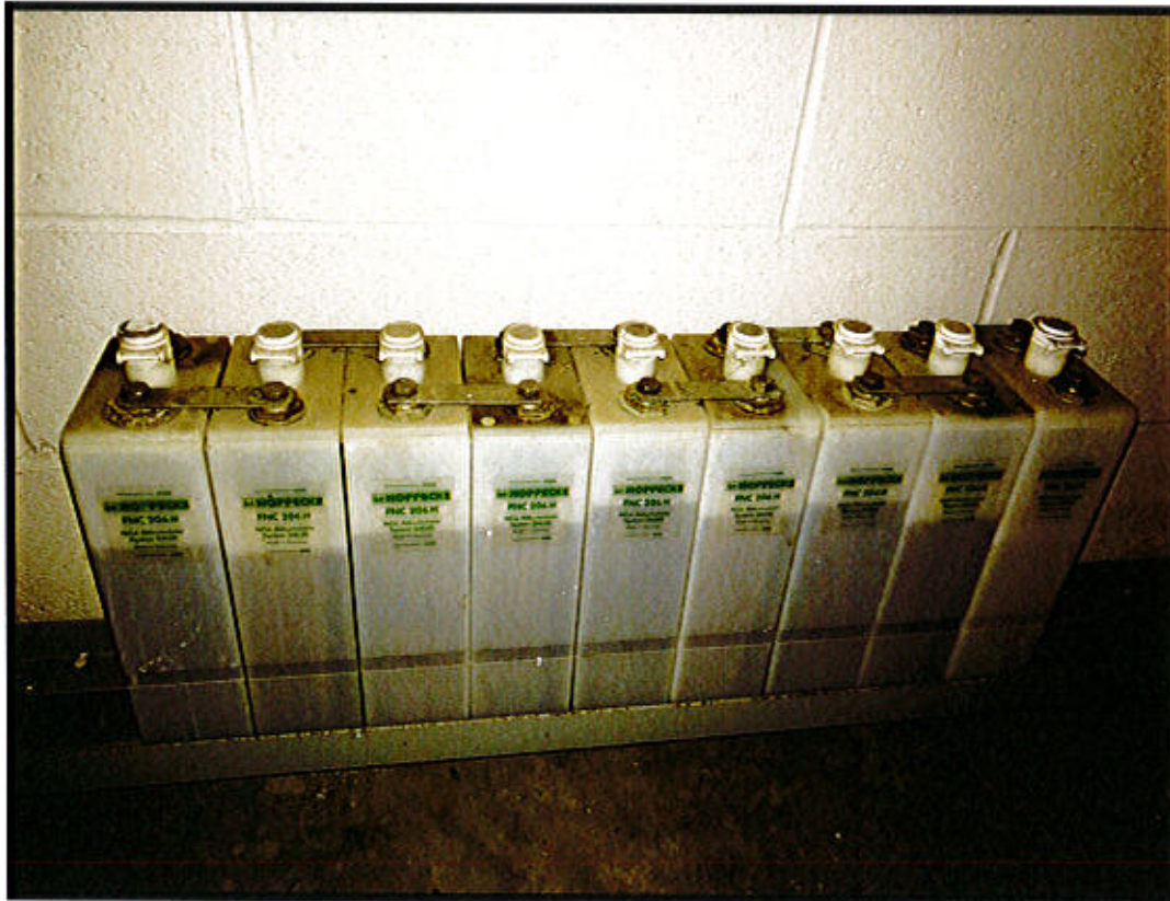
Photo 44. Haddam Maintenance Facility – Saybrook Road, Haddam, CT. Batteries.
