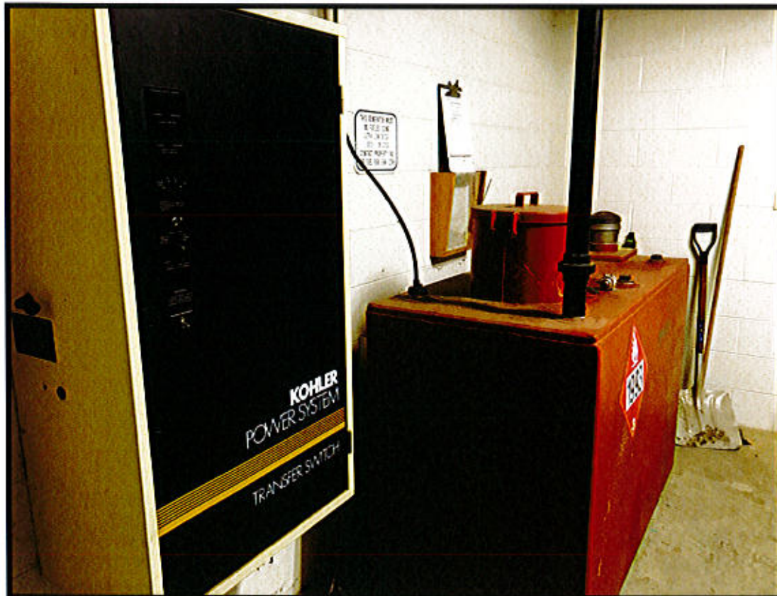
Photo 40. Haddam Maintenance Facility – Saybrook Road, Haddam, CT. Generator Transfer and Fuel Tank.
