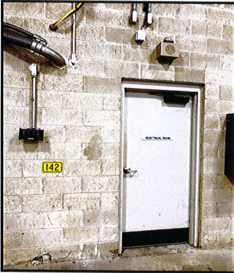
Photo 79. Rocky Hill Central Warehouse Facility – 600 Broad Street, Rocky Hill, CT. Electrical Room.
