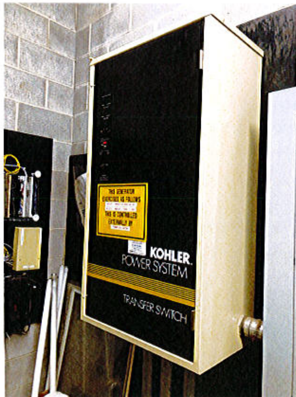
Generator transfer switch
