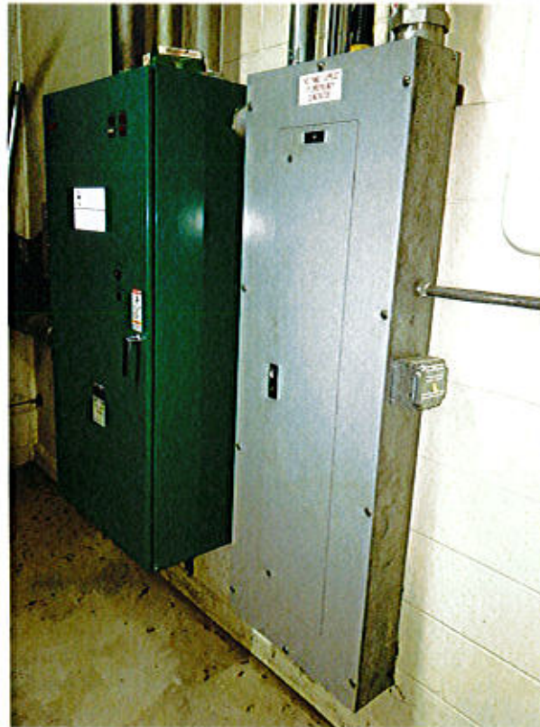
Generator & electrical box
