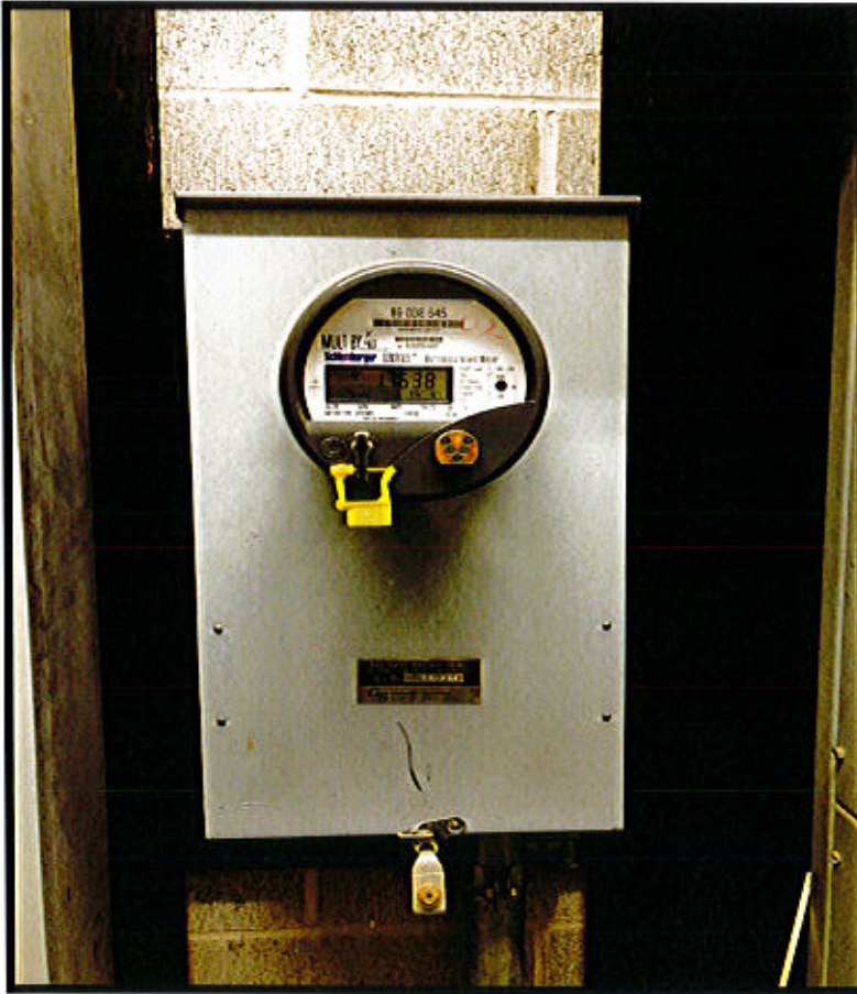
Photo 63. Mansfield Maintenance Facility – 100 N. Frontage Road, Mansfield, CT. Electrical Meter.
