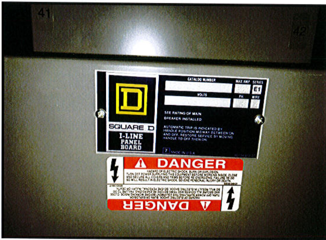
Photo 48. Hartford Bridge & Electrical Maintenance Facility – 49 Jennings Road, Hartford, CT Generator Panel Label.
