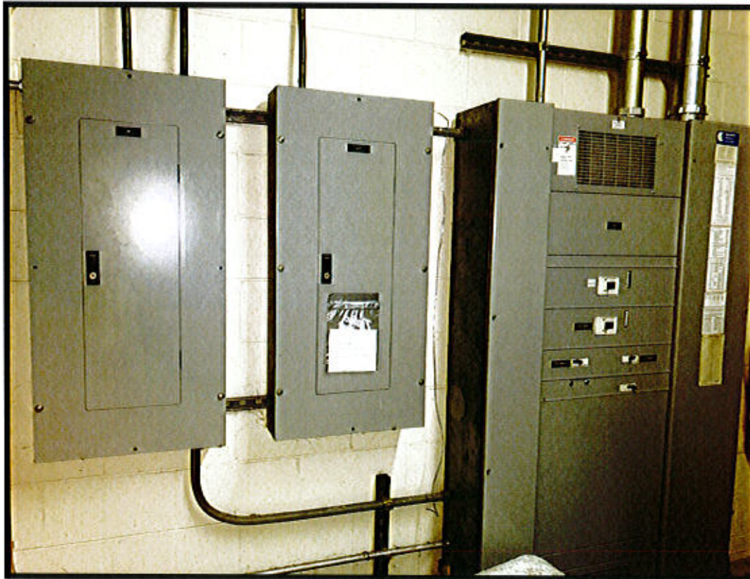
Photo 32. East Windsor Maintenance Facility – Prospect Hill Road, East Windsor, CT. Electrical Panels
