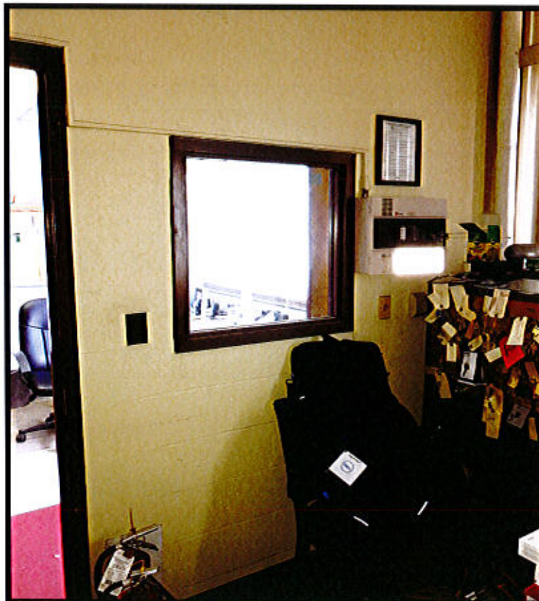
Photo 20. East Lyme Property & Facilities Region 2 Facility – Rt. 156, East Lyme, CT. Possible Annunciator Location.
