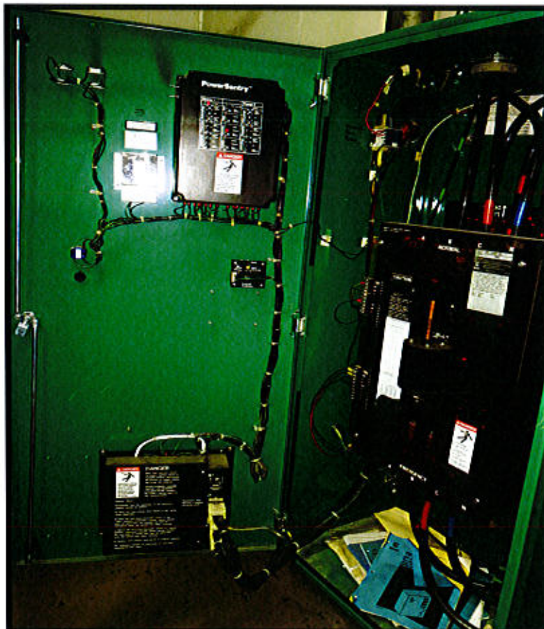
Photo 28. East Lyme Property & Facilities Region 2 Facility – Rt. 156, East Lyme, CT. Inside Generator Control.
