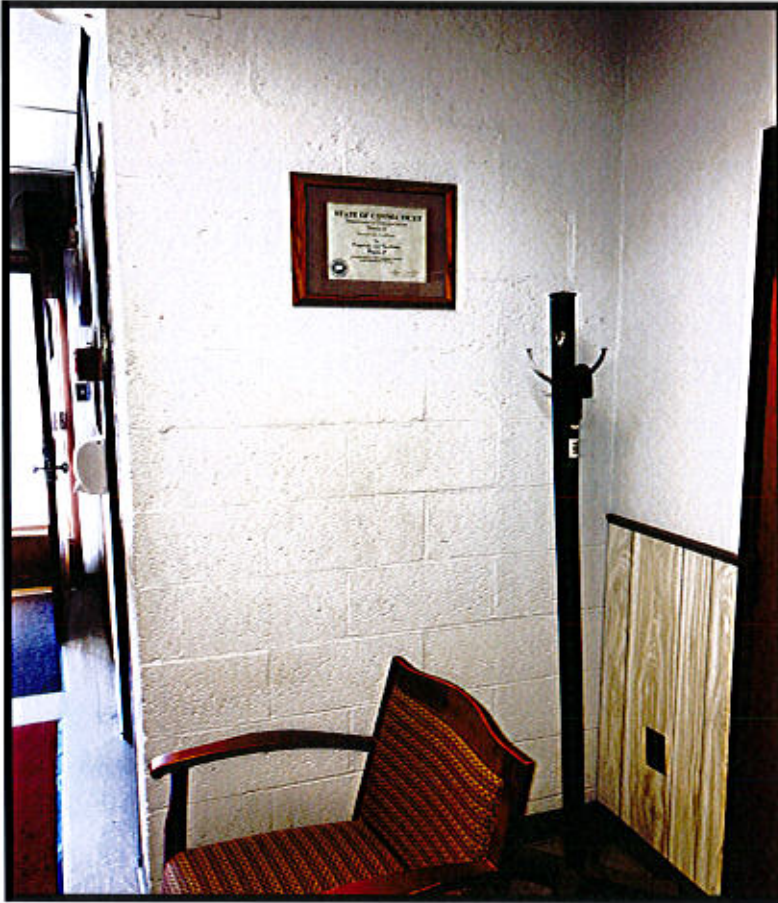
Photo 23. East Lyme Property & Facilities Region 2 Facility – Rt. 156, East Lyme, CT. Possible Annunciator Location.
