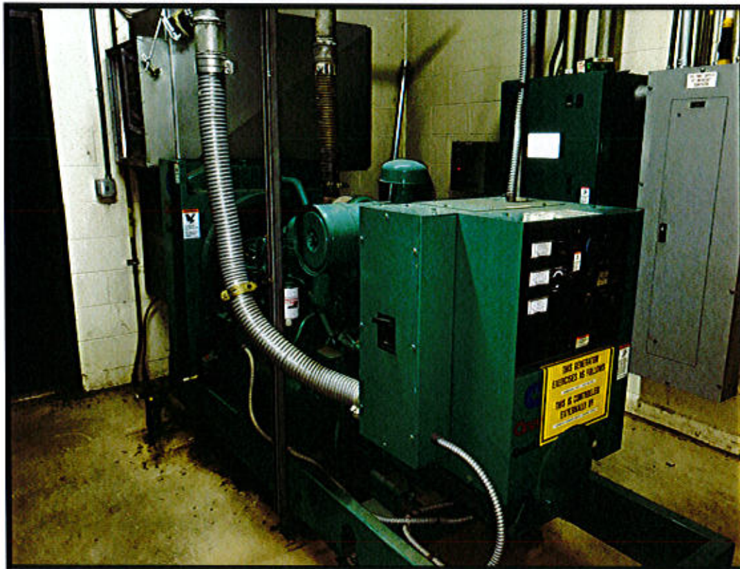
Photo 24. East Windsor Maintenance Facility – Prospect Hill Road, East Windsor, CT. Generator.
