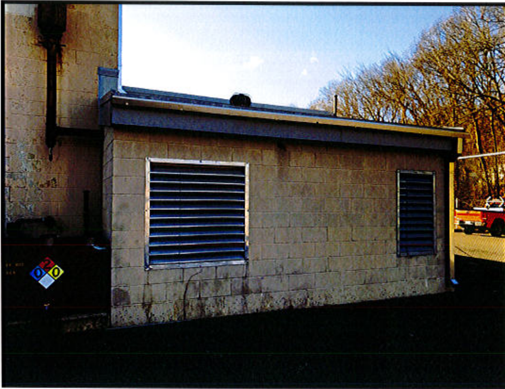
Photo 7. East Haven Repair Facility – 2100 N. High Street, East Haven, CT. Generator Vents.
