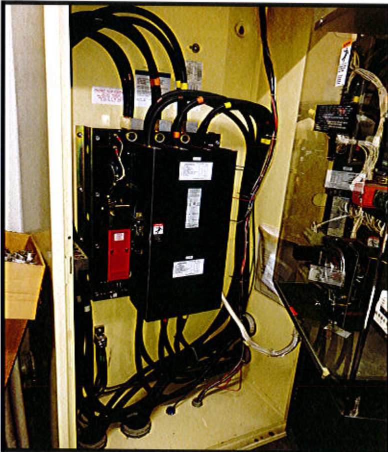
Photo 80. Rocky Hill Central Warehouse Facility – 600 Broad Street, Rocky Hill, CT. Generator Transfer.
