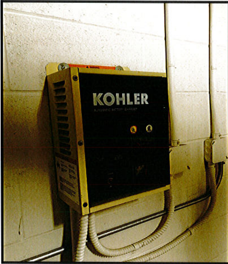
Photo 43. Haddam Maintenance Facility – Saybrook Road, Haddam, CT. Generator Battery Charger.
