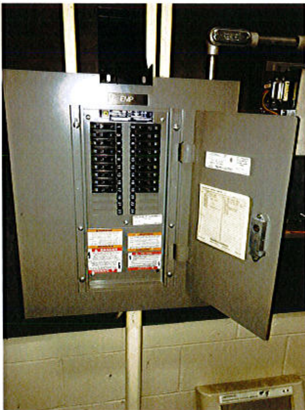
Generator room electrical panel
