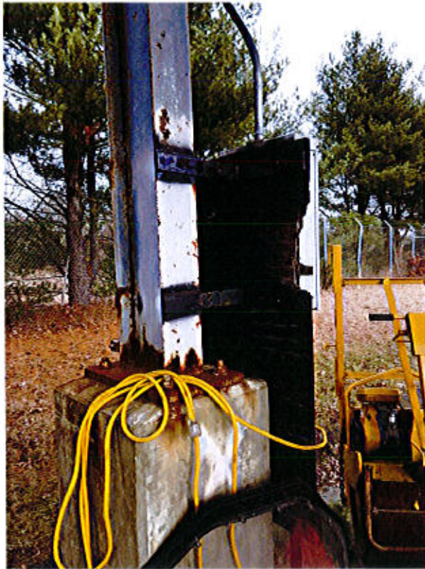
Generator electrical panel
