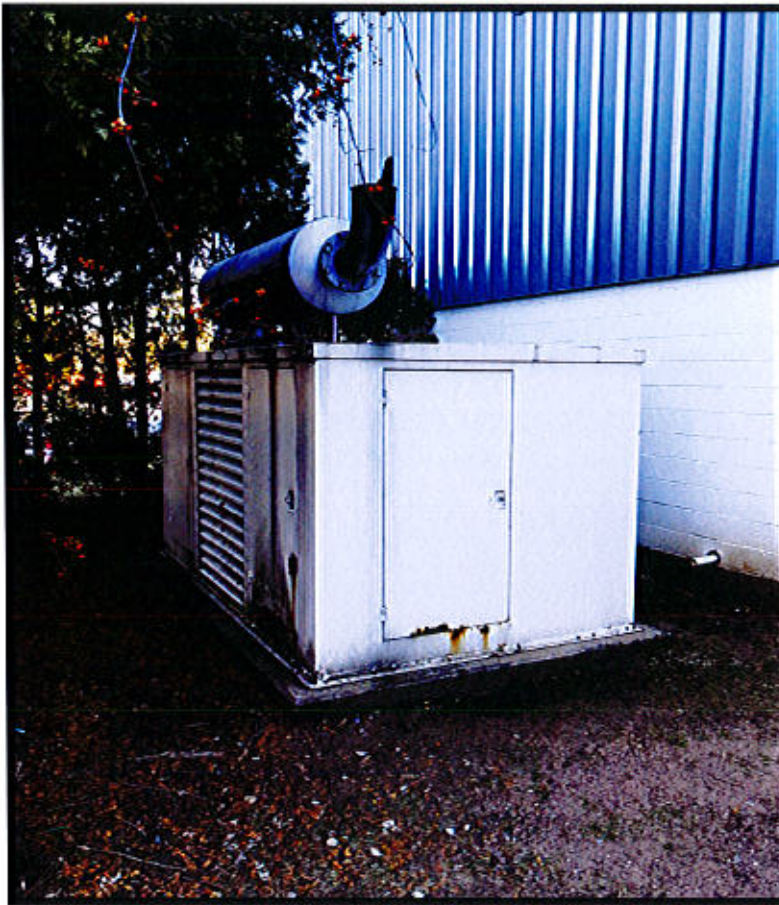
Photo 73. Mansfield Maintenance Facility – 100 N. Frontage Road, Mansfield, CT. Generator.
