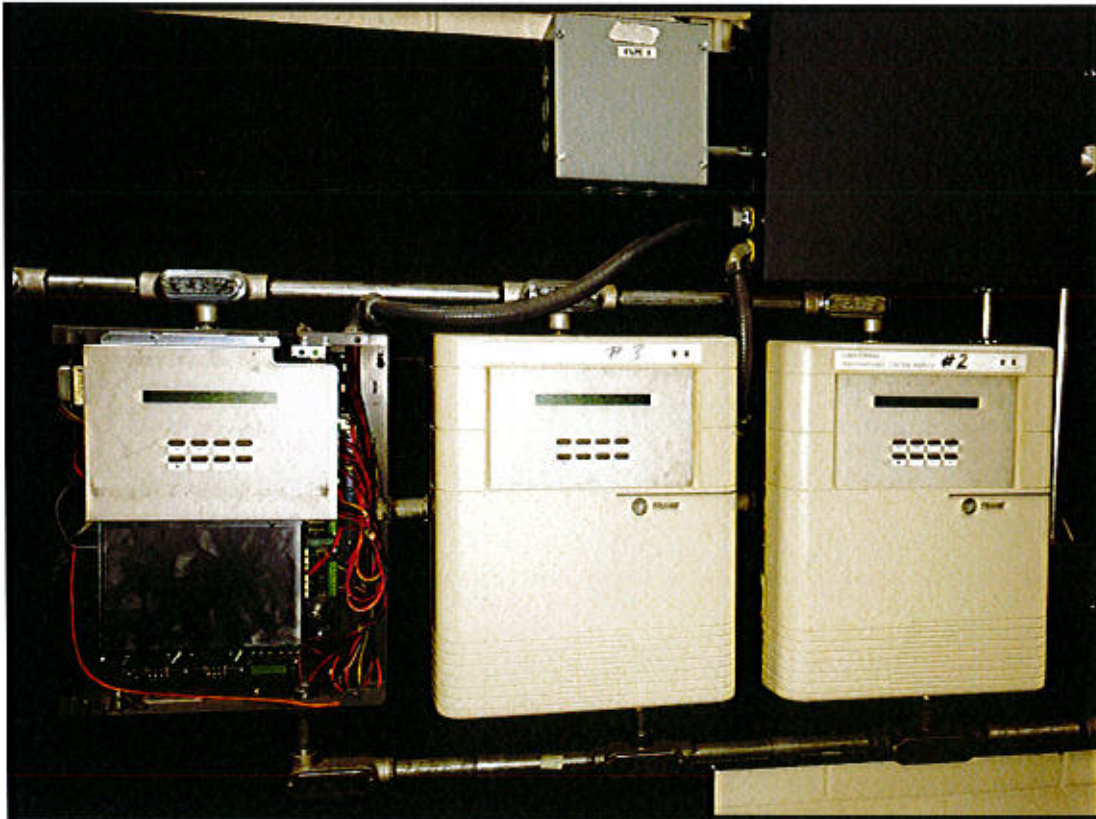
Photo 52. Hartford Bridge & Electrical Maintenance Facility – 49 Jennings Road, Hartford, CT Trane Control Boxes.
