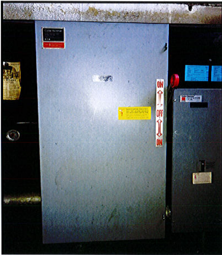
Photo 13. East Lyme Property & Facilities Region 2 Facility – Rt. 156, East Lyme, CT. Electrical Panel.
