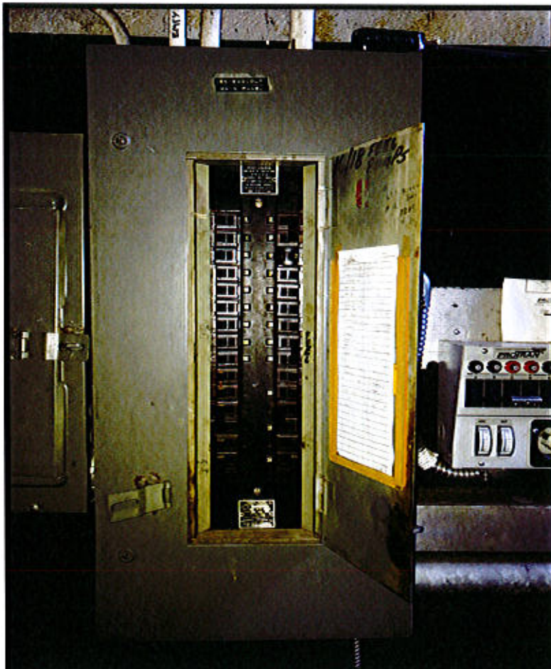
Photo 12. East Lyme Property & Facilities Region 2 Facility – Rt. 156, East Lyme, CT. Electrical Panel.
