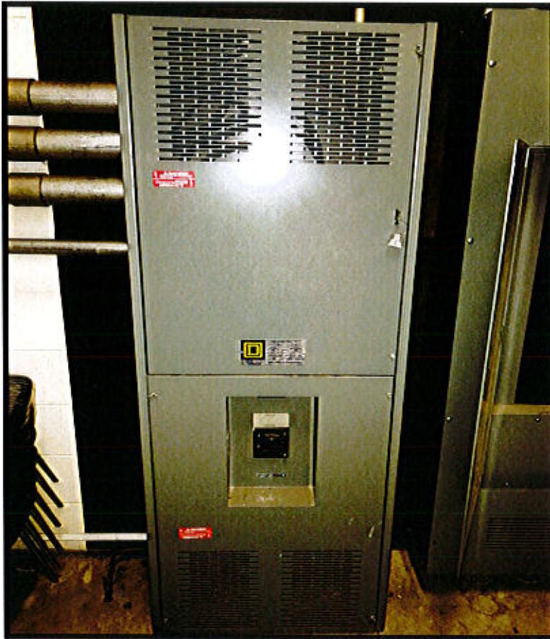
Photo 45. Hartford Bridge & Electrical Maintenance Facility – 49 Jennings Road, Hartford, CT Generator Room Panel.
