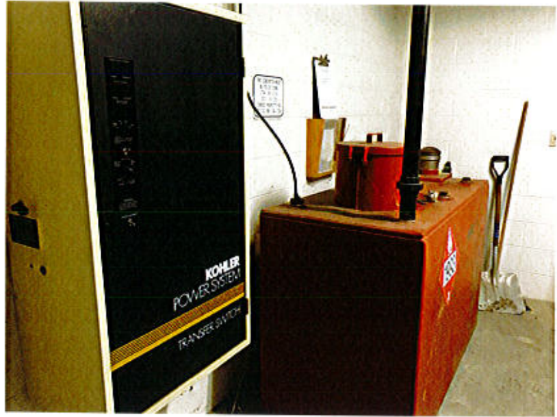
Generator transfer and fuel tank
