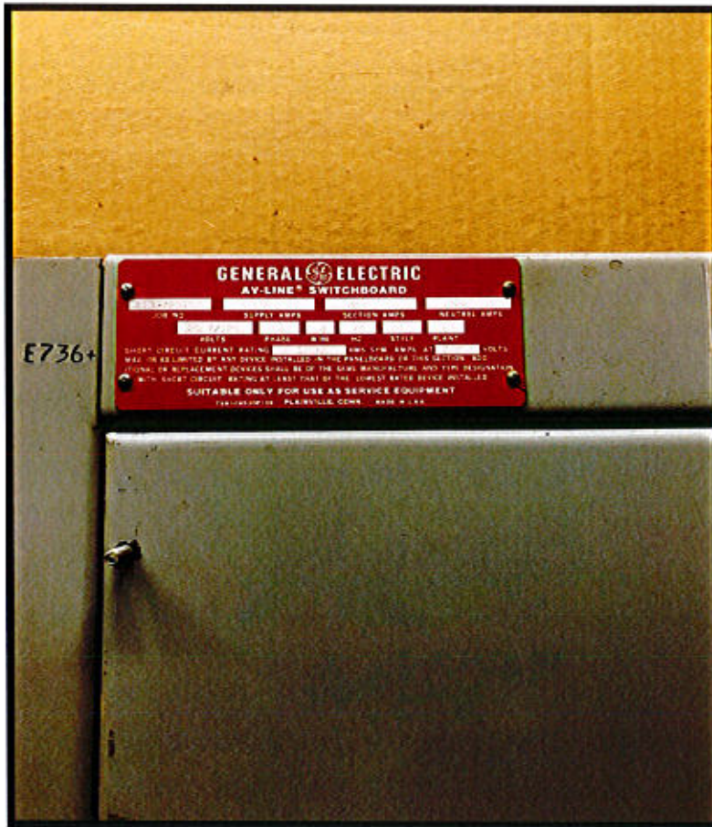
Photo 65. Mansfield Maintenance Facility – 100 N. Frontage Road, Mansfield, CT. Electrical Panel Label.
