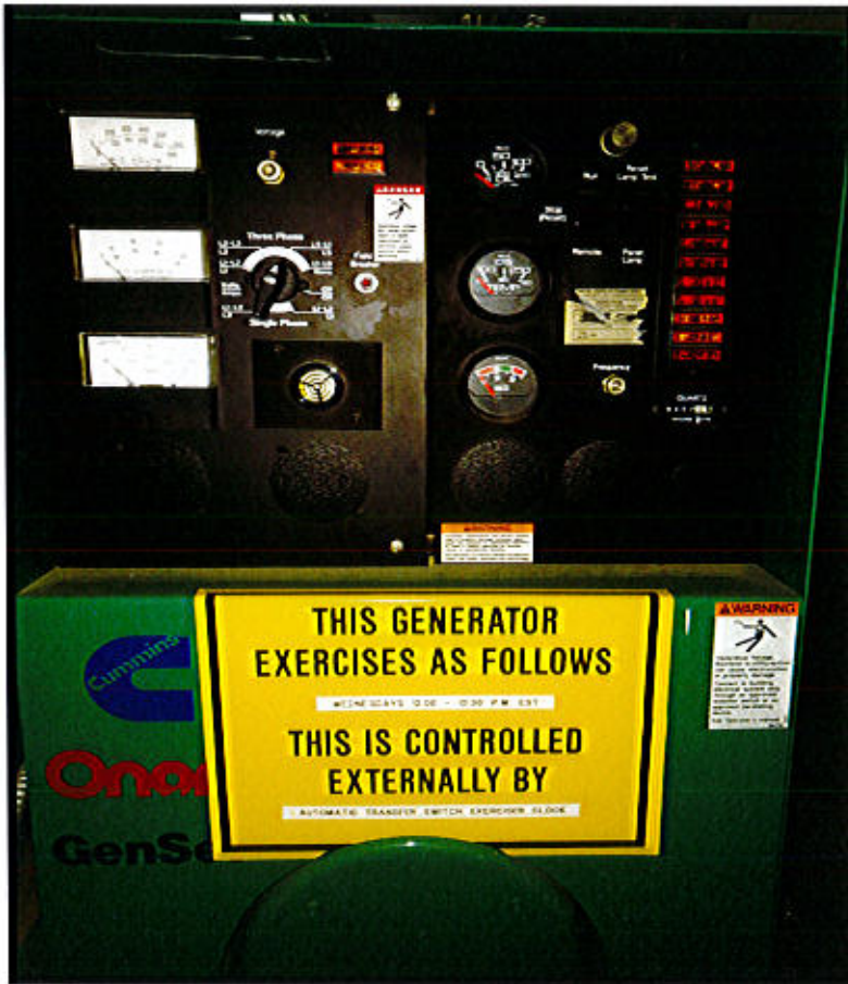
Photo 25. East Windsor Maintenance Facility – Prospect Hill Road, East Windsor, CT. Generator Control.
