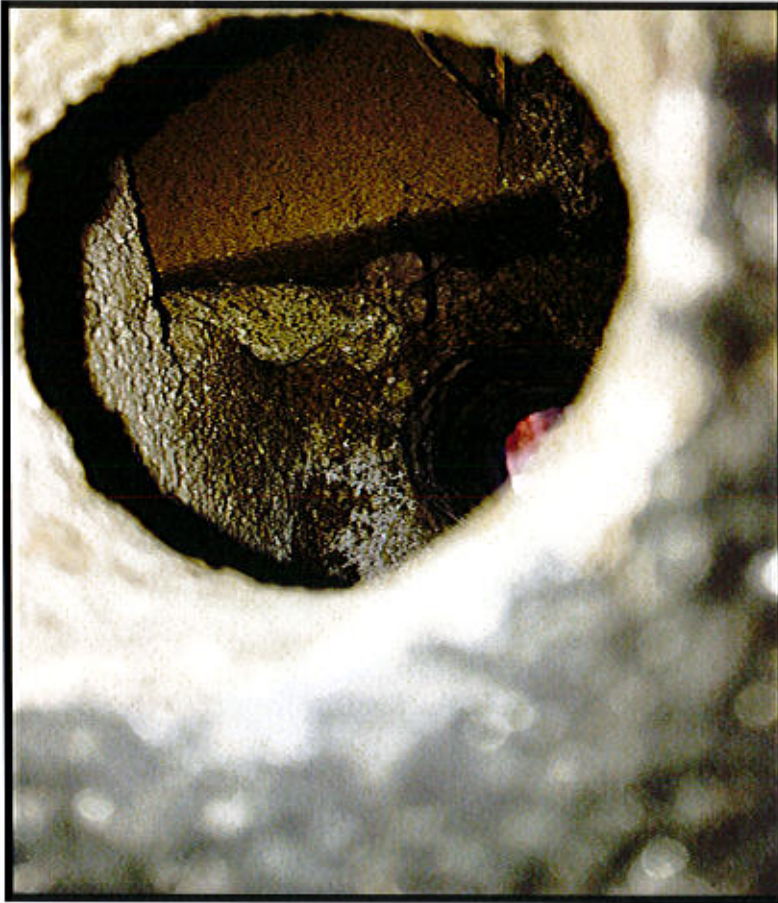
Photo 15. East Lyme Property & Facilities Region 2 Facility – Rt. 156, East Lyme, CT. Wall Penetration.
