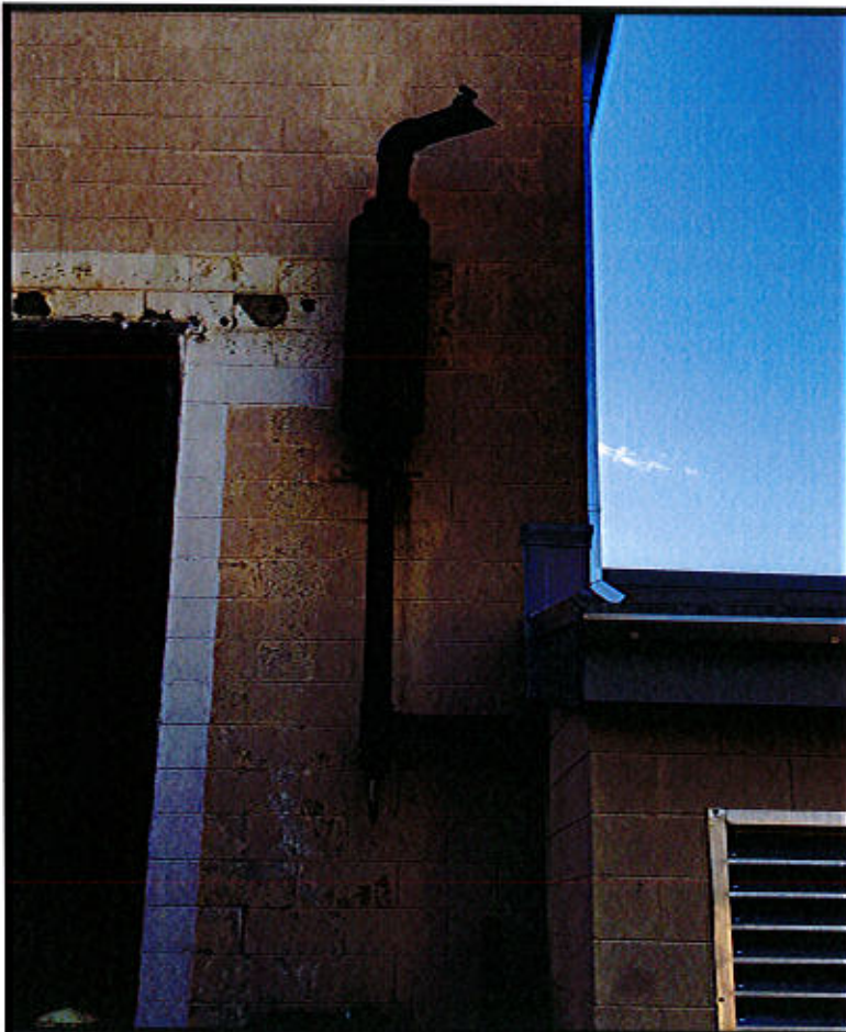
Photo 8. East Haven Repair Facility – 2100 N. High Street, East Haven, CT. Generator Exhaust.
