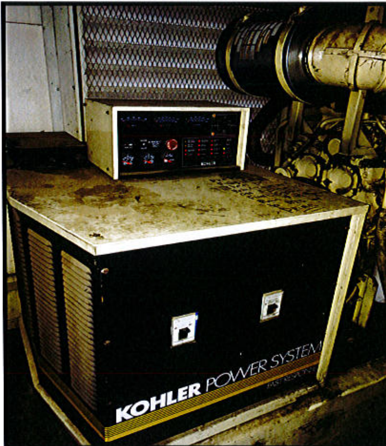
Photo 74. Mansfield Maintenance Facility – 100 N. Frontage Road, Mansfield, CT. Inside Generator.
