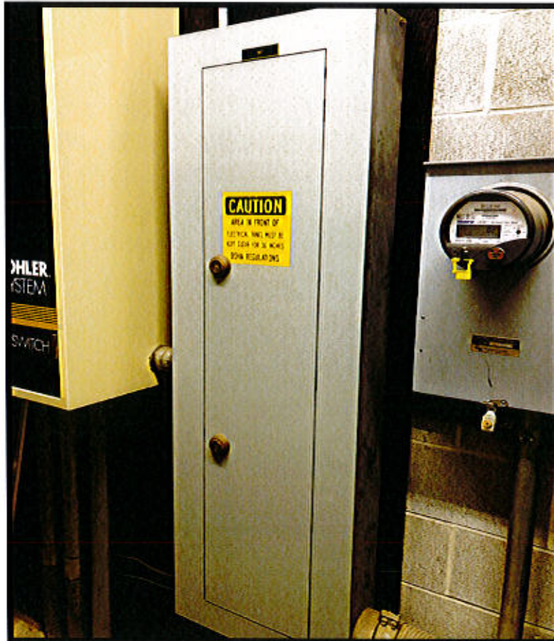
Photo 64. Mansfield Maintenance Facility – 100 N. Frontage Road, Mansfield, CT. Electrical Panel.
