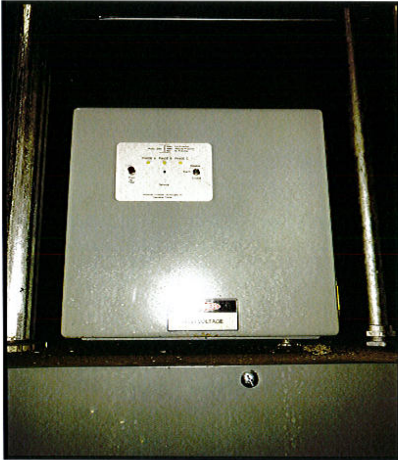
Photo 49. Hartford Bridge & Electrical Maintenance Facility – 49 Jennings Road, Hartford, CT Generator Room Panel.
