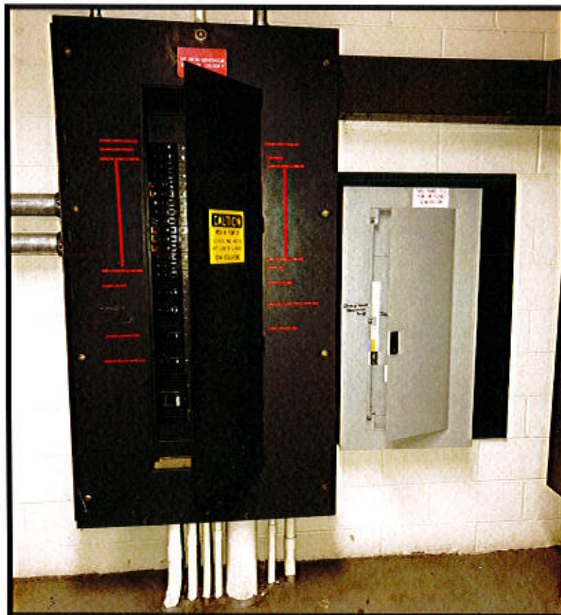
Photo 2. East Haven Repair Facility – 2100 N. High Street, East Haven, CT. Electrical Panels.
