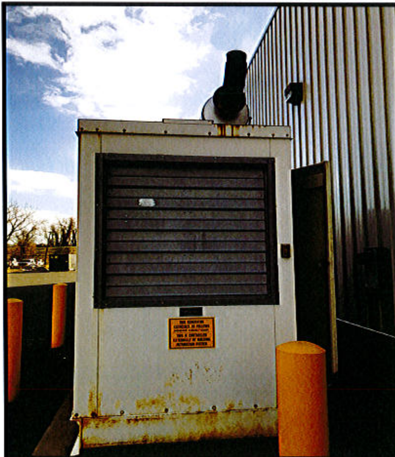
Photo 56. Hartford Bridge & Electrical Maintenance Facility – 49 Jennings Road, Hartford, CT Generator.
