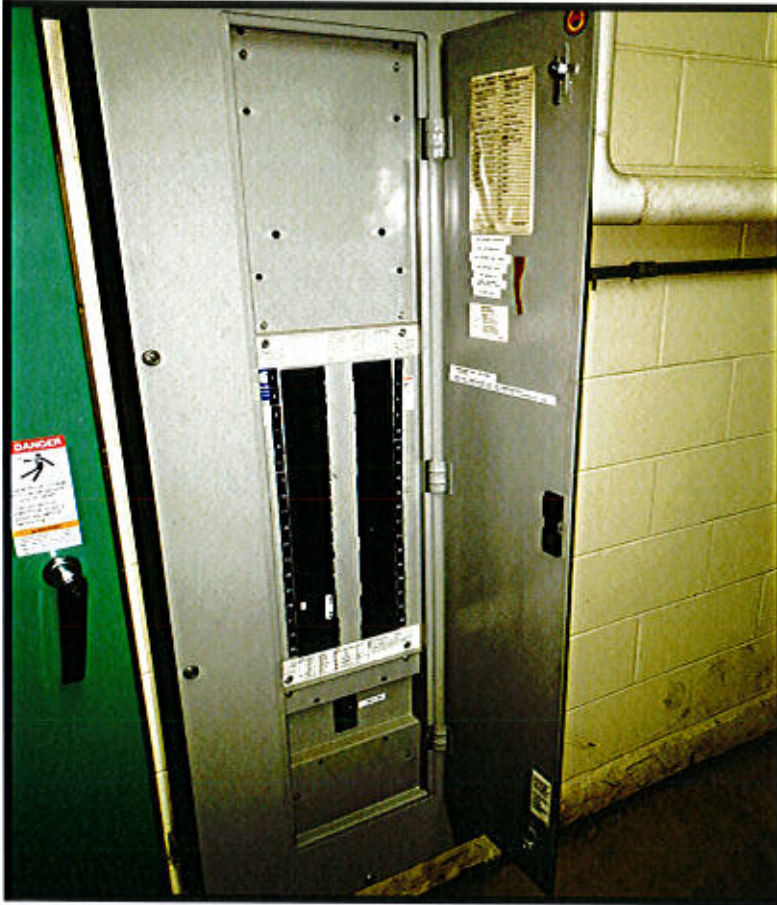
Photo 29. East Windsor Maintenance Facility – Prospect Hill Road, East Windsor, CT. Electrical Panel.
