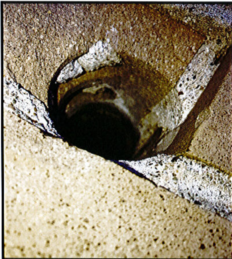
Photo 16. East Lyme Property & Facilities Region 2 Facility – Rt. 156, East Lyme, CT. Wall Penetration.
