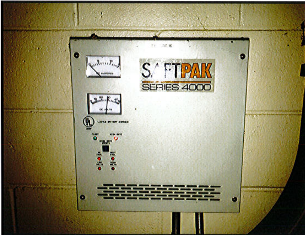
Photo 27. East Windsor Maintenance Facility – Prospect Hill Road, East Windsor, CT. Control Panel.
