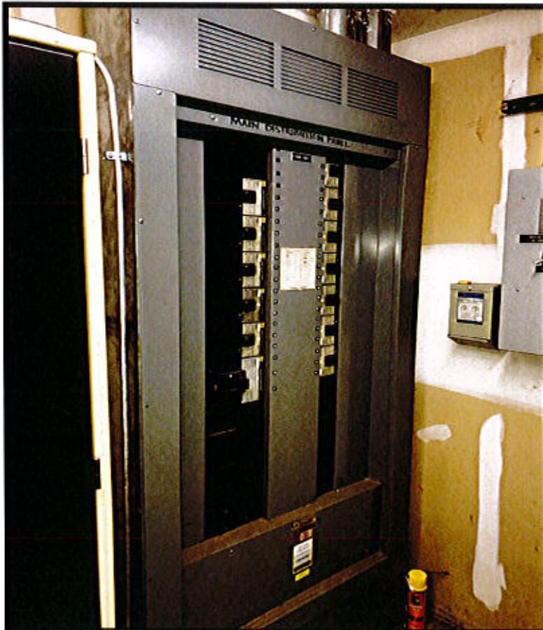
Photo 84. Rocky Hill Central Warehouse Facility – 600 Broad Street, Rocky Hill, CT. Electrical Panel.
