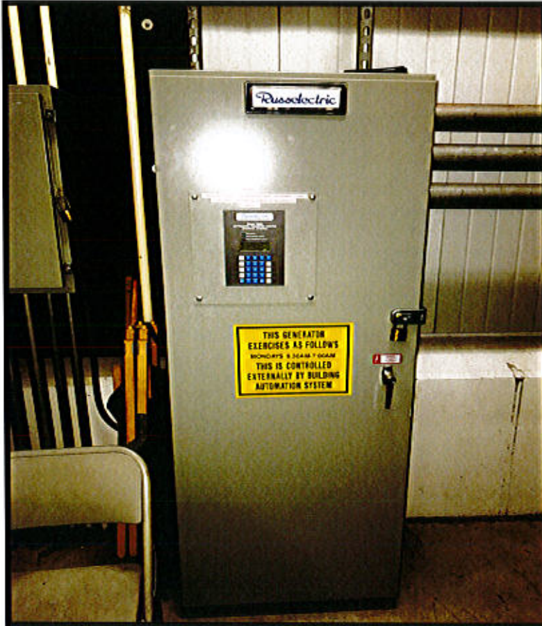
Photo 55. Hartford Bridge & Electrical Maintenance Facility – 49 Jennings Road, Hartford, CT Generator Control Box.
