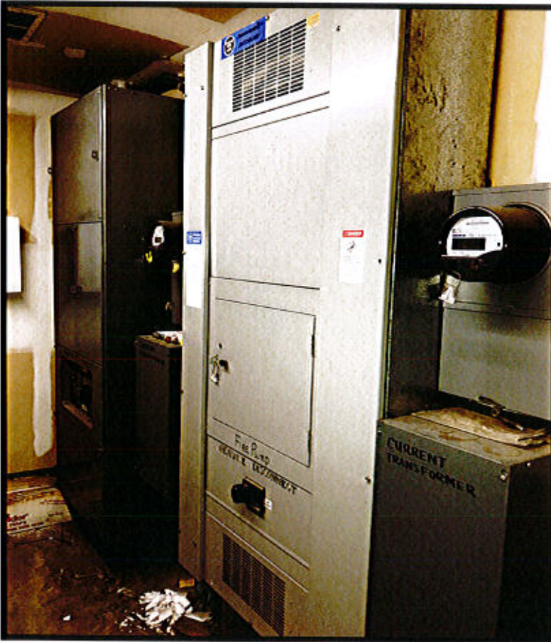
Photo 85. Rocky Hill Central Warehouse Facility – 600 Broad Street, Rocky Hill, CT. Electrical Panels.
