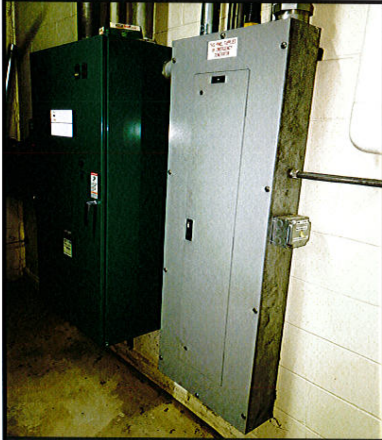
Photo 30. East Windsor Maintenance Facility – Prospect Hill Road, East Windsor, CT. Generator & Electrical Box.
