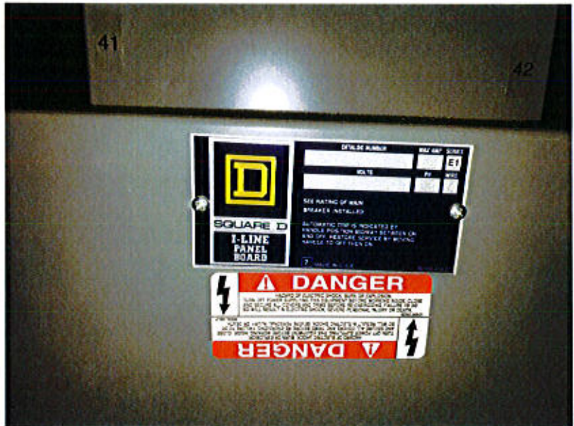
Generator panel label
