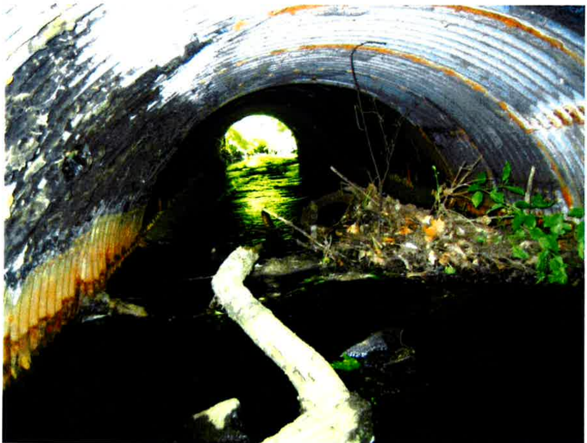
Image 3: Downstream view of culvert pipe. Note the loss of protective asphalt coating, corrosion and distortion of the metal pipe liner and debris.
