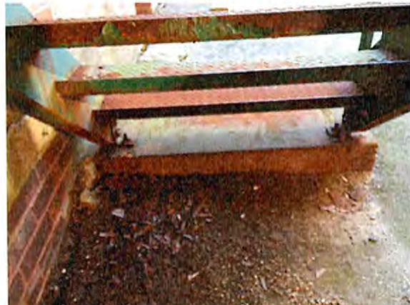
Figure 4: Deteriorated Steel Flakes Below Stair
