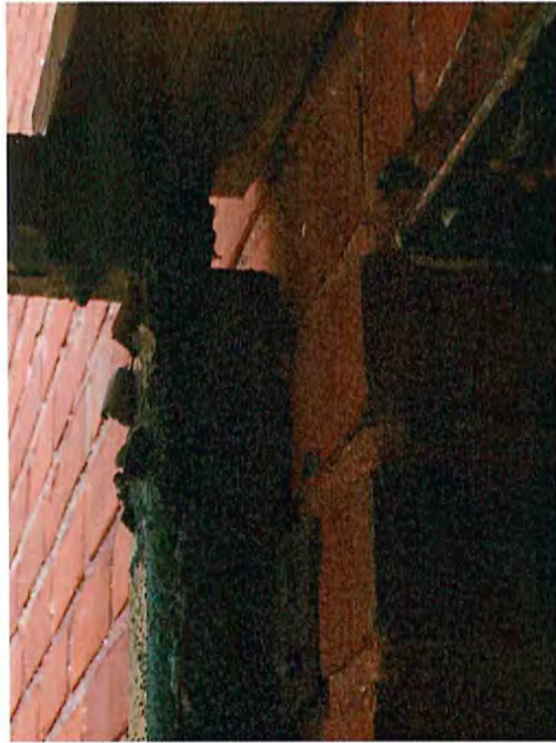
Figure 6: Roof Column Not Aligning
