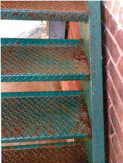
Figure 2: Rust Expansion Damage
