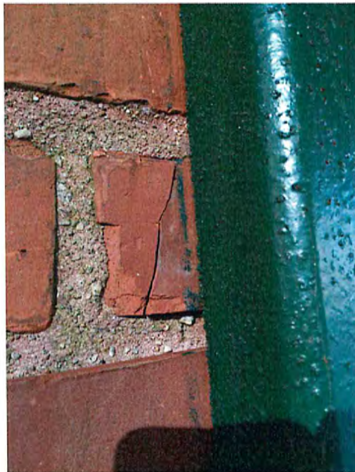
Figure 7: Brick Damaged by Roof Clip
