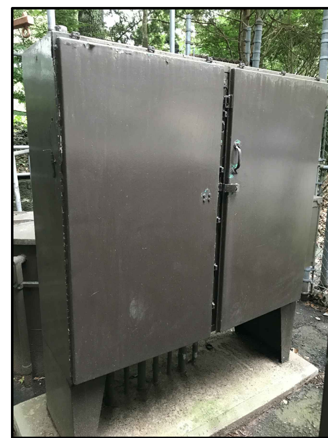
PHOTOGRAPH ELECTRICAL DISTRIBUTION CONTROL PANEL #3
