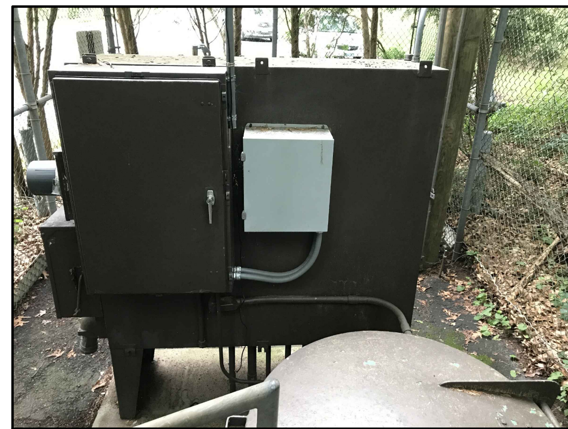
PHOTOGRAPH INSTRUMENTATION CONTROL PANEL #2
