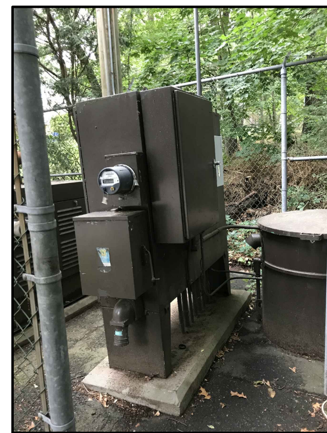
PHOTOGRAPH STANCHION MOUNTED EQUIPMENT #1
