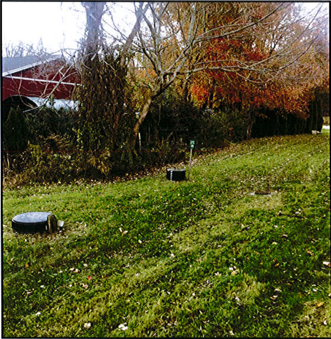
PHOTO 5. D-side Septic Tank & Monitoring Wells.
