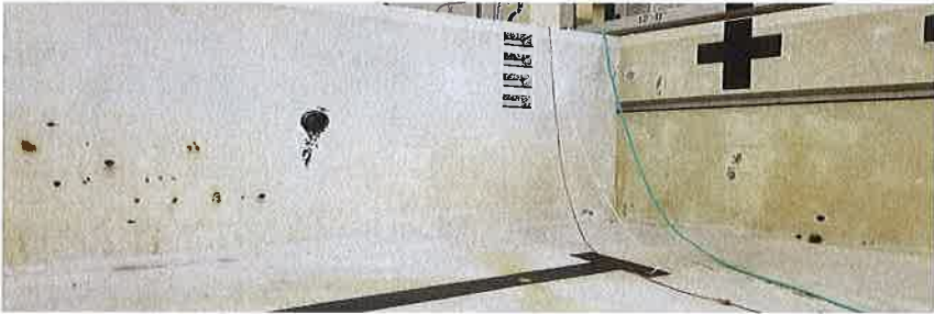
Examples of Pool Staining, likely caused from wire ties or wire mesh with improper coverage
