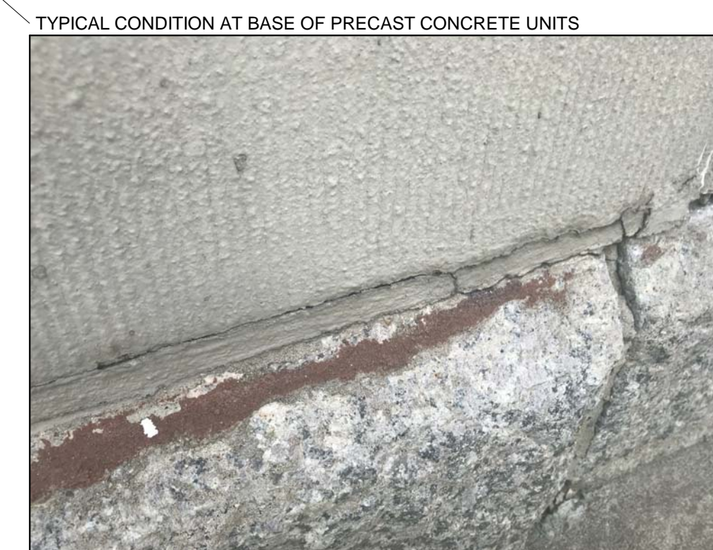
TYPICAL CONDITION AT BASE OF PRECAST CONCRETE UNITS
