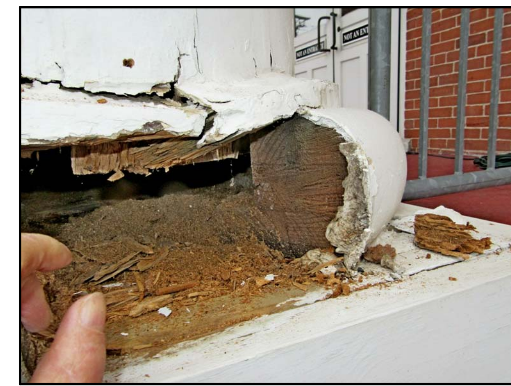
CLOSE UP OF AREA OF REMOVED BULLNOSE BASE SEGMENT. NOTE ROTTED COVE BASE TRIM ABOVE BULLNOSE SEGMENTS. PHOTO C04
