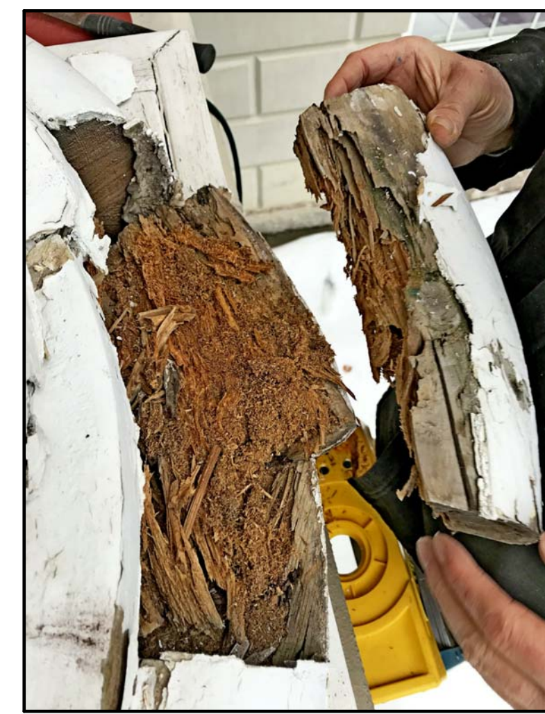
1/8 SEGMENT OF ROTTED BULLNOSE 2 PART BASE. ROTTED AND EASILY REMOVED BY HAND PHOTO C03
