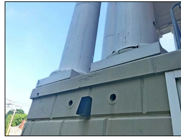
TYPICAL CONDITION AT BASE OF WOOD COLUMNS AND TOP OF CONCRETE
