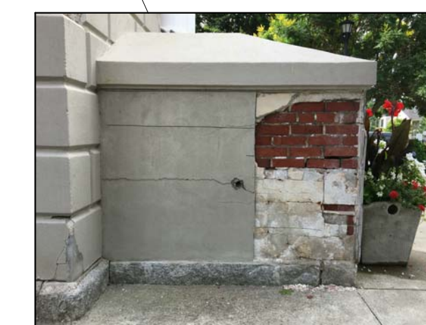
REMOVAL TEST PATCH OF DELAMINATED STUCCO. ALL EXISTING STUCCO TO BE REMOVED, BRICK TO BE REPOINTED, AND NEW STUCCO TO BE INSTALLED AND TOOLED TO MATCH RUSTICATION PATTERN.
