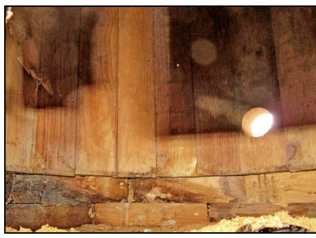
INTERIOR OF COLUMN BASE WITH VERTICAL STAVES AND 2 PART BULLNOSE BASE. NOTE VENTILATION HOLE IN SHAFT PHOTO C01
