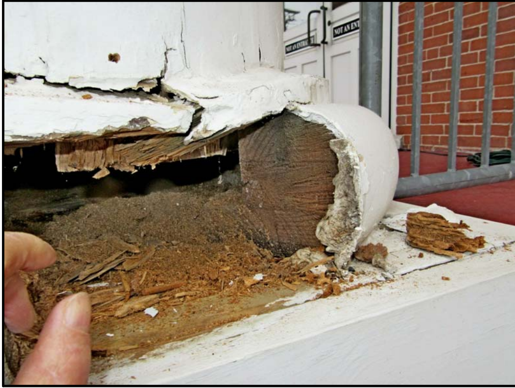
CLOSE UP OF AREA OF REMOVED BULLNOSE BASE SEGMENT. NOTE ROTTED COVE BASE TRIM ABOVE BULLNOSE SEGMENTS. PHOTO C04
