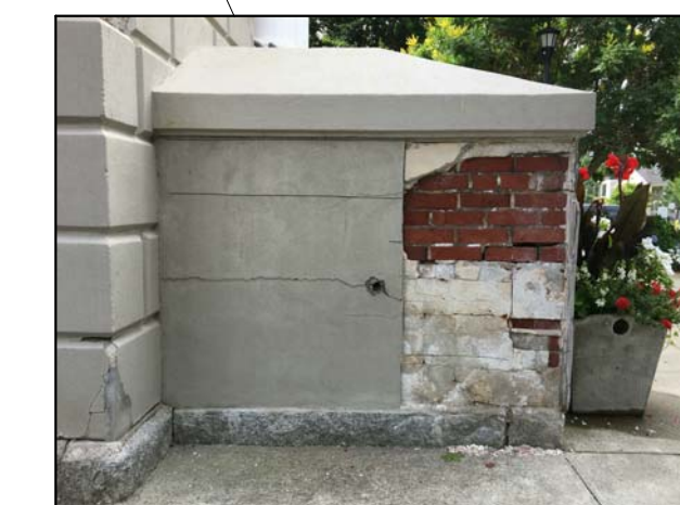
REMOVAL TEST PATCH OF DELAMINATED STUCCO. ALL EXISTING STUCCO TO BE REMOVED, BRICK TO BE REPOINTED, AND NEW STUCCO TO BE INSTALLED AND TOOLED TO MATCH RUSTICATION PATTERN.
