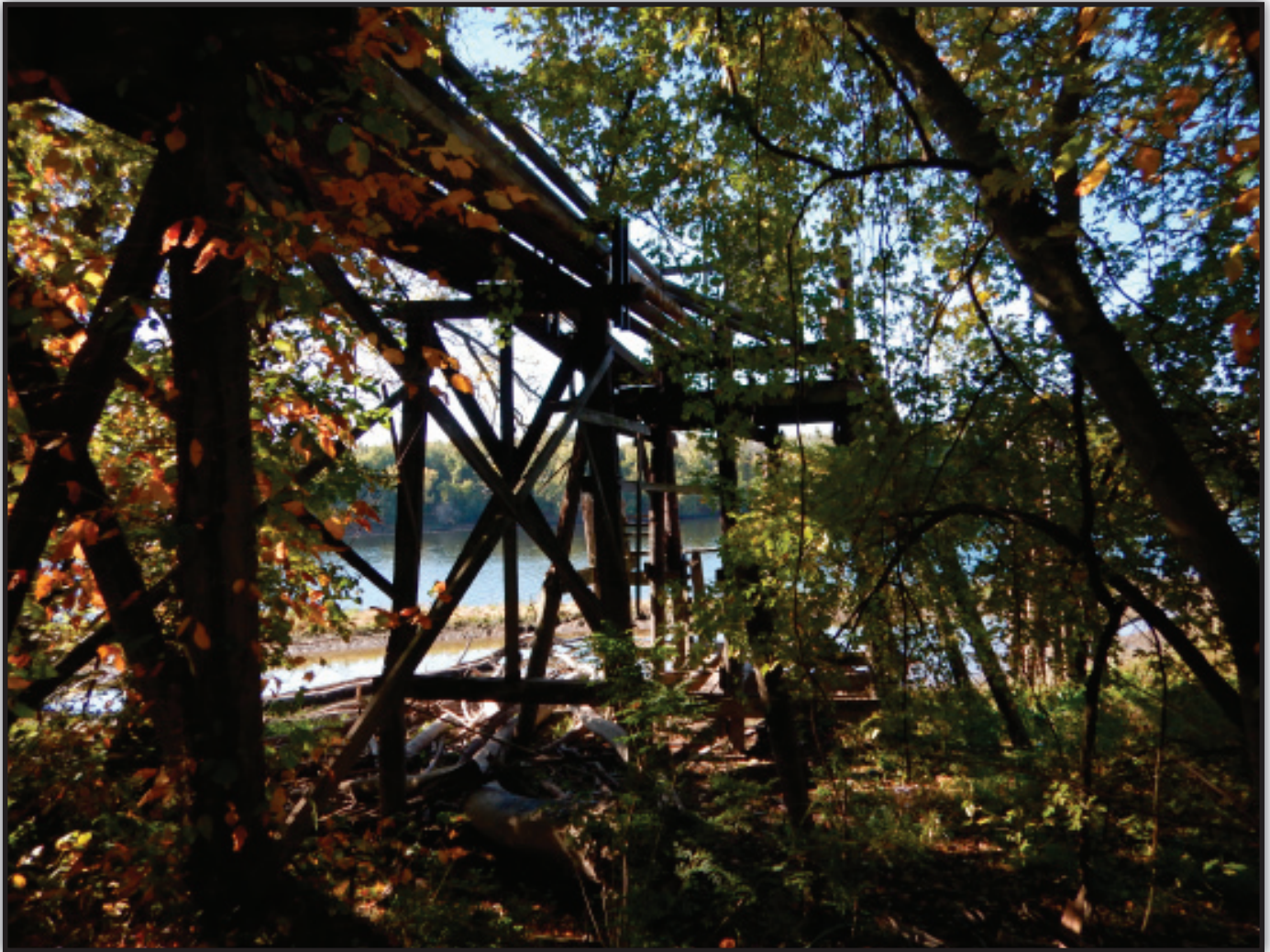
PHOTO 4. Looking west at piping and piping support structure.
