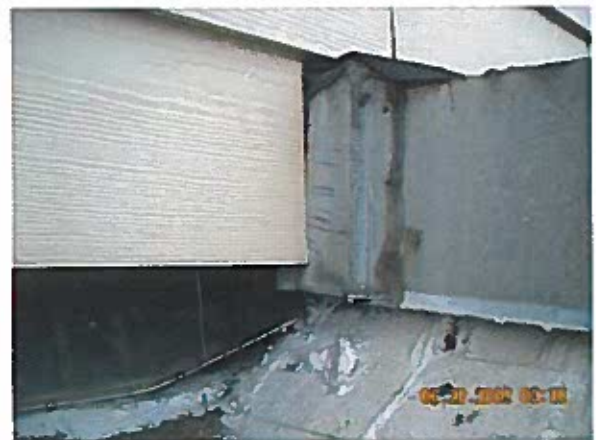
Area 2— Anomaly Poor termination at Area 2 to Area 3 roof areas
