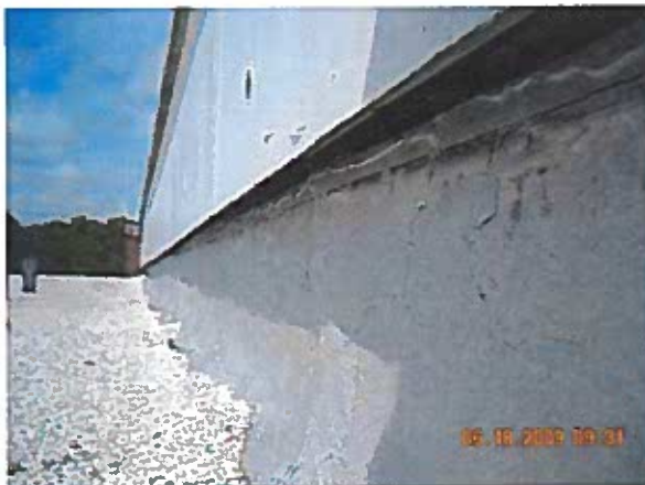
Area 13 — Observation Base flashings are showing signs of distress
