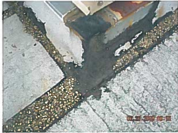
Area 6—Observation Poor base flashing detail (close-up)
