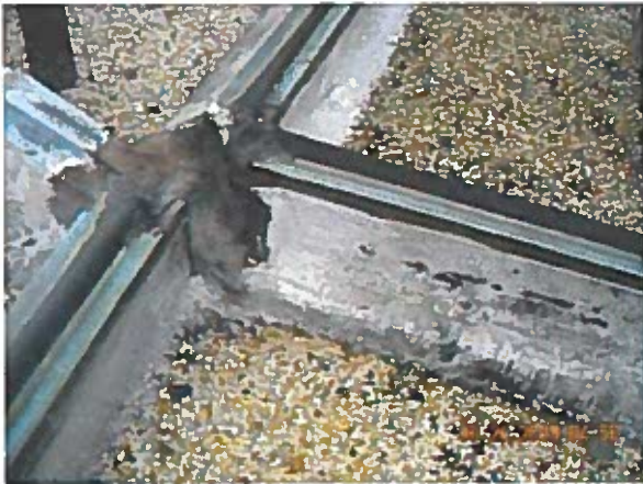
Area 21— Anomaly Poor termination design at expansion joint transition
