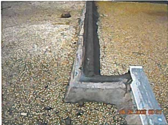
Area 9 — Anomaly Base flashings are in poor/deteriorated condition
