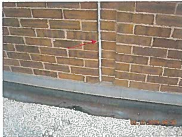
Area 4 — Anomaly Deteriorated joint sealant
