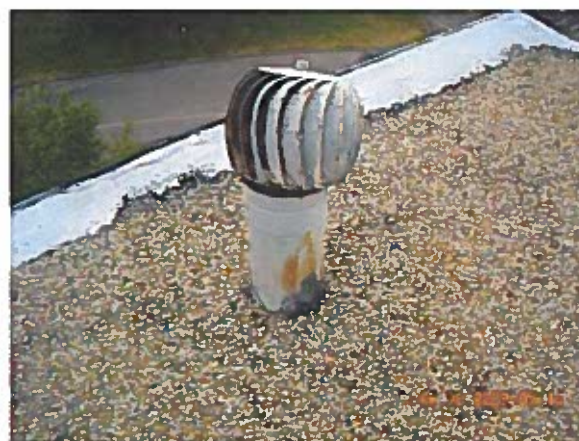
Area 12—Anomaly Turbine vent is broken
