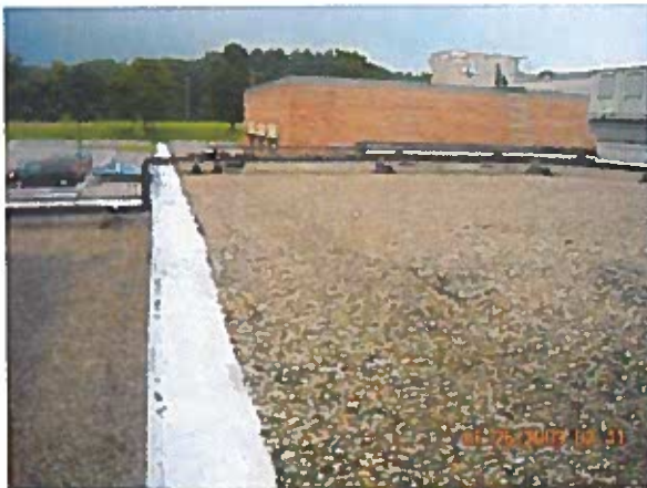
Area 3— Overview Splice patches throughout roof area are delaminating around the edges. NOTE: This condition is typical at all roof locations
