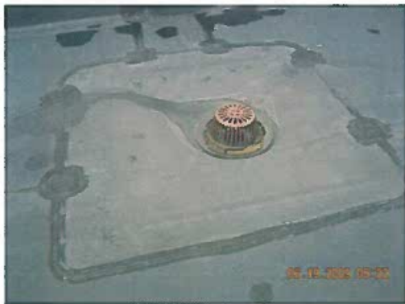
Area 9—Anomaly Surface splices delaminating at edges
