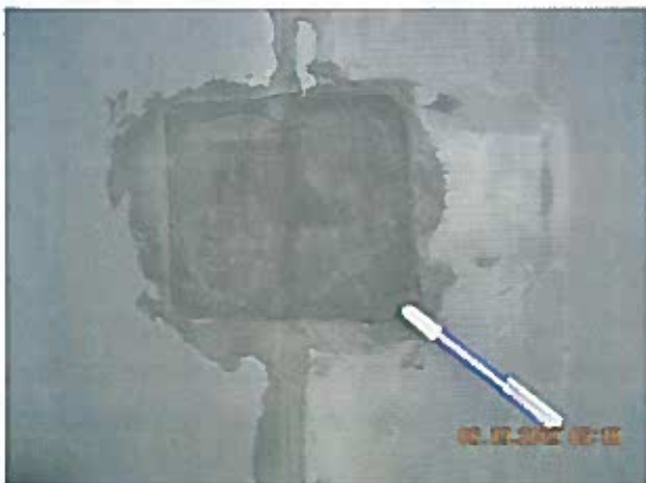
Area 9—Anomaly Surface splices delaminating at edges
