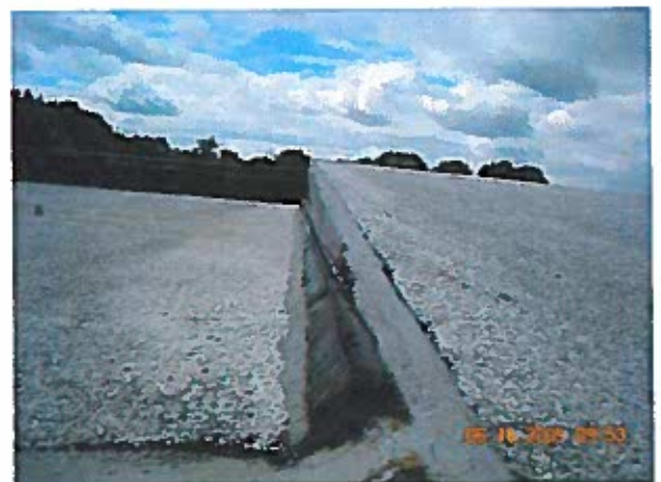
Area 12 — Anomalies Poor roof tie-in at roof transitions
