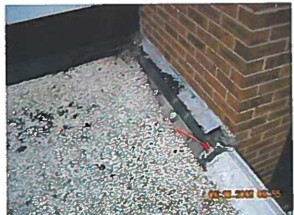
Area 11 — Anomaly Poor tie-in between expansion joint and edge metal
