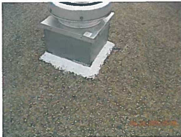
Area 11—Anomaly Missing curb flashing
