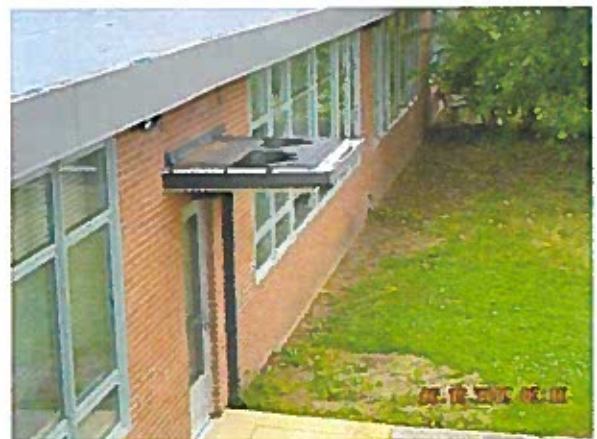
Area 14— Overview and Observations Terminations appear to be in satisfactory condition. Some delamination of splice seams/patches were observed.
