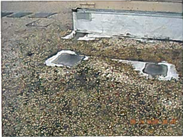
Area 22 — Anomaly Repairs are in poor condition at penetration removal area
