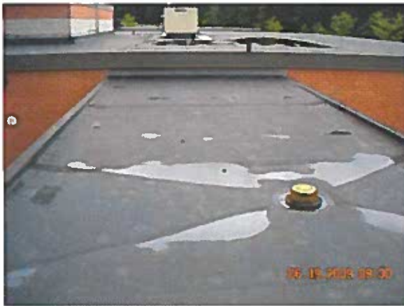
Area 6—Anomalies Splice patches in the field of the roof are delaminating
