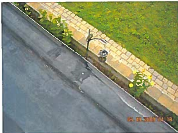
Area 5— Anomaly Splice patches at roof perimeters are open at metal junctions. These areas received remedial repairs where applicable.
