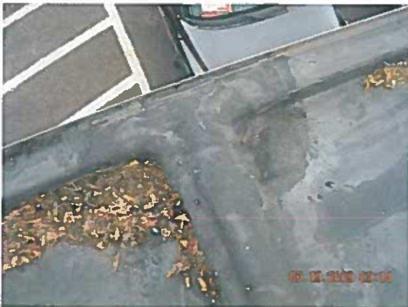
Area 1—Observation View of expansion joint termination at the outside roof edge
