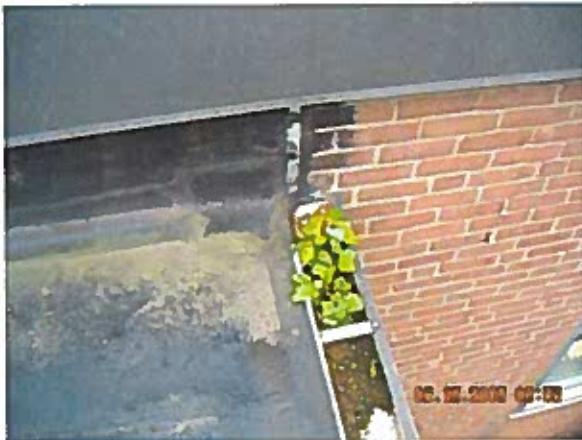
Area 12—Observations Terminations appear to be in satisfactory condition. Gutters were cleared of debris
