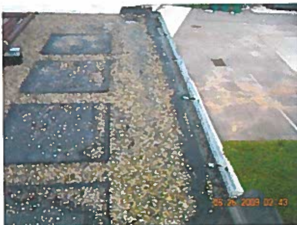
Area 3— Anomaly Damaged strip-in at edge metal
