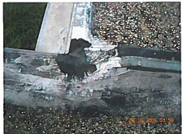
Area 23—Anomaly Expansion joint does not terminate to the perimeter edge
