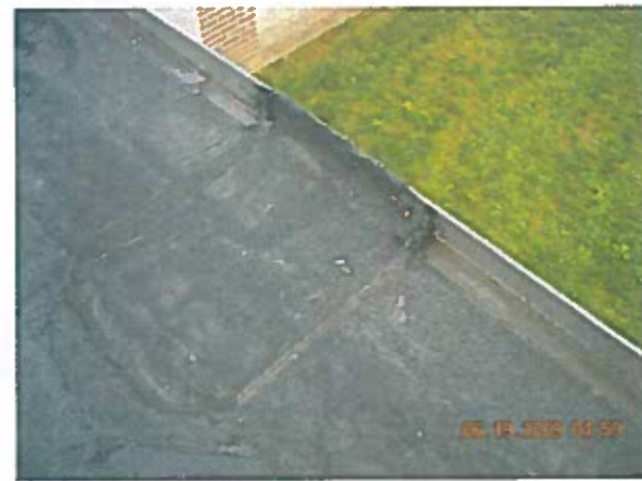
Area 6—Anomaly Surface splice open at roof to vertical transition
