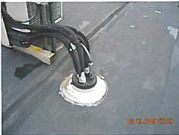
Area 10— Anomaly Conduits clustered through roof penetration pocket
