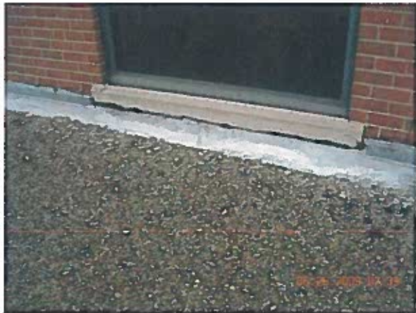
Area 2 — Anomaly Missing termination bar beneath window support sill
