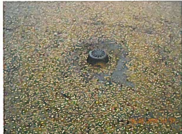
Area 21— Anomaly Some areas of exposed membrane at roof drains
