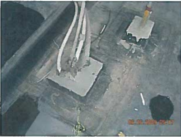
Gymnasium Area 1—Anomaly Plastic coated conduits are not recommended for penetration pockets
