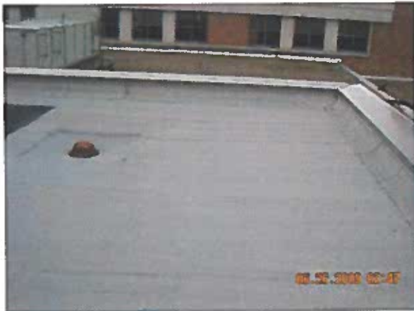
Area 3b —Overview Some areas indicate membrane sheet was overheated when installed.
