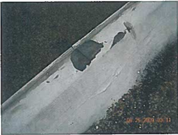
Area 7 — Anomaly Some splits in the strip-in flashings were observed around the perimeter
