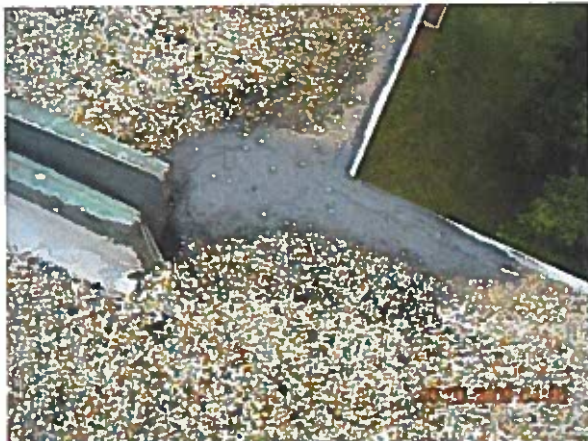
Area 17 — Anomaly Expansion joint did not extend to roof edge causing split in membrane
