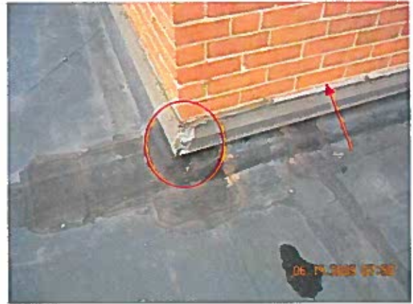
Area 1—Anamoly Deteriorated sealants at top edge of surfaced mounted counter-flashings with open sheet metal miters
