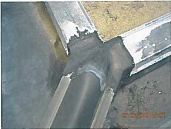
Gymnasium Area 2— Anomaly Termination splices at perimeter edges are delaminating at their edges
