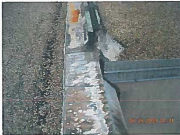
Area 13 — Anomaly Wall joint open at edge metal to expansion joint transition
