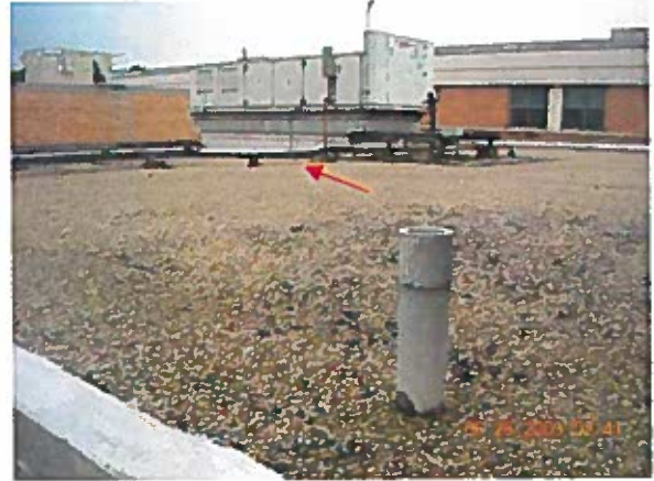
Area 3— Overview Cover strips at edge metal transitions are lifting. Remedial repairs were conducted where moisture wasn't present
