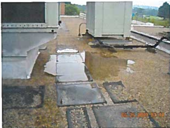
Area 4 — Anomaly Apparent restricted roof drain with missing drain strainer
