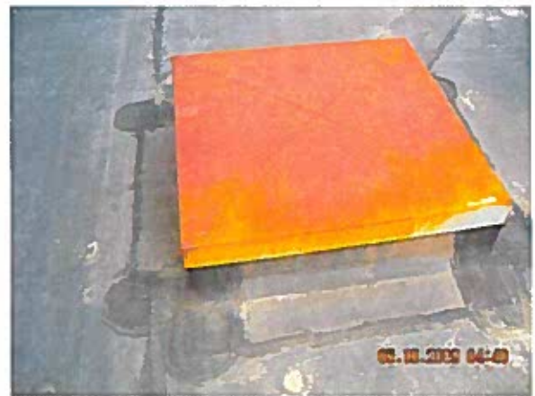
Area 1—Anomaly Galvanized steel curb caps oxidizing
