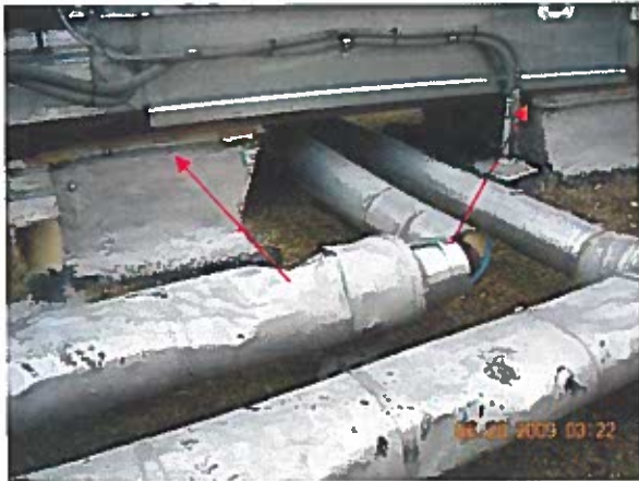
Area 3—Anomaly Low counter flashing trim
