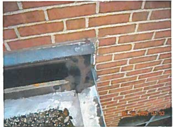
Area 19 — Anomaly Open end on expansion joint termination
