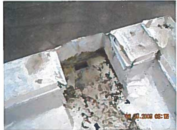
Area 2— Anomaly Scupper metal damaged
