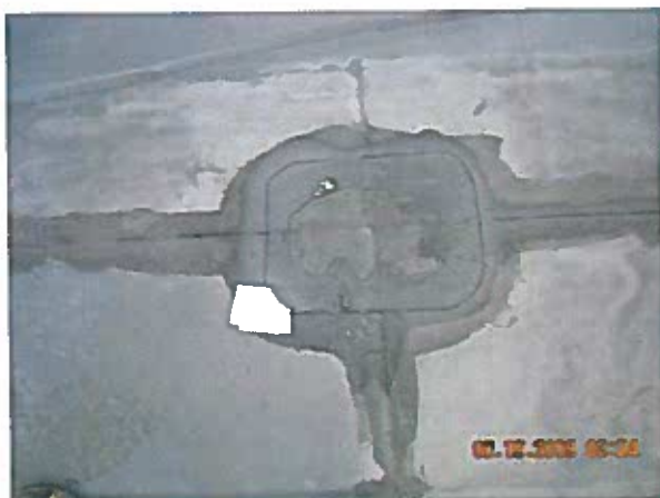
Area 2—Anomaly Splice patches delaminating at their perimeters
