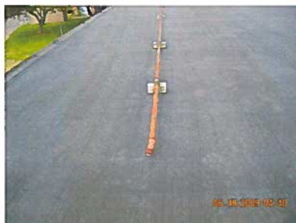
Area 1—Observation Unused utility pipe—Recommend removal
