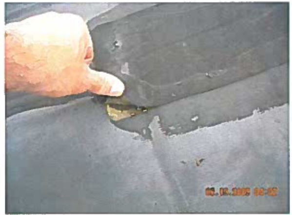
Area 4— Anomaly Splice patches are delaminating in many areas
