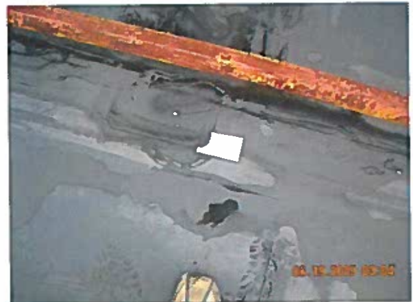
Area 1— Anomaly Splice patches are delaminating at their perimeters
