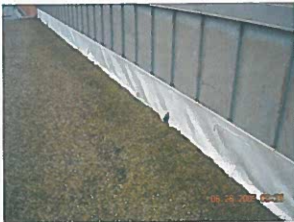
Area 5 — Anomaly Loose base flashings along wall
