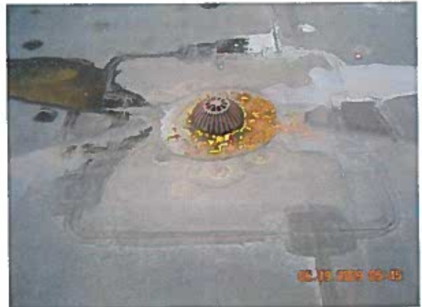
Area 12—Anomaly Target patches are delaminating in areas
