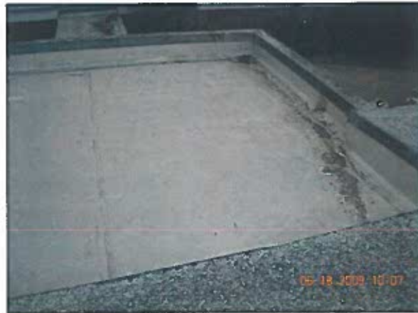
Area 19 — Overview Gravel was removed from the membrane surface
