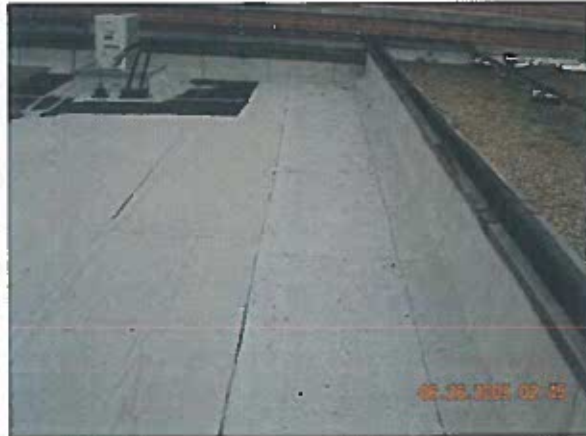
Area 3a —Anomaly Splice lap is delaminating along the edge at most locations.
