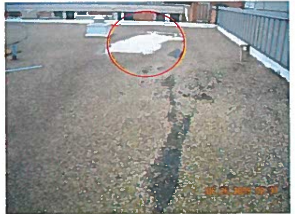
Area 1— Anomalies Additional areas of exposed membrane. Circle indicates a restricted roof drain leader
