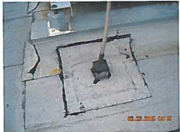
Area 9b — Anomaly Plastic conduits are not recommended to penetrate a penetration pocket
