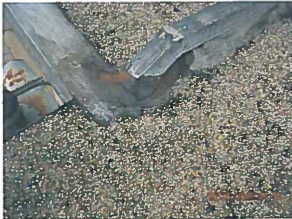
Area 20 — Anomaly Expansion joint does not correctly terminate to the perimeter edge
