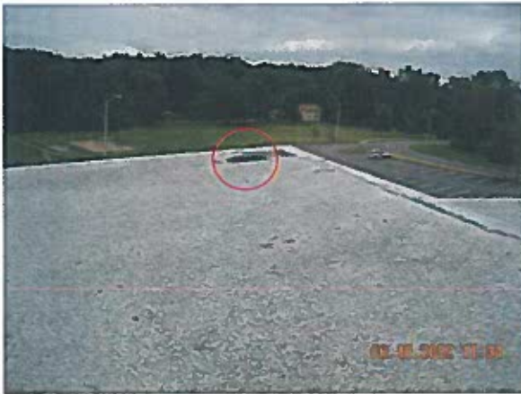
Area 8 — Anomalies Some exposed membrane areas
