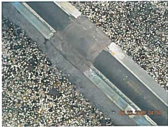
Area 20 — Anomaly Expansion joint cover strips are loose
