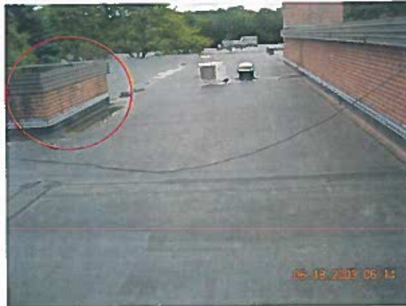
Area 2—Overview NOTE: Small raised roof area ponds water and has failed edge metal strip-in flashings around perimeter
