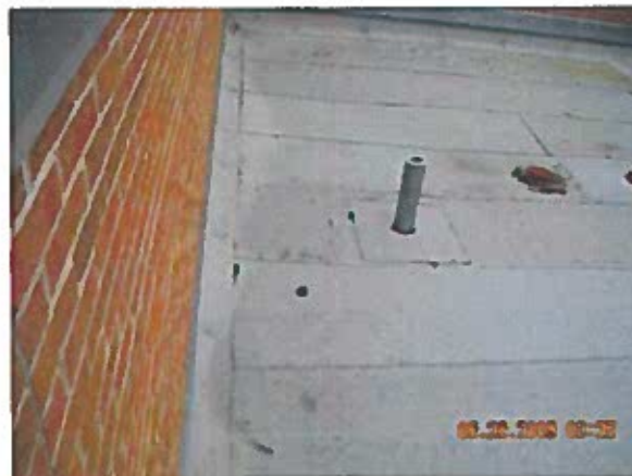
Area 5a—Anomaly Some areas of membrane were installed with excessive wrinkles in the sheet
