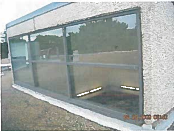
Area 4—Anomaly Cracked cementitious board on skylight
