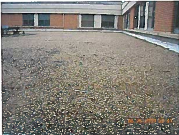
Area 3— Overview Splice laps are delaminating at some roof drain targets
