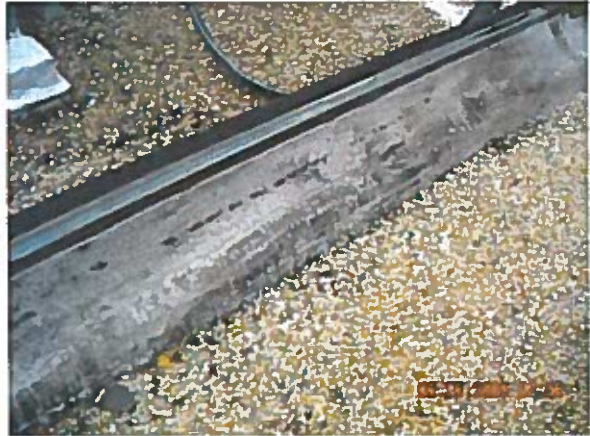
Area 21— Anomaly Base flashings are on poor condition
