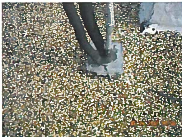
Area 10 — Anomaly Penetration pipes mastic deteriorating are clustered along with
