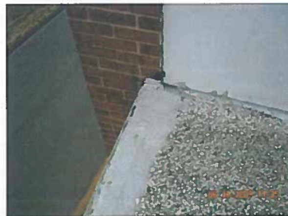
Area 7 — Anomaly Poor edge metal termination
