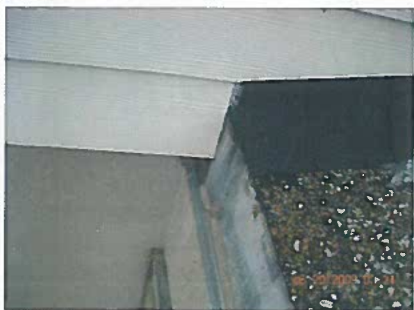
Area 3—Anomaly Poor expansion joint detail with open laps
