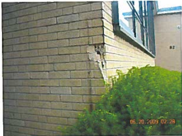
Damaged brick observed
