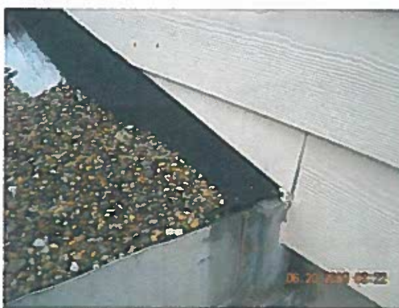
Area 3—Anomaly Poor expansion joint detail with open laps
