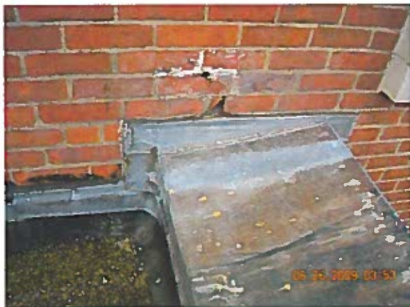
Area 9 — Observation Brick work damage at coping termination
