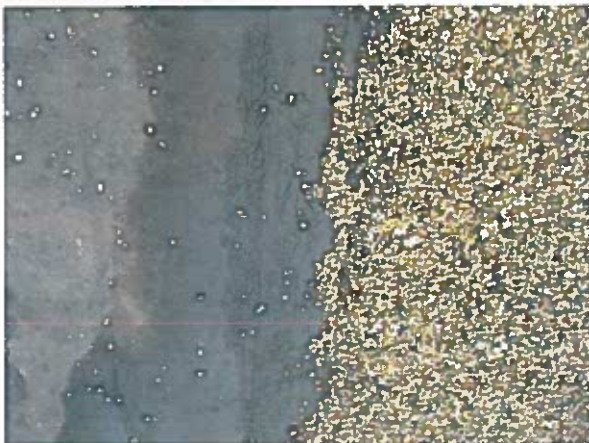
Area 1— Anomaly Tie-in on repair beginning to deteriorate
