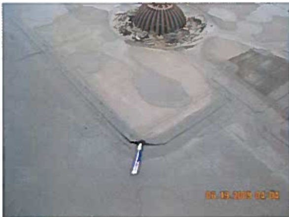
Area 4— Anomaly Splice targets are delaminating around the edges
