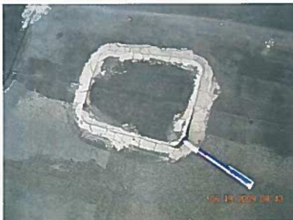
Area 8 — Anomalies Splice patches at edge metal transitions are delaminating, splice patches in the field of the roof are delaminating and counter-flashing sealants are deteriorating
