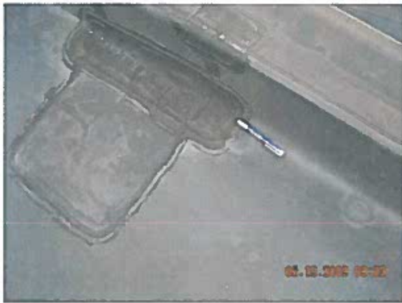
Area 5 — Anomalies Splice patches at wall transitions around the perimeter are delaminating
