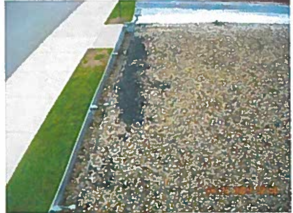
Area 14 — Anomaly Exposed membrane was observed in many areas around the perimeter edge metal
