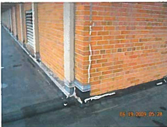
Area 10— Observation Wall crack was typically repaired in the past. Current sealants are deteriorating.
