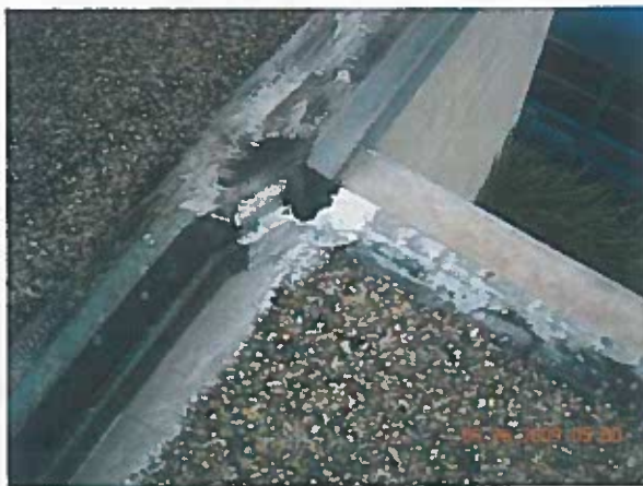
Area 24—Anomaly Expansion joint does not terminate to the perimeter edge
