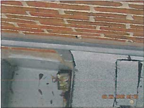
Area 5c — Overview NOTE: Roof area appears to be in satisfactory condition
