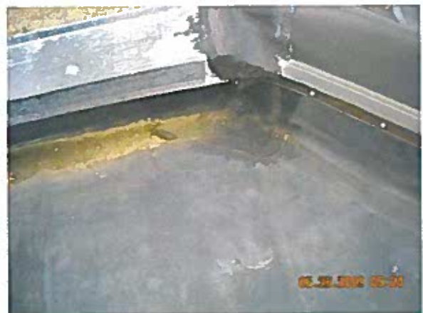
Gymnasium Area 2—Anomaly Many splice are delaminating
