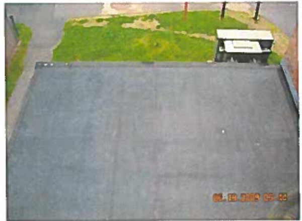
Area 7—Anomalies Edge metal cover strips are splitting or delaminating
