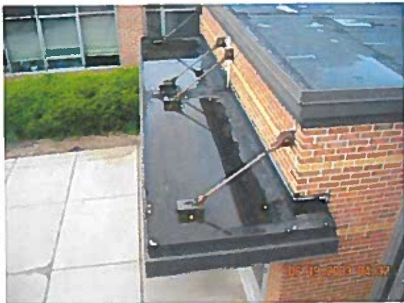
Area 7—Overview and Observation Note: Ponding water
