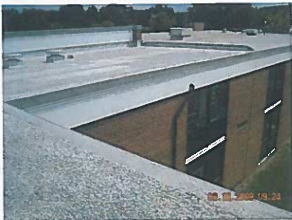
Area 13 — Overview and Observations Terminations appear to be in satisfactory condition. Some delamination of splice seams/patches were observed.
