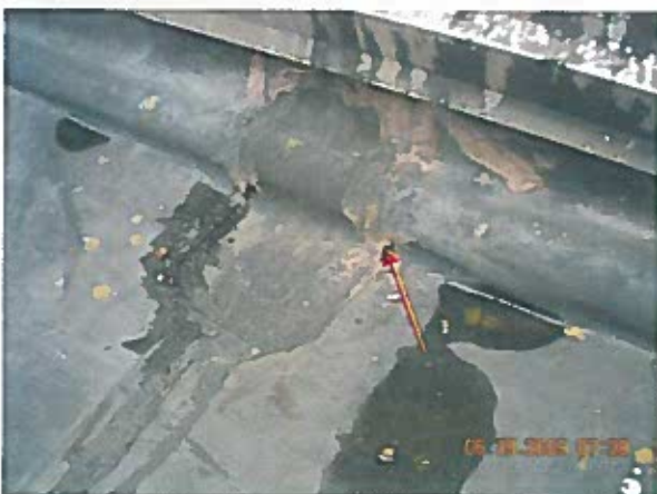
Area 1—Anomaly Openings in splice patches. Remedial repairs were conducted in these areas.
