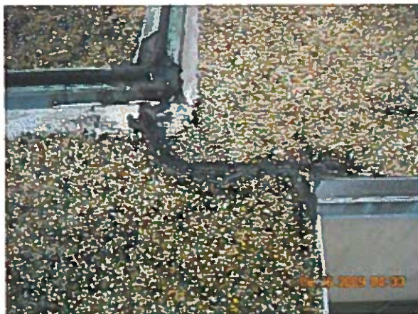
Area 15 — Anomaly Expansion joint did not extend to roof edge causing split in membrane
