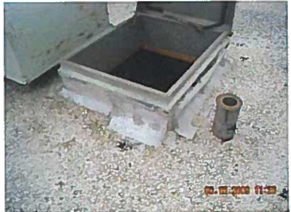
Area 7 — Anomaly Poor base flashing installation at roof hatch
