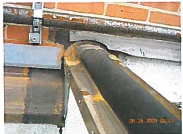
Area 3— Anomaly Open sealant at expansion joint termination
