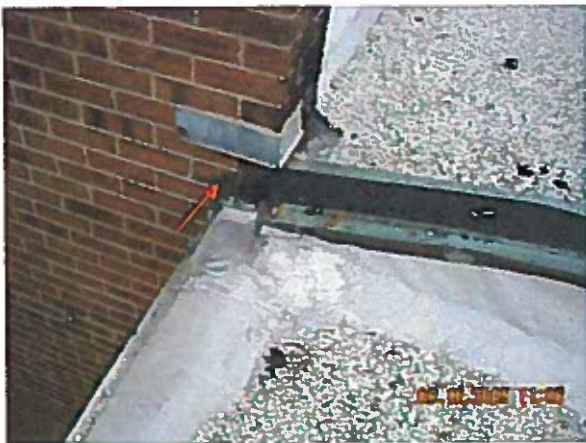
Area 6 — Anomaly Expansion joint does not extend past metal edge
