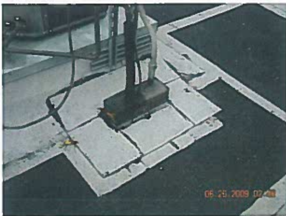
Area 3a —Anomaly Refrigerant pipe insulation extends into pourable sealer
