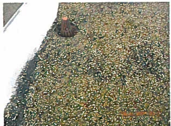
Area 7 — Anomaly Some exposed membrane was observed around roof drains
