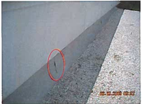
Area 13 — Anomaly Base flashing laps are not fully adhered
