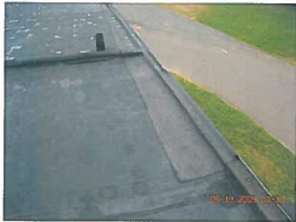
Area 2— Anomaly View of roof repair where building was modified. Splice patch appears open at termination points
