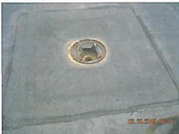
Area 6 — Anomaly Missing roof drain strainers, splice laps are delaminating at some roof drain targets, many splice patches are delaminating and edge metal cover strips are splitting or delaminating
