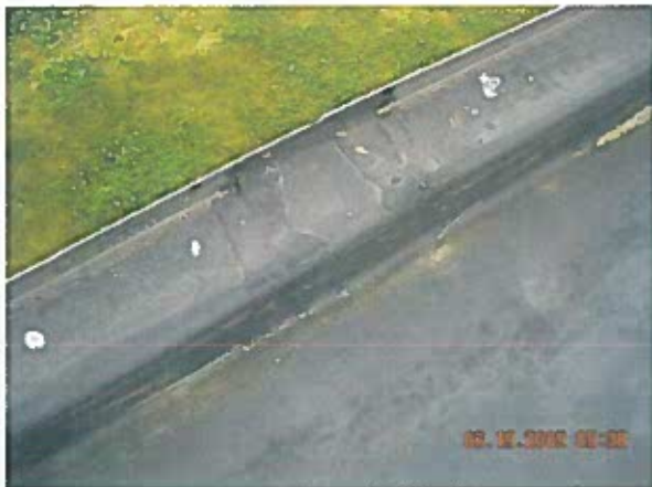
Area 11—Anomaly Splice patches along perimeter are delaminating from edge metal
