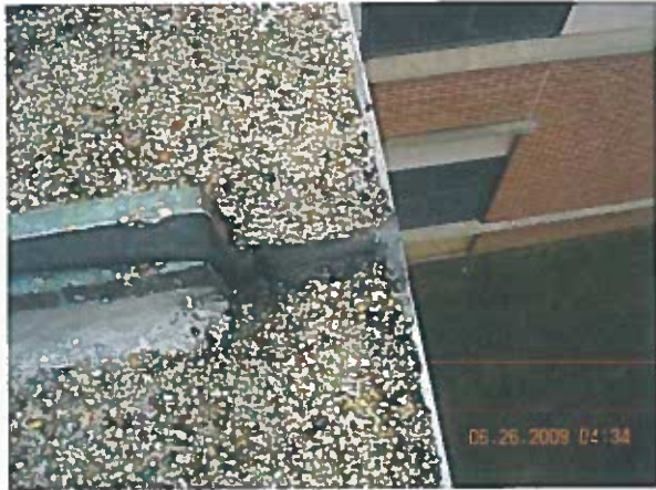
Area 16 — Anomaly Expansion joint did not adequately extend to roof edge
