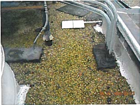
Area 4 — Anomaly Pipe penetrations are clustered
