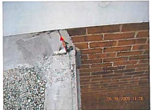
Area 6 — Anomaly Missing termination on base flashing
