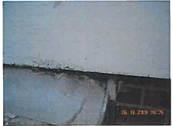
Area 13 — Anomaly Base flashing is not terminated at edge metal
