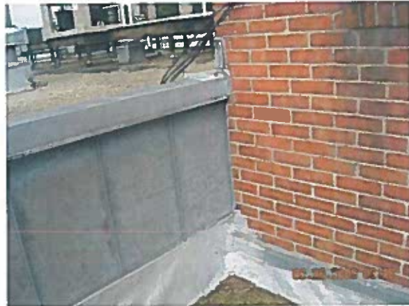
Area 5 — Anomaly Open metal work at wall transitions
