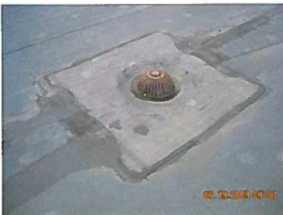
Area 2—Anomaly Splice laps are delaminating at some roof drain targets NOTE: Splice patches about area are delaminating around the edges.
