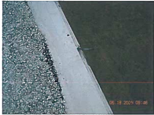
Area 14 — Anomaly Strip-in membrane along perimeter is not adhered to edge metal. Remedial repairs were conducted at these locations
