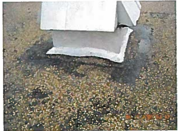
Area 4 — Anomaly Base flashings are damaged around curb unit
