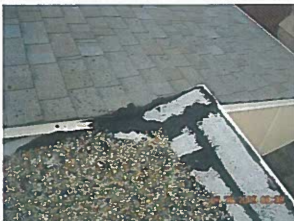
Area 9—Anomaly Poor tie-in detail at built-up to shingle transition
