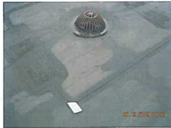
Area 5— Anomaly Target patches delaminating at edges
