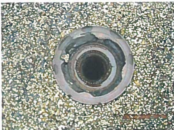
Area 11—Anomaly Missing drain strainer
