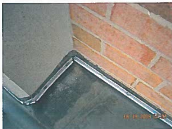
Area 6—Anomaly Sealant deterioration at termination bar
