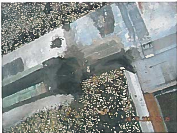
Area 16 — Anomaly Expansion joint did not extend to roof edge
