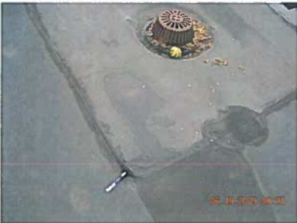
Area 5 — Anomalies Splice laps are delaminating at some roof drain targets NOTE: Splice patches about area are delaminating around the edges.
