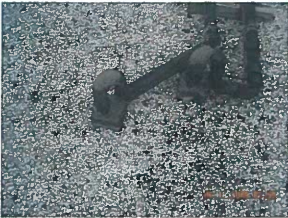
Area 1— Anomaly Non-waterproofed pipe insulation appears to extending into pourable sealer pocket
