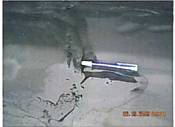
Area 4— Anomaly Many splice patches are delaminating at the transitions
