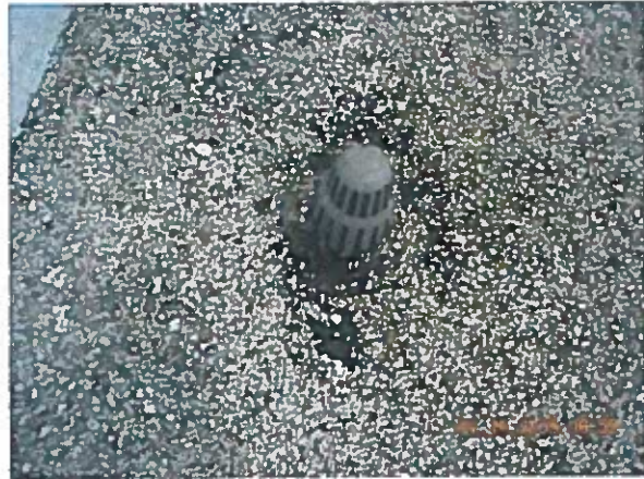
Area 11 — Anomaly Broken roof drain strainer
