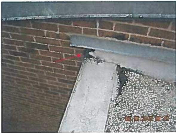
Area 4 — Anomaly Base flashing does not extend beyond roof edge metal
