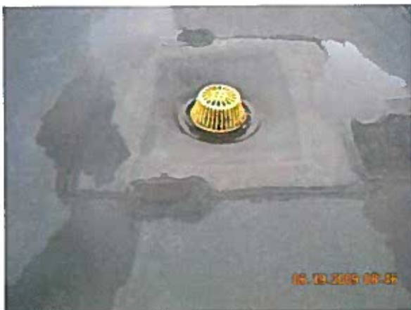
Area 9 — Anomaly Open splices on roof drain targets
