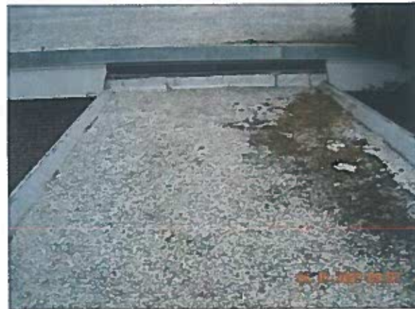
Area 11 — Anomalies Debris was removed from the roof surface
