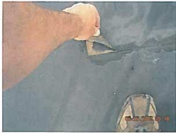
Gymnasium Area 1—Anomaly Many splice patches are delaminating
