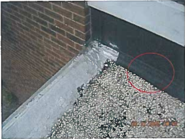
Area 11 — Anomaly Expansion joint material is deteriorated
