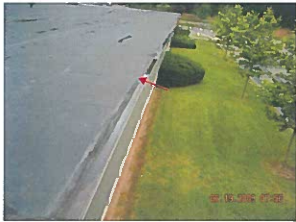
Area 1—Anamoly Cover strips at edge metal transitions are lifting. Remedial repairs were conducted where moisture wasn't present
