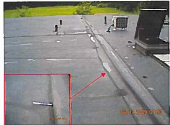
Area 2—Anomaly Splice lap is delaminating along the edge at most locations.
