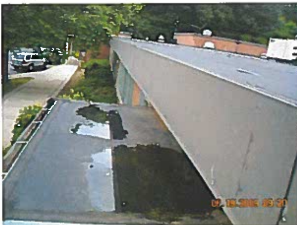
Area 13— Overview and Observations Terminations appear to be in satisfactory condition. Some delamination of splice seams/patches were observed.
