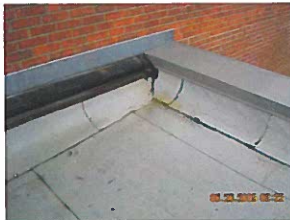
Area 5b—Anomaly Open expansion joint corner (sealant) and some areas of membrane were installed with excessive wrinkles in the sheet
