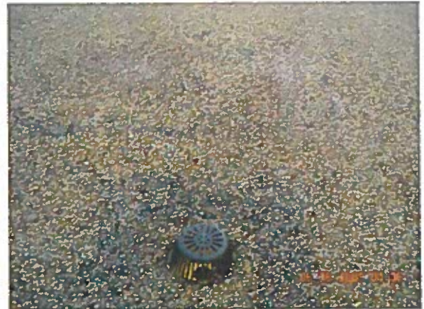
Area — anomaly Exposed membrane was observed around roof drain areas
