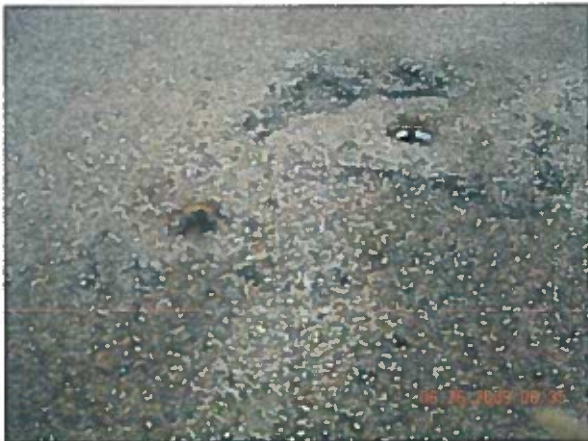
Area 9—Anomaly Missing drain strainers
