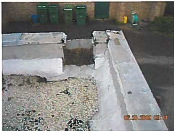
Area 2— Anomaly Scupper metal damaged
