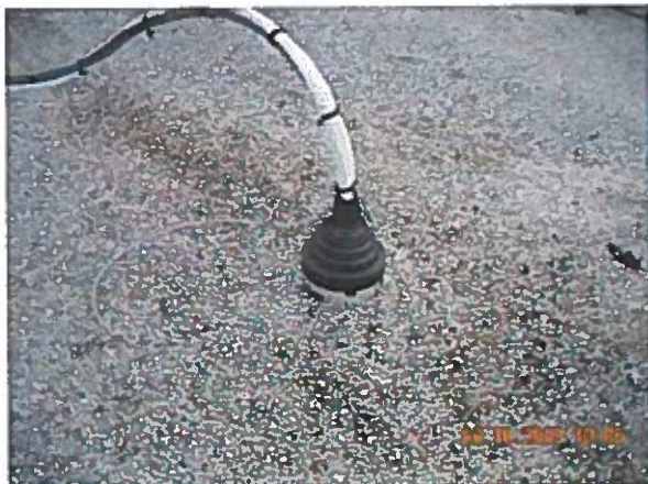
Area 15 — Anomaly Poor installation of refrigerant pipes
