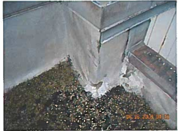
Area 12 — Anomaly Damaged base flashing
