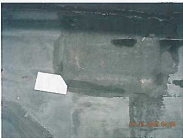
Area 4—Anomaly Splice patches delaminating in many areas
