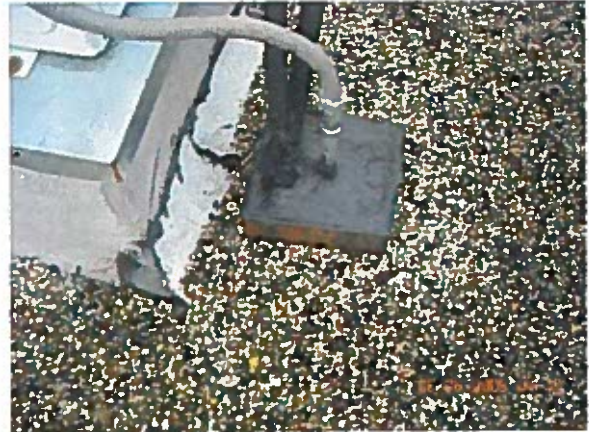
Area 22—anomaly Insulated pipe installed into penetration pocket
