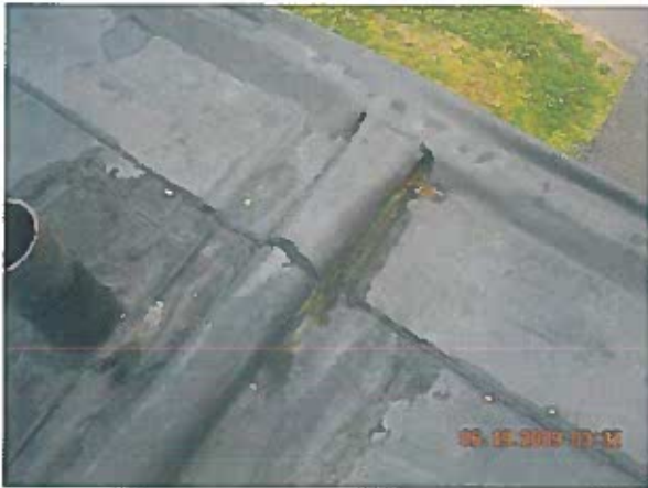
Area 2—Anomaly Repair patch was not flashed into the expansion joint
