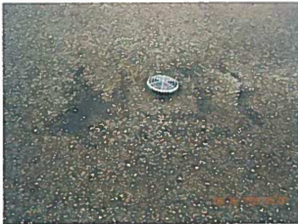
Area 24—Anomaly Some areas of exposed membrane at roof drains
