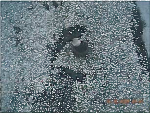
Area 14 — Anomaly Exposed membrane and broken roof drain strainer
