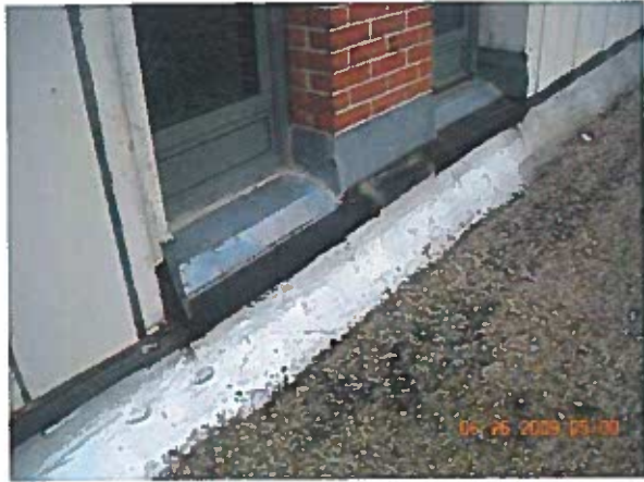
Area 24—Anomaly Several open cover strips at window area
