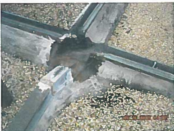
Area 20 — Anomaly Expansion joint transitions are in poor condition
