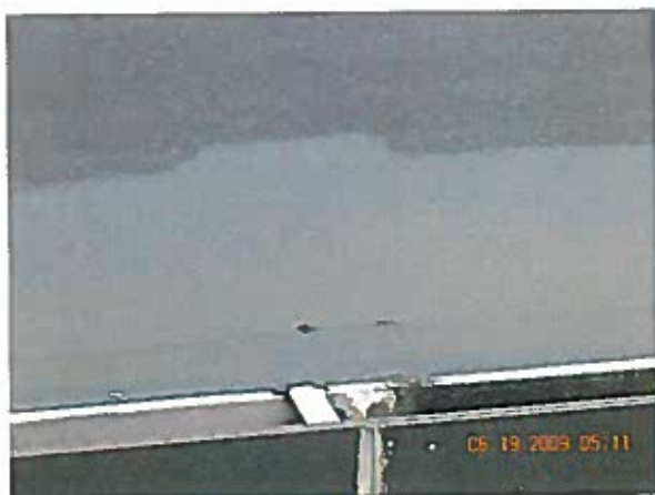
Area 8—Observation Fasteners appear to be protruding beneath membrane
