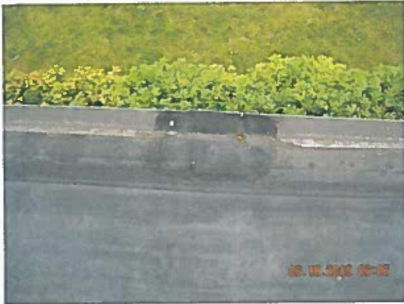
Area 1—Anomalies Cover plate strip-ins are splitting at seam, many splice patches about roof area delaminating and roof drain target splices are delaminating around the edges
