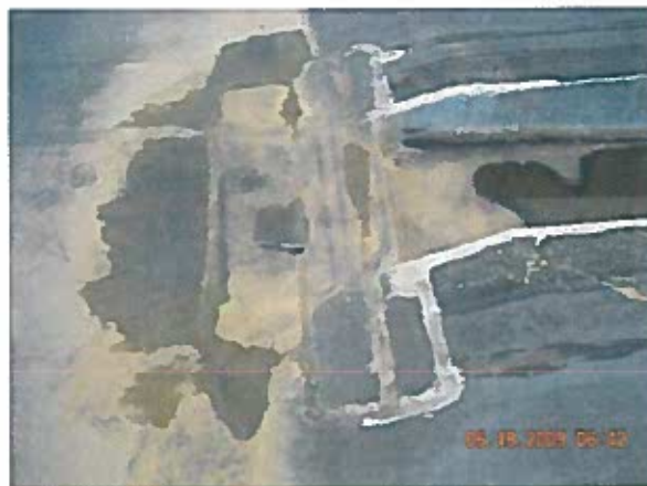
Area 6 — Anomaly Strip-in flashings a open around scupper flashing
