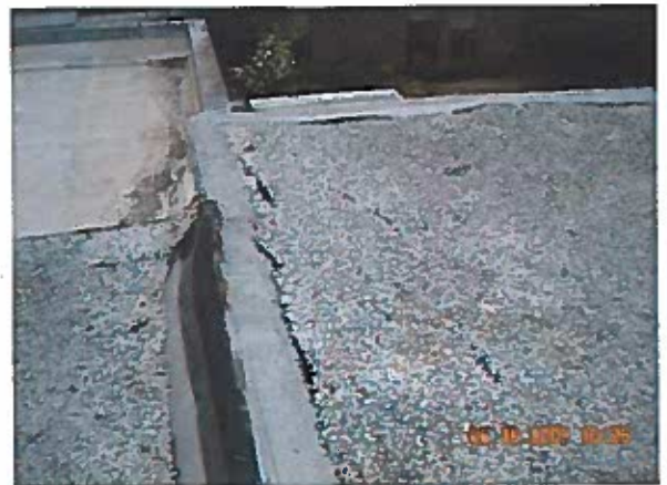
Area 16 — Anomaly Expansion joint does not extend to the roof's perimeter
