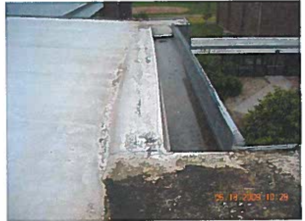
Area 20 — Anomaly Gutter appears to be back-pitched
