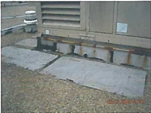
Area 6—Observation Poor base flashing detail
