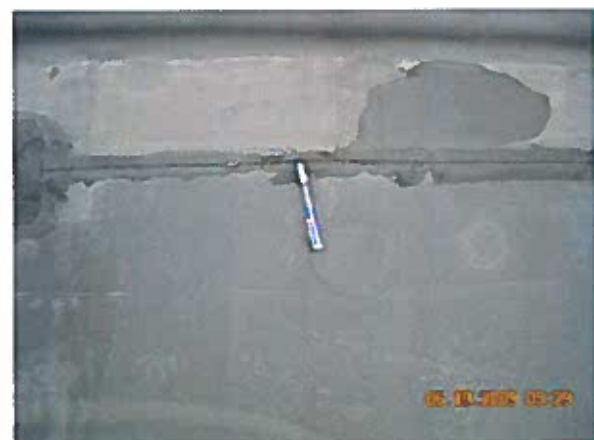
Area 10—Anomaly Expansion joint cover strip is delaminating in areas
