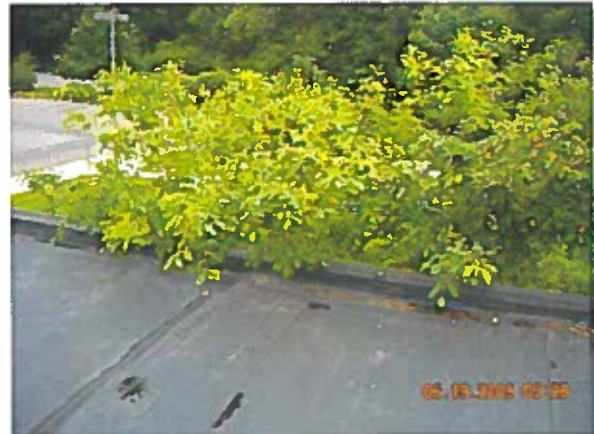
Area 10—Anomaly Vegetation should be trimmed back from roof area
