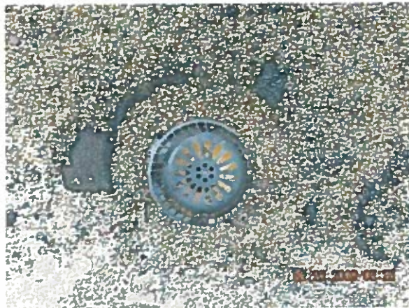
Gymnasium Area 3— Anomaly Exposed membrane was observed around roof drain
