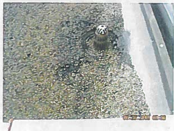
Gymnasium Area 5 — Anomaly Exposed membrane observed at roof drain
