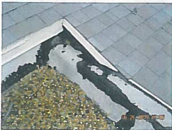
Area 10—Anomaly Poor base flashing detail at transition
