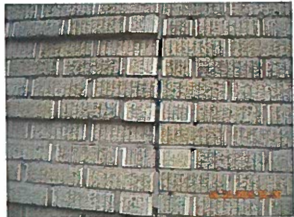
Wall joints in need of repair
