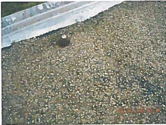
Area 5—Anomaly Excessive gravel buildup at roof's perimeter
