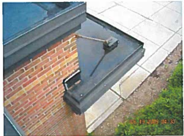
Area 7—Overview and Observation Note: Ponding water
