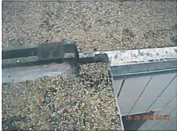
Area 18 — Anomaly Expansion joint did not extend correctly to roof edge causing split in membrane
