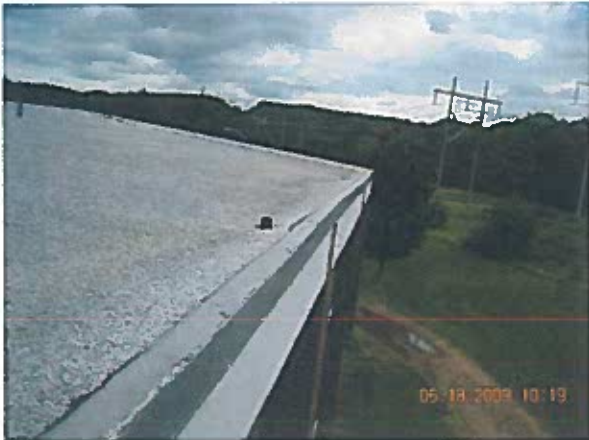
Area 18 — Observations Some minor strip-in flashings are un-adhered to the edge metal. Remedial repairs were conducted at these locations.
