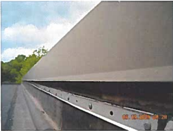
Area 6—Anomalies Splice patches in the field of the roof are delaminating and counter-flashing sealants are deteriorating
