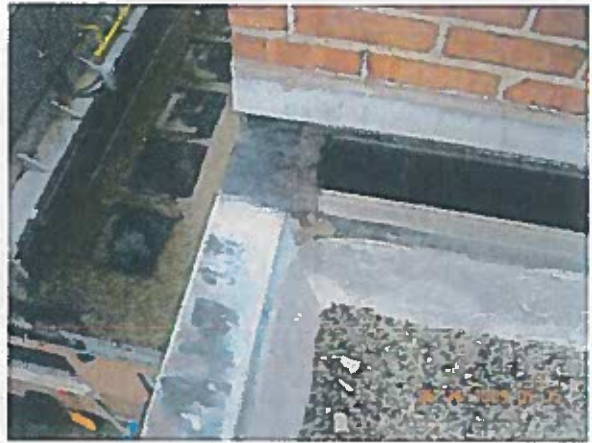
Gymnasium Area 6 — Observation Expansion joint does not extend to the outside edge
