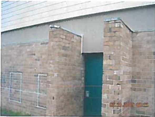
View of unsecured metal caps (typical) NOTE: Contractor secured all metal caps
