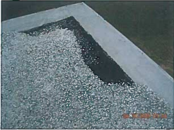
Area 14 — Anomaly NOTE: Exposed membrane in isolated areas
