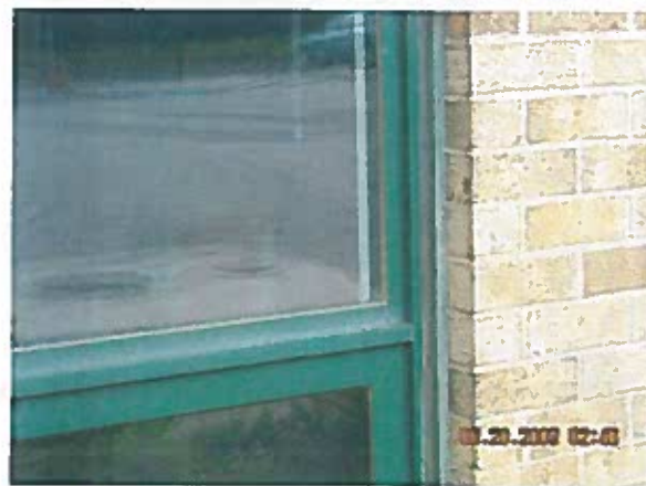
Window perimeter sealants in poor condition
