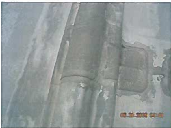
Area 6—Anomaly Splice patches over expansion joints are delaminating
