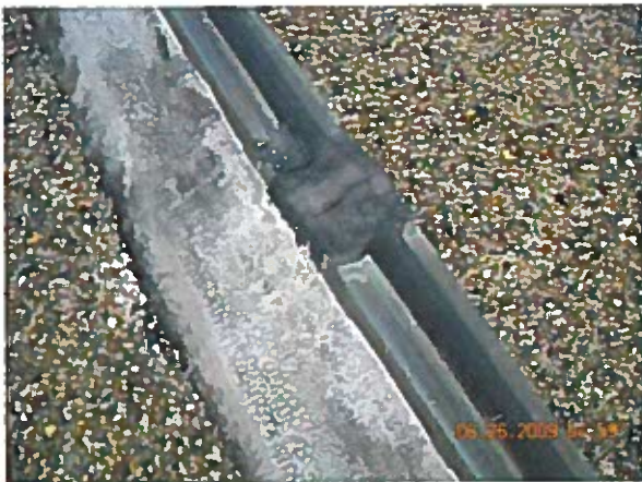
Area 23— Anomaly Expansion joint cover strips are delaminating
