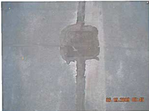
Area 12—Anomaly Splice patches are delaminating in areas
