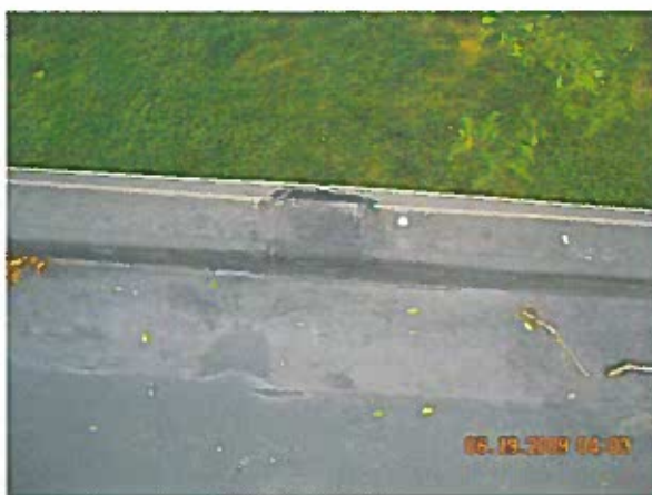
Area 4— Anomaly Splice patches at roof perimeters are open at metal junctions. These areas received remedial repairs where applicable.
