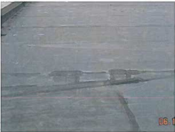
Area 1—Anamoly Splice patches throughout roof area are delaminating around the edges. NOTE: This condition is typical at all roof locations
