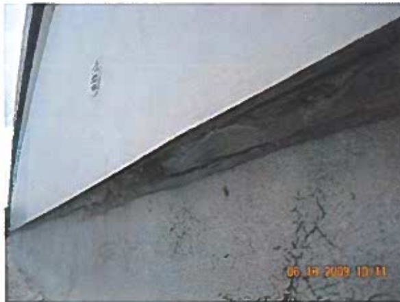
Area 17 — Anomaly Base flashing missing termination securement
