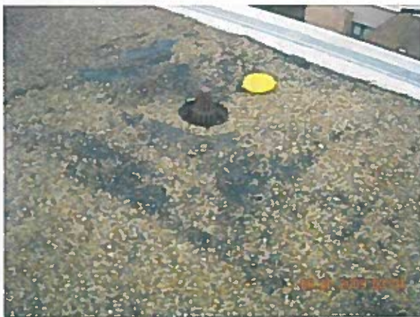
Area 1—Anomaly Exposed membrane felts around roof drains
