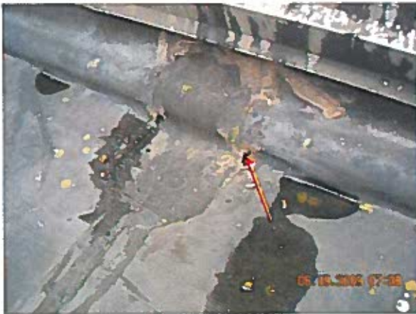
Area 1—Anamoly Open voids at cover strip transitions
