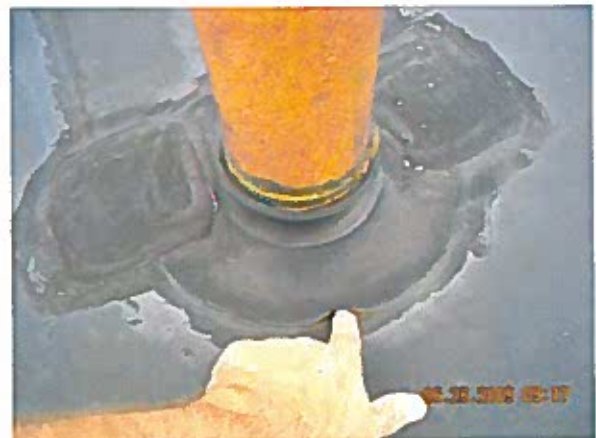
Gymnasium Area I—Anomaly Some pipe boots are deteriorated with delaminating splices
