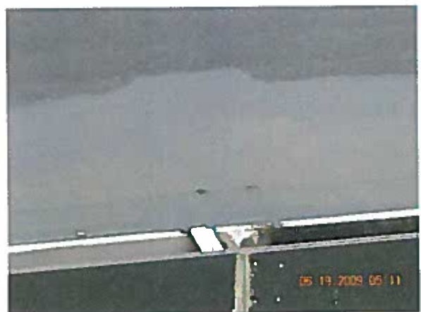
Area 8—Overview Sealants appear to be deteriorating at gutter laps.
