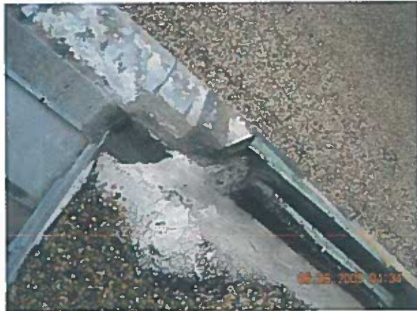
Area 16 — Anomaly Expansion joint open at the roof edge
