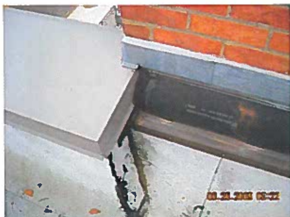
Area 5b — Anomaly Open expansion joint corner (sealant)
