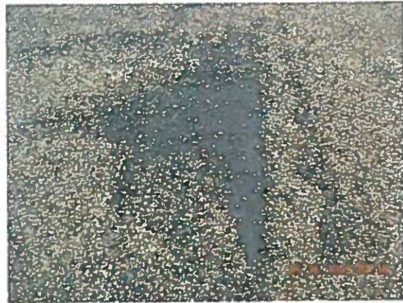
Area 5—Anomaly Apparent exposed membrane areas
