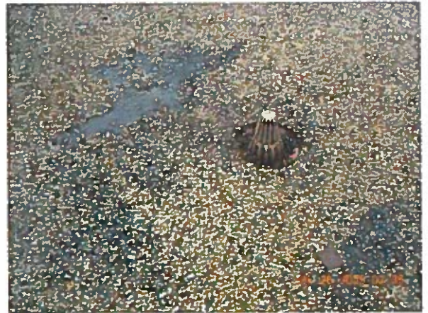
Area 1— Anomalies Exposed membrane felts at roof drain. Similar exposed felt conditions appear around perimeter edges
