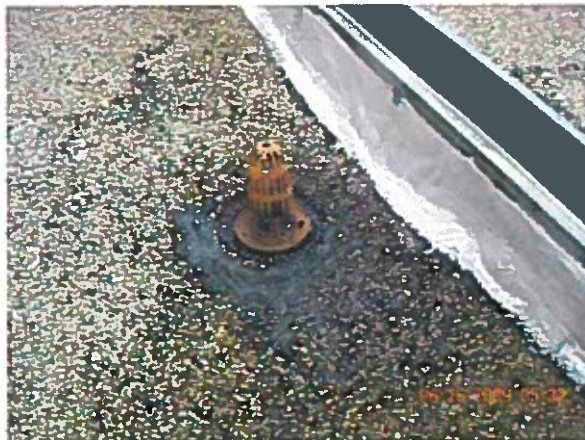
Gymnasium Area 5 — Anomaly Exposed membrane was observed at roof drain
