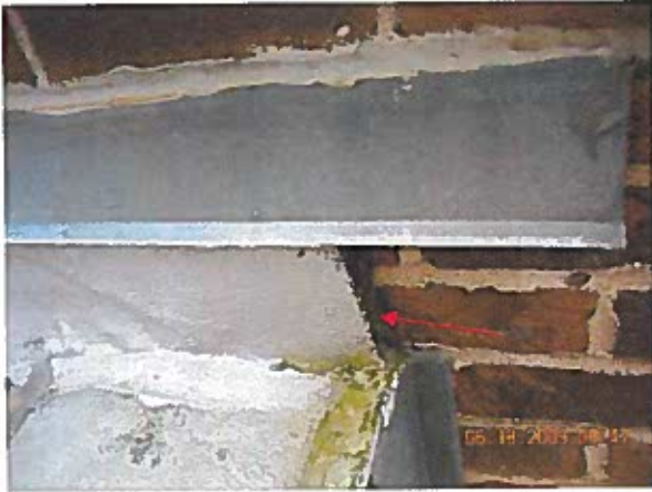
Area 3 — Anomaly Termination securement missing at this location
