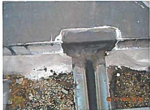
Area 10 — Anomalies Sealants deteriorating at expansion joint transitions
