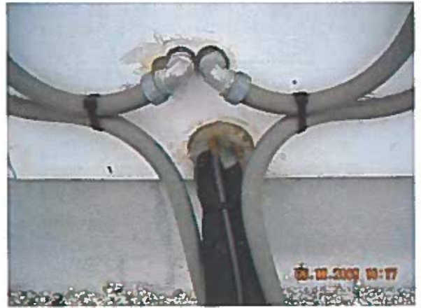
Area 17 — Anomaly Conduits are not sealed at through wall locations
