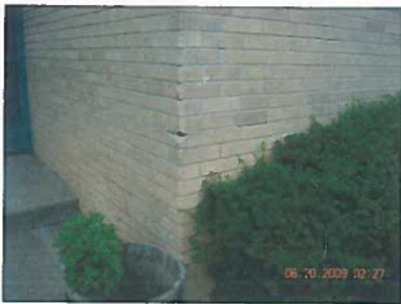
Some damaged brick was observed
