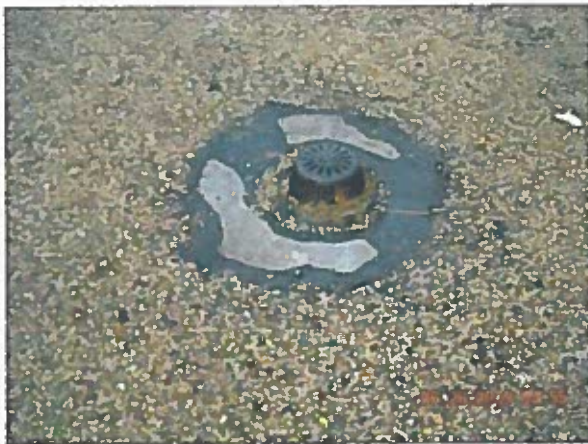
Area 20 — Anomaly Drain flashings membrane is exposed
