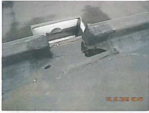
Area 3 —Anomalies Open laps at all scuppers, splice patches at edge metal transitions are delaminating and splice patches in the field of the roof are delaminating
