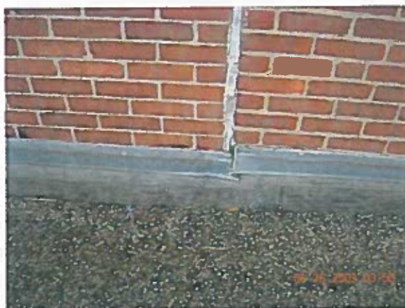
Area 8 — Observation Wall joints sealants are deteriorated
