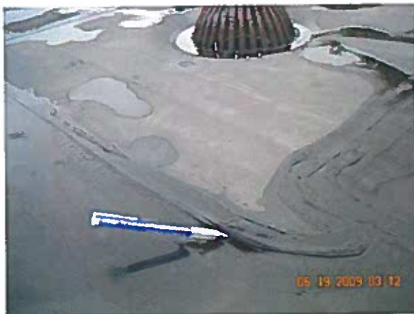
Area 1— Anomaly Target splices are delaminating at their perimeters
