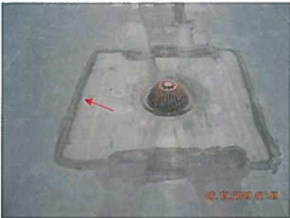
Area 1—Anamoly Splice laps are delaminating at some roof drain targets
