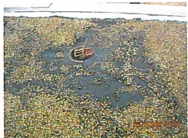
Area 1—Anomaly Broken drain strainer along with exposed membrane felts
