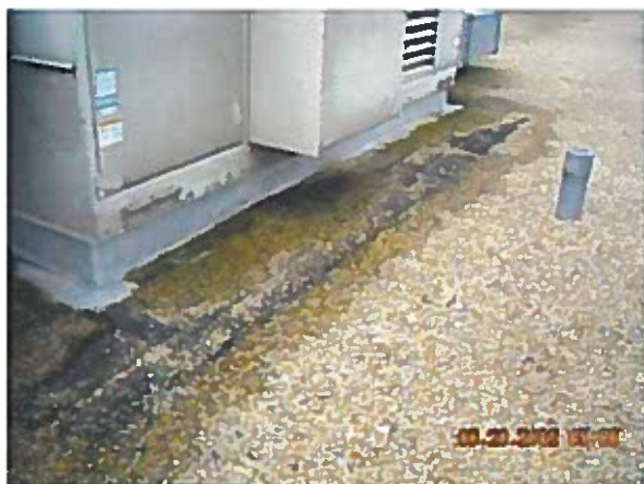
Area 11—Anomaly Roof repair is showing indications of deterioration
