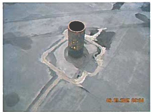
Area 4— Anomaly Target patches at roof projections are delaminating at many areas.
