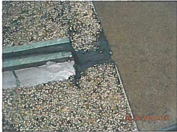
Area — Anomaly Expansion joint did not extend correctly to roof edge causing splits in membrane
