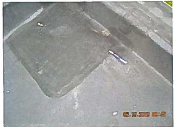
Area 9 — Anomalies Splice patches at edge metal transitions are delaminating, splice patches in the field of the roof are delaminating
