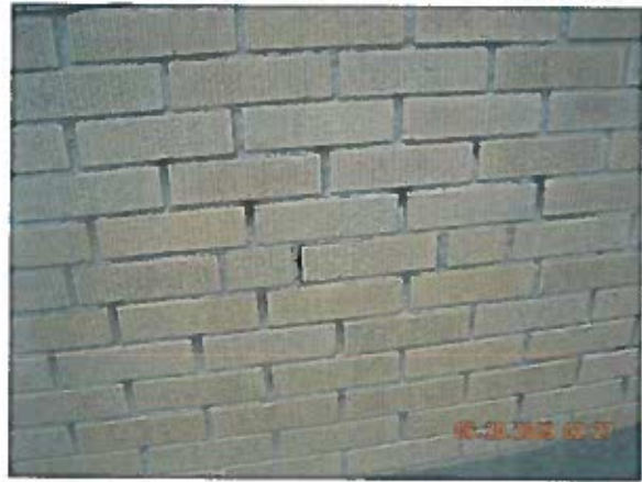
Mortar joints appear to be deteriorating
