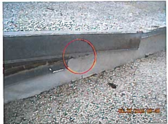
Area 3 — Observation Suggest applying counter flashing metal over area shown
