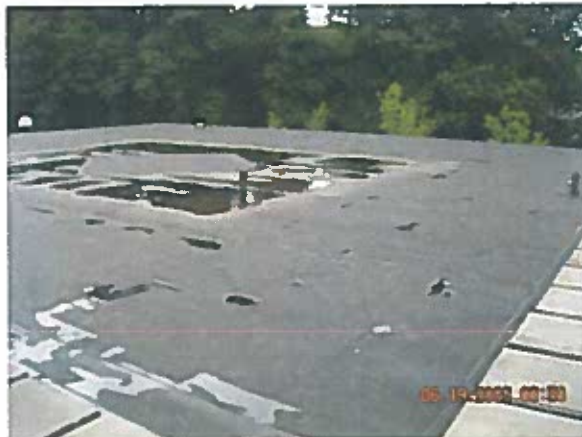
Area 11 — Overview NOTE: Excessive ponding was observed
