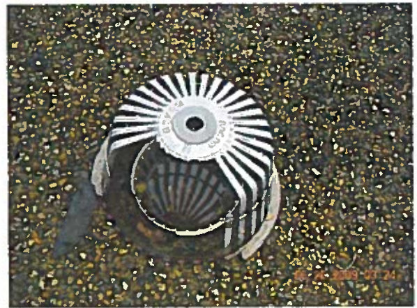
Area 3—Anomaly Broken drain strainer
