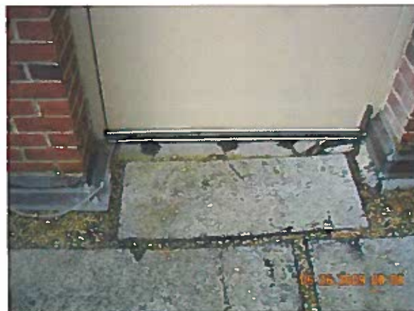
Area 1—Anomaly Low flashing height with topical repairs
