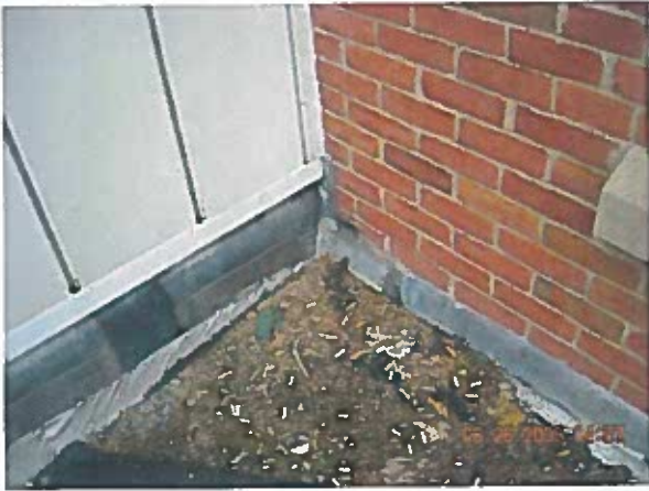
Area 21— Anomaly Poor expansion joint tie-in at wall
