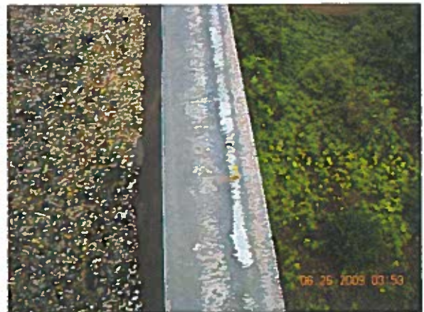
Area 9 — Anomaly Physical damage was observed at the metal coping
