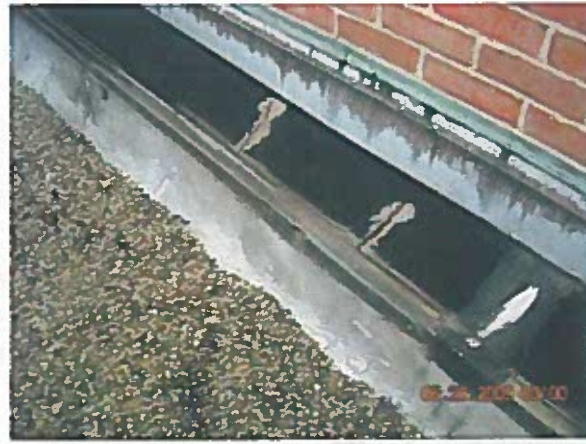
Area 4 — Anomaly Expansion joint is deteriorated
