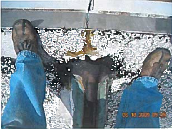
Area 13 — Anomaly Expansion joint does not extend to the outside edge
