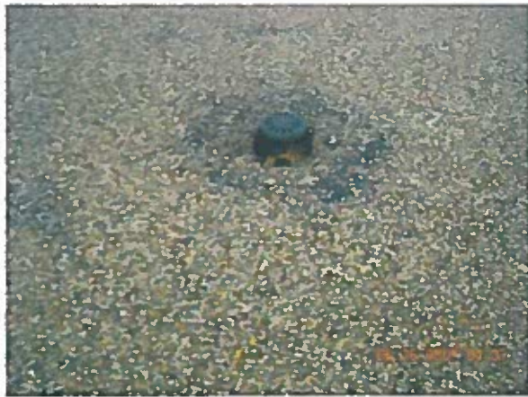
Area 18 — Anomaly Exposed membrane was observed around roof drain areas
