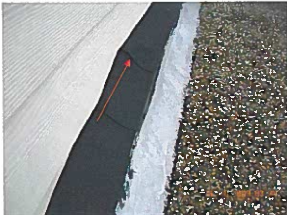
Area 3—Anomaly Open expansion joint laps
