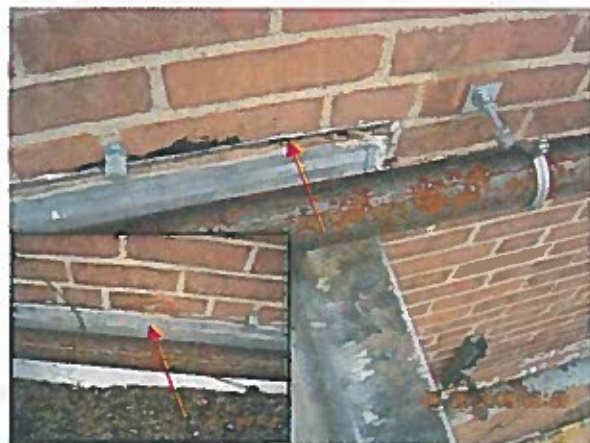
Area 2—Anomaly Missing sealant at counter flashing reglet
