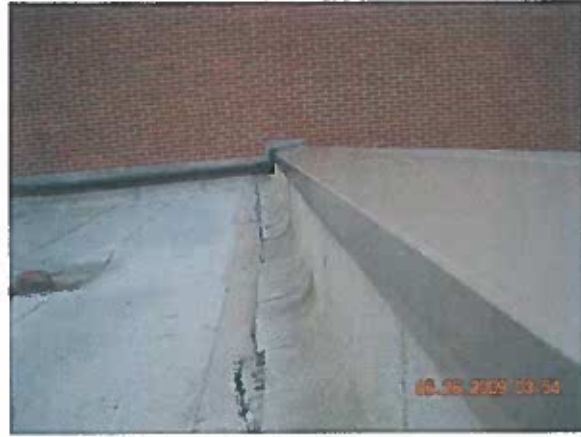
Area 9a — Overview / Observation Membrane has many wrinkles in the sheet
