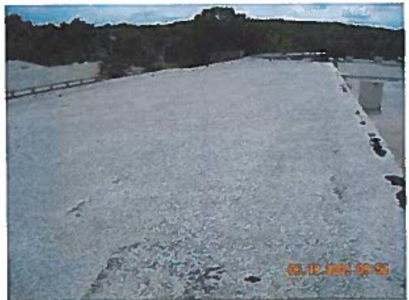
Area 12 — Overview NOTE: Exposed membrane along perimeter edge
