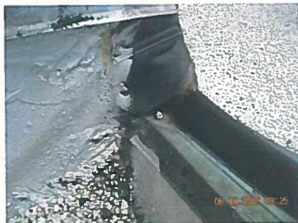
Area 13 — Anomaly Poor expansion joint tie-in
