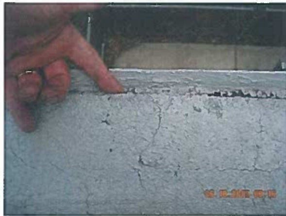
Area 1— Anomaly Strip-in flashings were un-adhered to the edge metal in many location. Where identified, remedial repairs were conducted to these locations
