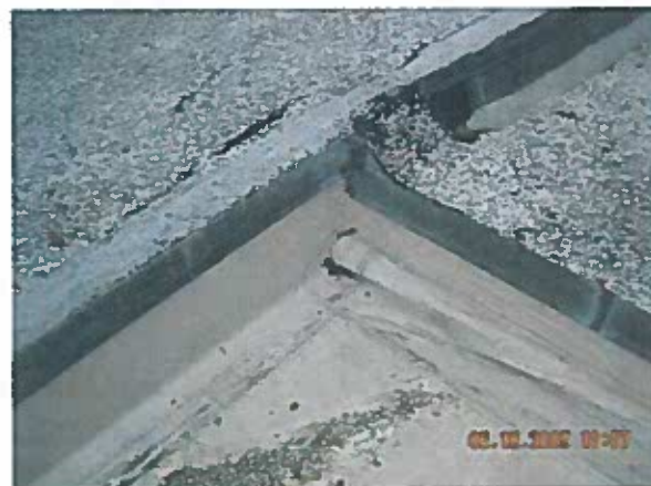
Area 19 — Anomaly Expansion joint does not extend to the roof's perimeter edge
