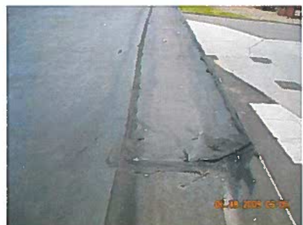
Area 1—Anomaly Metal edge strip-in delaminating from gravel guard
