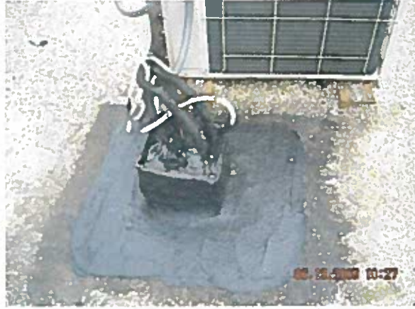
Area 16 — Observation Plastic coated conduits require a gooseneck chase
