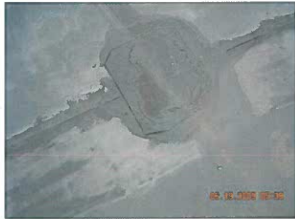
Area 11—Anomaly Surface splices are delaminating in many areas
