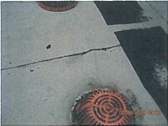
Area 5b — Anomaly View of wrinkle in sheet between roof drains
