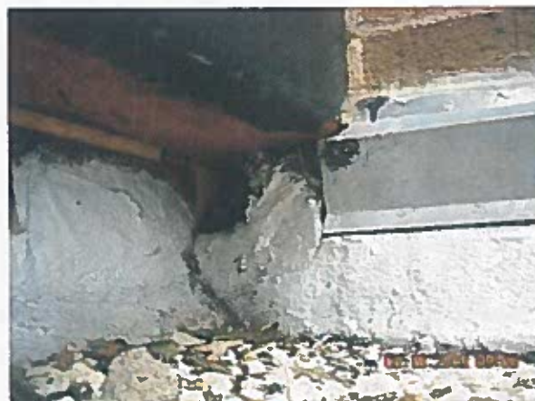
Area 11 — Anomaly Apparent opening below window
