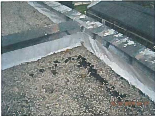
Area 13 — Anomaly Base flashings loose at inside corner
