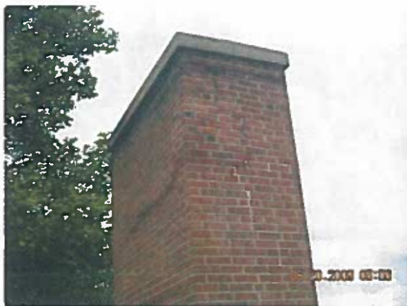
Area 2—Observation Mortar joints on brick work failing
