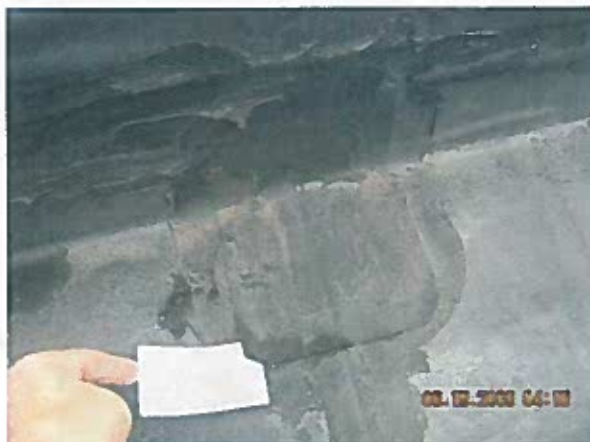
Area 5— Anomaly Splice patches delaminating at edges
