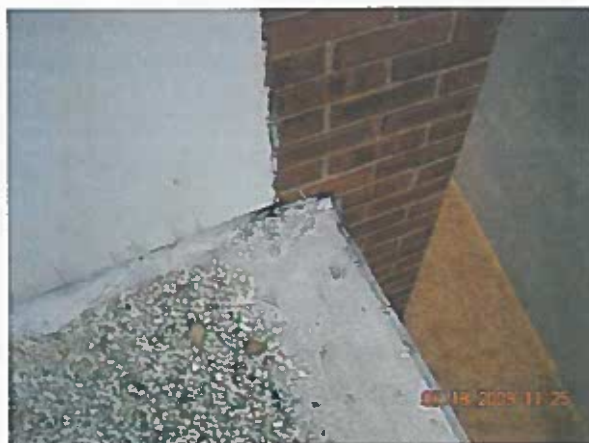
Area 7 — Anomaly Poor edge metal termination
