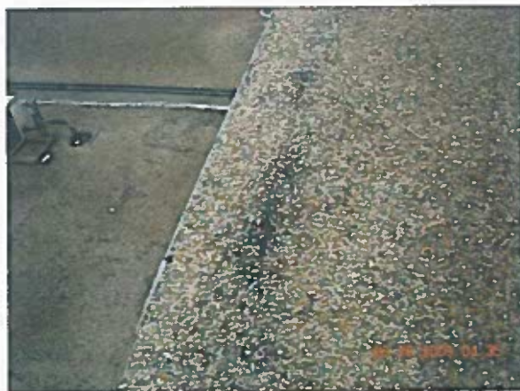
Area 16 — Anomaly Exposed membrane at some areas around the perimeter
