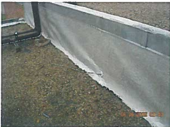
Area 2—Anomaly Apparent loose base flashings
