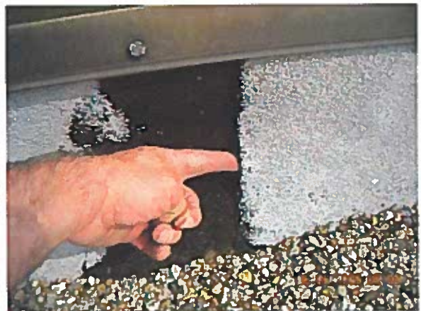
Area 6b — Anomaly Some voids in the flashing laps were identified
