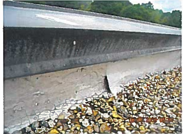
Gymnasium Area 4— Anomaly View of open base flashing along outside wall
