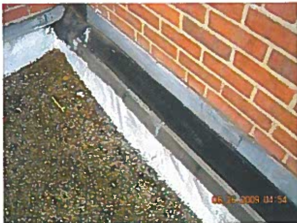
Area 19 — Anomaly Expansion joint cover is deteriorated
