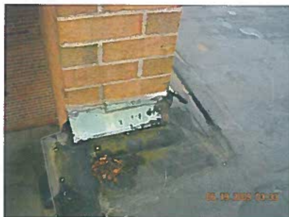
Area 2—Anomaly Metal counter flashing in poor condition
