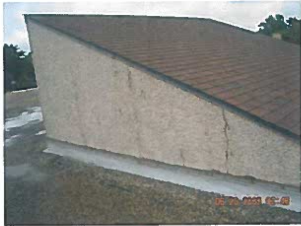
Area 4—Anomaly Cracked cementitious board on skylight
