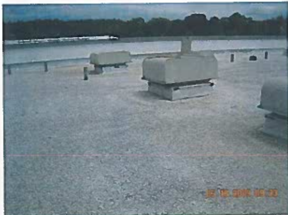
Area 13 —Observations Terminations appear to be in satisfactory condition. Gutters were cleared of debris
