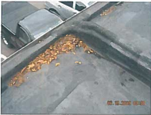
Area 2—Overview View of expansion joint at roof transition at roof edge Debris was removed from the roof's surface
