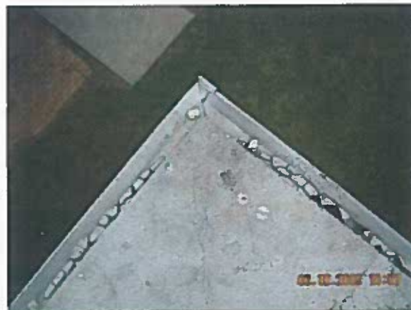
Area 5 — Anomaly Strip-in membrane delaminating from edge metal
