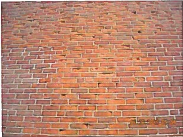
Area 6a — Observation Brick work deteriorating from moisture intrusion
