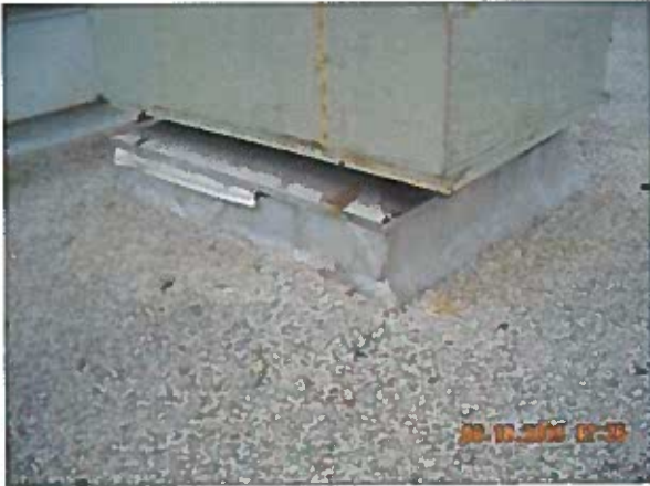
Area 7 — Anomaly Loose base flashings around ventilators
