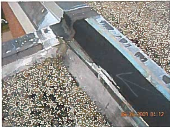
Area 12 — Anomaly Expansion joint damage
