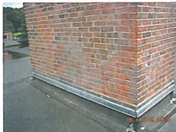
Area 6 — Anomaly Brick tuck-pointing recommended
