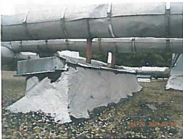
Area 4—Anomaly Damaged curb flashing a support stand
