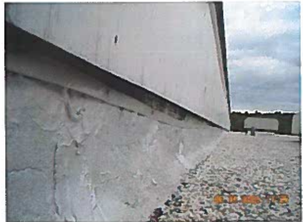
Area 7 — Anomalies Open termination at base flashings NOTE: Base flashings appear to be in poor condition
