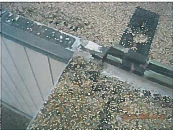
Area 18 — Anomaly Expansion joint did not extend correctly to roof edge causing split in membrane
