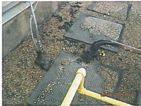
Area 6a — Anomaly Pipe penetration pockets are clustered with deteriorated fillers (typical)
