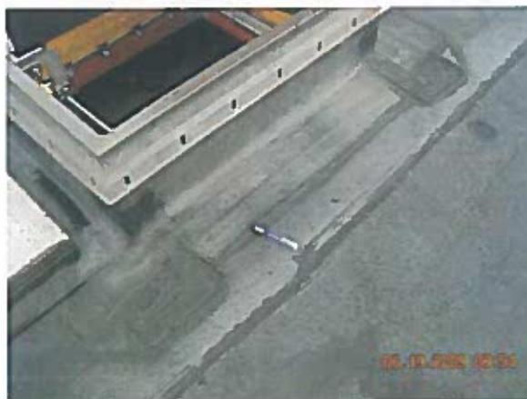
Area 11 — Anomalies Splice patches at edge metal transitions are delaminating and splice patches in the field of the roof are delaminating
