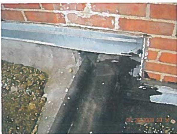
Area 8 — Anomaly Open terminations were observed along with open inside corners on sheet metal work
