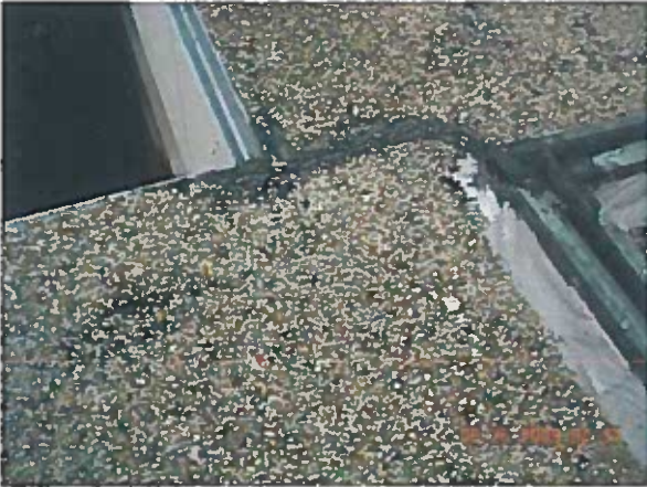
Area — Anomaly Expansion joint did not extend to roof edge causing split in membrane
