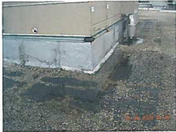
Area 13 — Observation Ponding water at base of A/C unit
