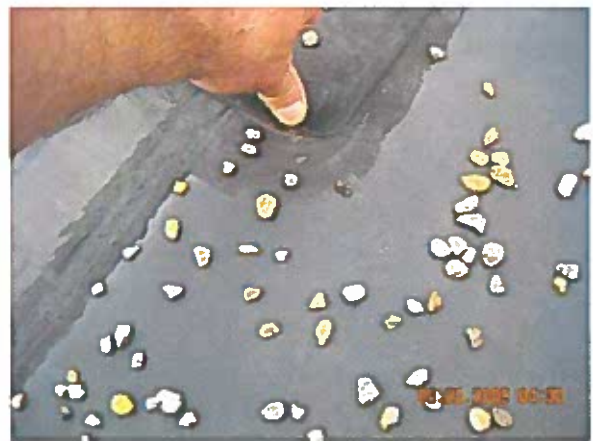
Area 5—Anomaly Splice patches delaminating from membrane
