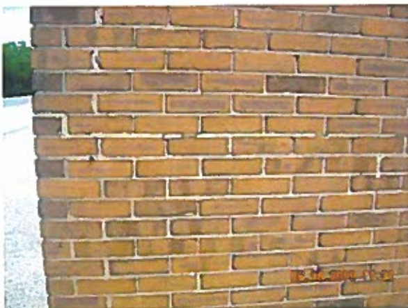
Area 7 — Anomaly Mortar beds for brick in poor condition
