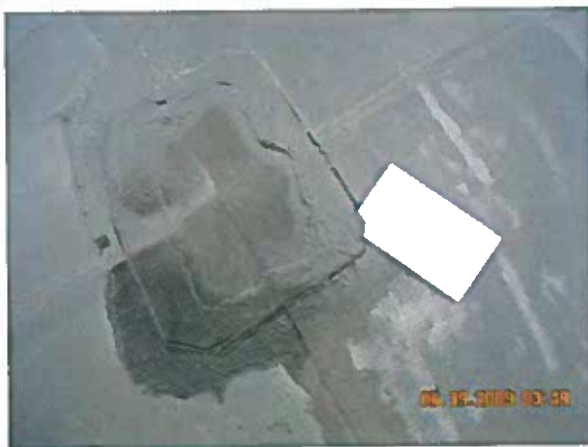
Area 3—Anomaly Splice patches delaminating in many areas
