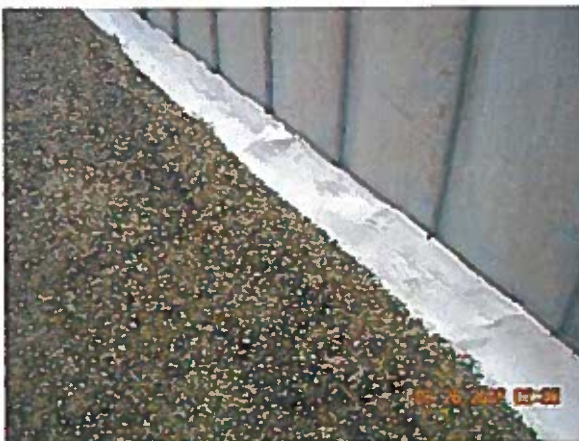
Area 1— Anomaly Apparent loose base flashings
