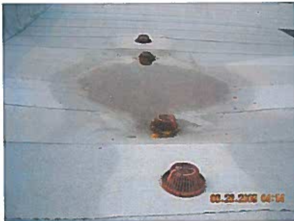
Area 9b — Anomaly Appears cricket was not installed during the installation
