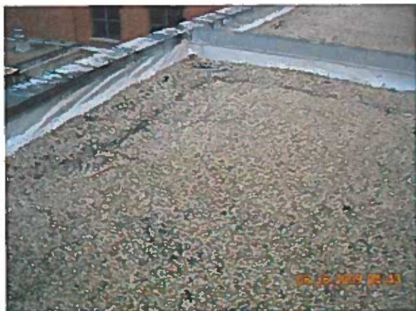
Area 25—Anomaly Base flashings are loose at perimeter wall
