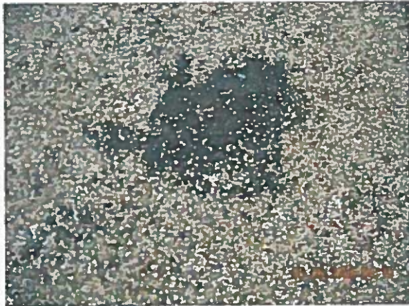
Area 11 — Anomaly Several areas of exposed membrane
