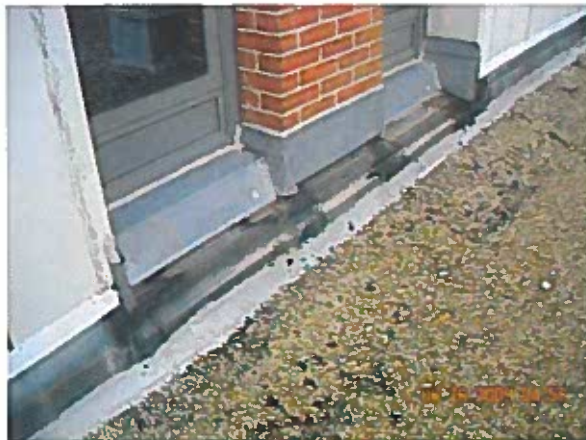
Area 21— Anomaly Several open cover strips at window area
