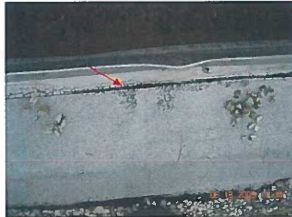
Area 8 — Anomaly Strip-in delaminating from edge metal Remedial repairs conducted to these areas
