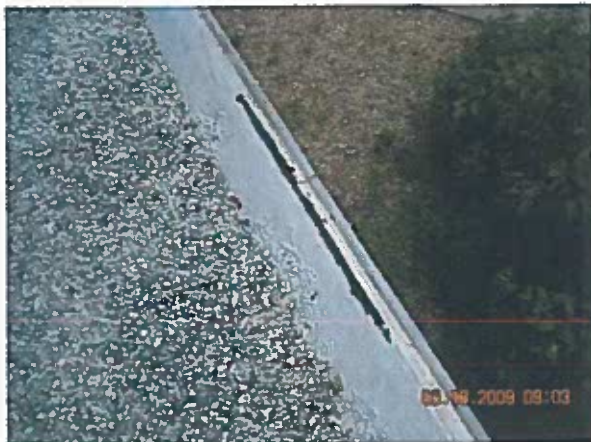
Area 11 — Anomaly Remedial repairs were conducted to the strip-in at locations delaminated from edge metal
