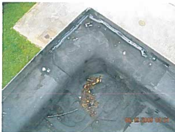
Area 1—Anomaly Open splice along outside edge was sealed
