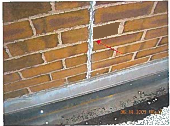
Area 3 — Anomaly Deteriorated sealant joints were observed
