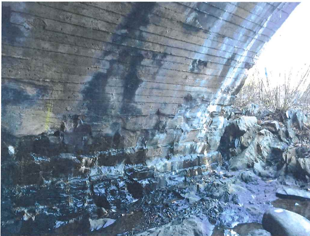
Image 4: Northwest corner of bridge arch. The original masonry is visible at the base of the arch where the board-formed concrete coating has eroded over time.
