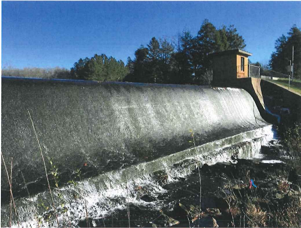
Image 5: This “ogee” dam is named for the S-shaped profile of its spillway. It was constructed in 1909-1911 to create the Wepawaug Reservoir and provide water to New Haven.
