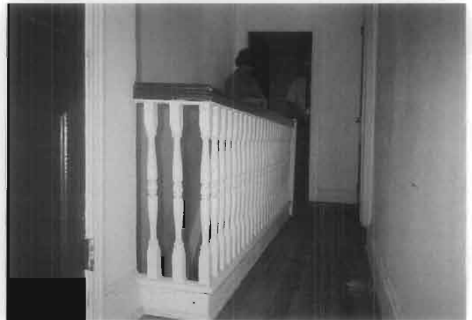
Figure 28. This recently completed housing, which is now lead-safe, could become re-contaminated from lead if safe conditions are not maintained. Damp mopping floor surfaces and regular dusting to keep the house clean will ensure its continuing safety.
