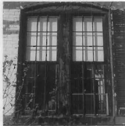
Figure 6. Deteriorating operable windows often contribute to lead dust in a house. Peeling paint and small particles from abraded surfaces collect in window troughs or sills and are then carried inside by air currents, settling on floors. When the lead dust mixes with regular house dust, it can easily be ingested by a child through hand to mouth contact. In homes with small children, floors and other surfaces should be kept as clean as possible to avoid lead contamination.
