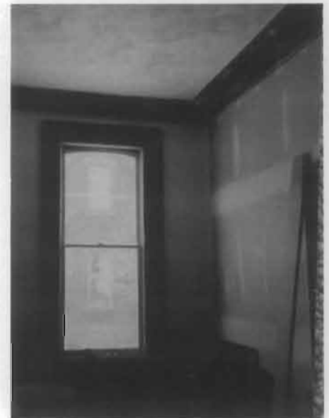
Figure 25. In some cases, skim coating deteriorated plaster and repainting is adequate. If the plaster is seriously damaged or failing, drywall may be considered so long as the molding and window reveal relationships are retained. In this case, plaster between the windows was repaired and repainted and the side wall plaster was replaced with drywall. Photo: Landmarks Design Associates.
