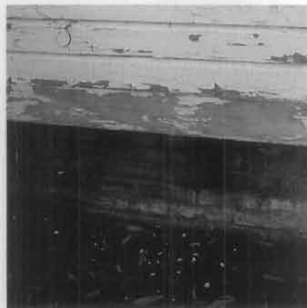
Figure 7. Chalking exterior paint can cause dangerous lead levels in soil around a house. Lead levels are usually highest in the one foot wide area adjacent to the building foundation. In these cases, the existing soil should be replaced with new soil or sod. This is particularly important if children and small pets play in contaminated areas, then inadvertently track the dirt inside.
