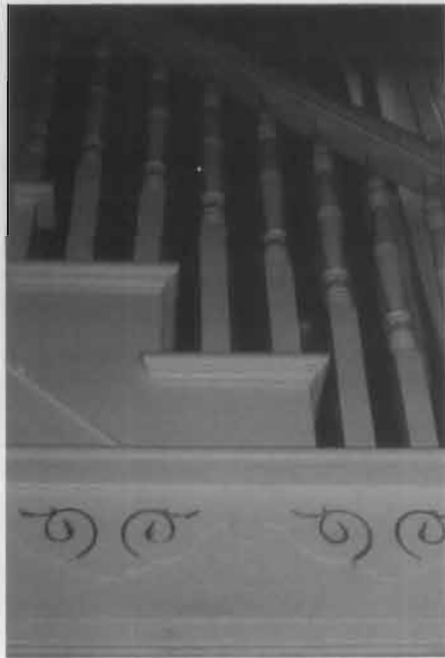
Figure 23. Stair banisters and railings are considered mouthable surfaces. In this case, the old paint was wet sanded to a sound layer. Special encapsulant paints were then applied in three thin layers to avoid obscuring the woodwork's fine detailing. It should be noted that many encapsulant paints are now treated with a bitter agent to discourage mouth contact. Photo: Landmarks Design Associates.
