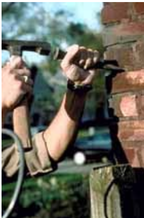
Here, a hammer and chisel are being correctly used to prepare a joint for repointing. Photo: John P. Speweik.
