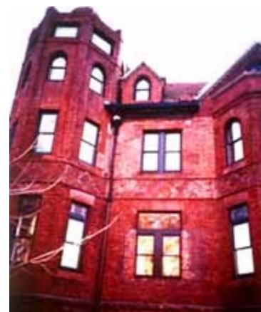
Unskilled repointing has
