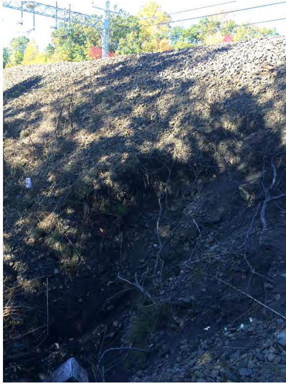
Downstream Embankment at culvert – note sloughing
