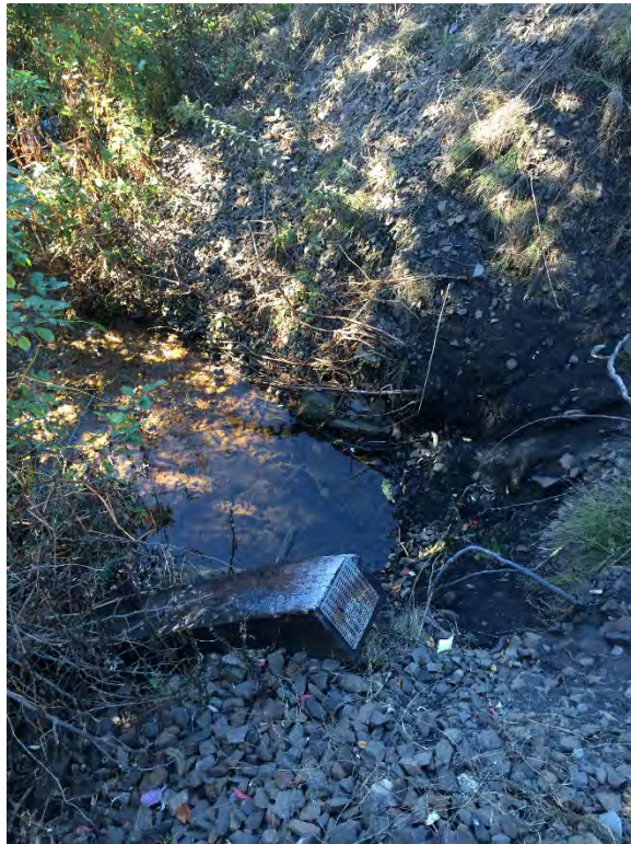
Downstream outlet – note collapsed structure
