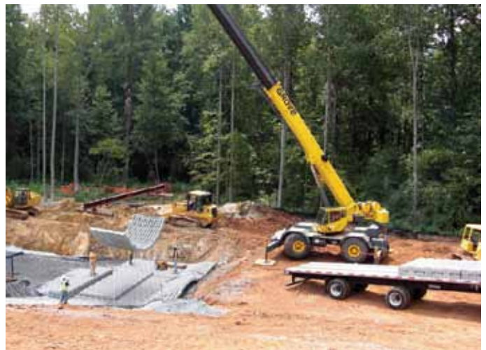
The use of a crane is optimal for fast and safe unloading and installation of the mats.
