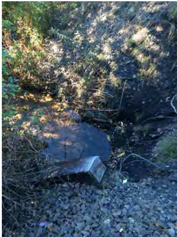
Downstream outlet – note collapsed structure
