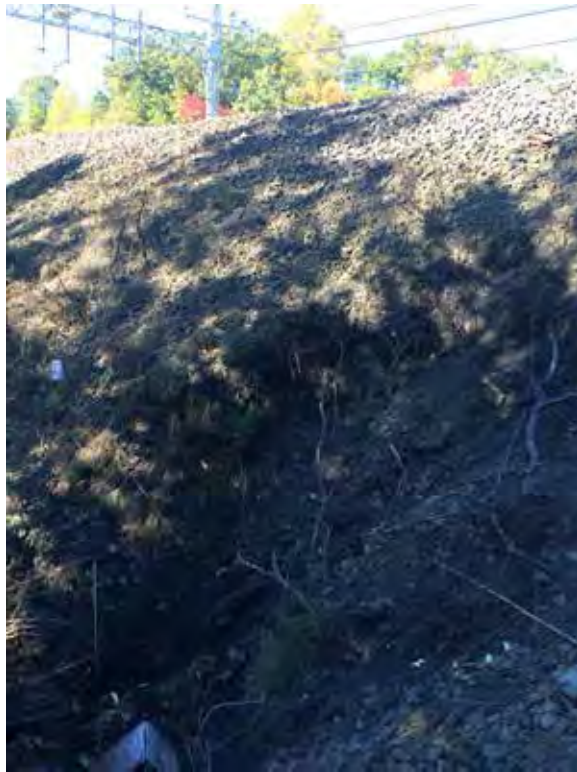
Downstream Embankment at culvert – note sloughing
