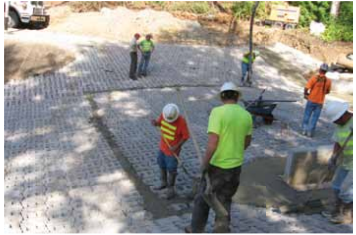
Grout to the top of the block or slightly lower — not above.
