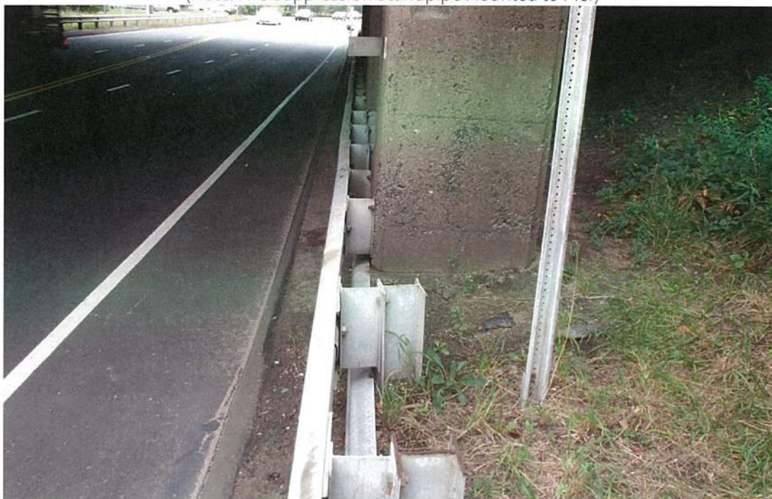
17. Lateral Clearances West Pier (Pier 1) North end (Note: This is location of minimum horizontal clearance)
