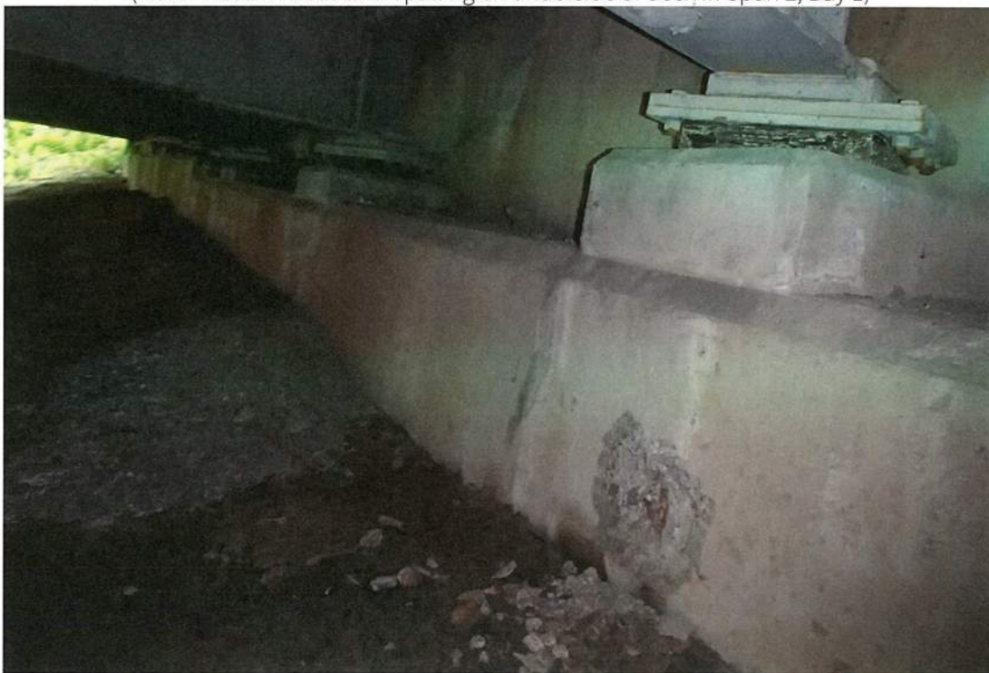
10. Looking South along West Abutment (Note: Spall on Abutment Face and Elastomeric Bearings supporting Beams)
