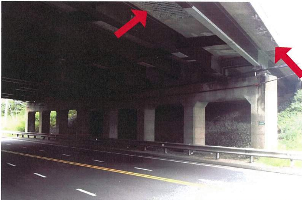
Image 2: Underside of deck and substructure of Bridge #00196, viewed from East Main Street. Note the concrete deterioration and exposed reinforcing bars of the deck (red arrows).
