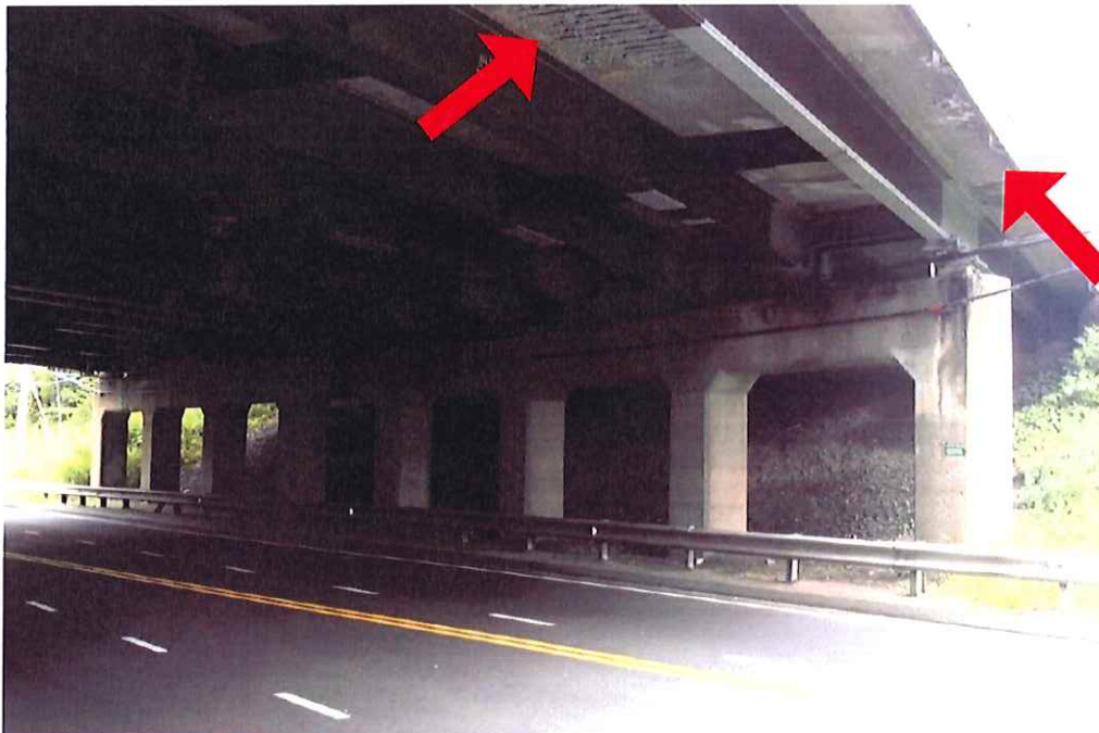
Image 2: Underside of deck and substructure of Bridge #00196, viewed from East Main Street. Note the concrete deterioration and exposed reinforcing bars of the deck (red arrows).
