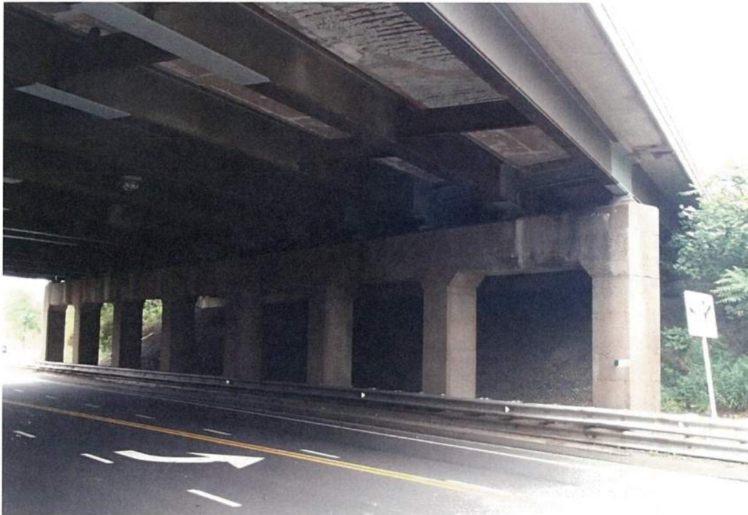
9. West Pier (Pier 1) East Elevation (Note: Hollow Areas and Spalling on underside of deck in Span 2, Bay 1)
