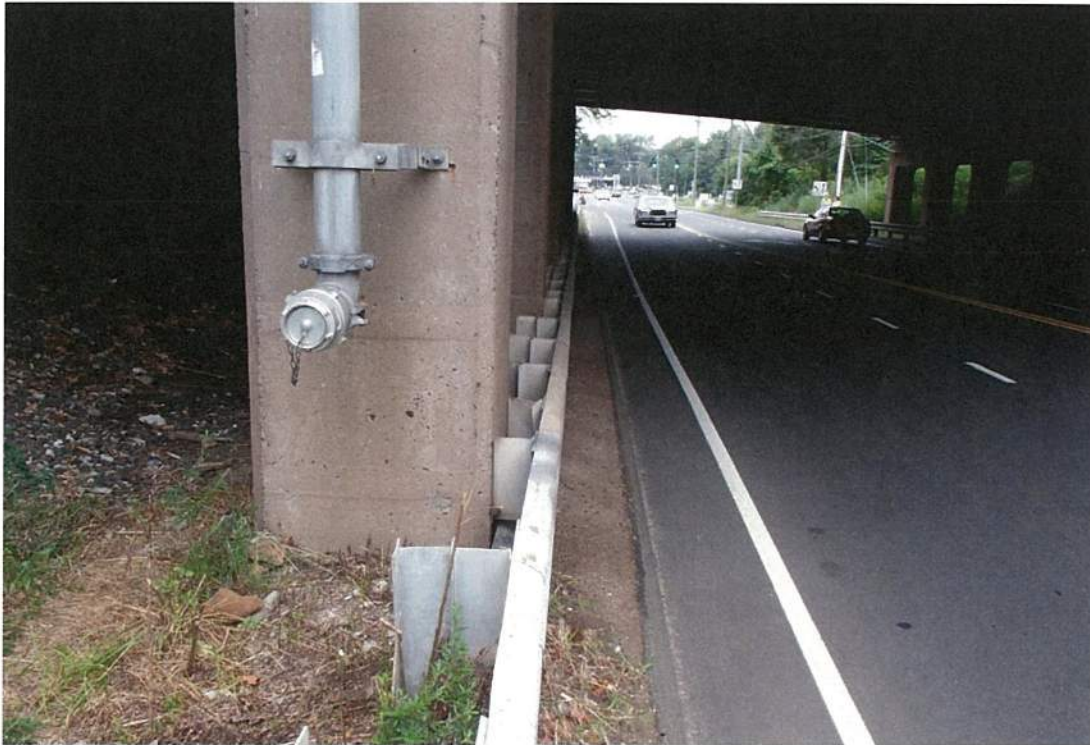
16. Lateral Clearances West Pier (Pier 1) South end (Note: Fire Suppression Standpipe Mounted to Pier)
