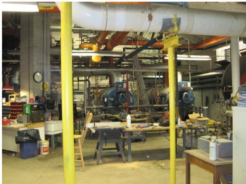
Figure 5: CT Boiler House Interior (Looking at Existing Auxiliary Boilers)
