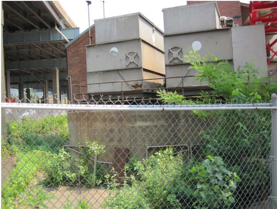
Figure 7: Retired-In-Place Cooling Towers and Associated Platform
