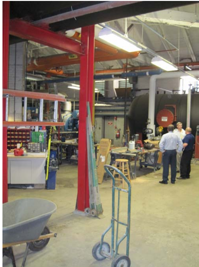
Figure 6: CT Boiler House Interior (Looking at Existing Chilled Water Expansion/Surge Tank)
