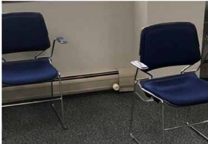
Existing Perimeter Finned Tube
