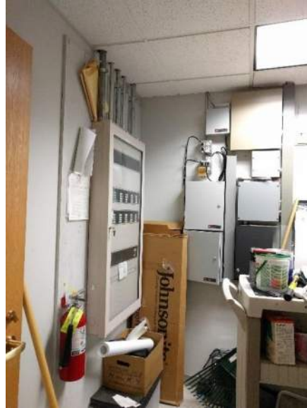
Existing Fire Alarm Control Panel
