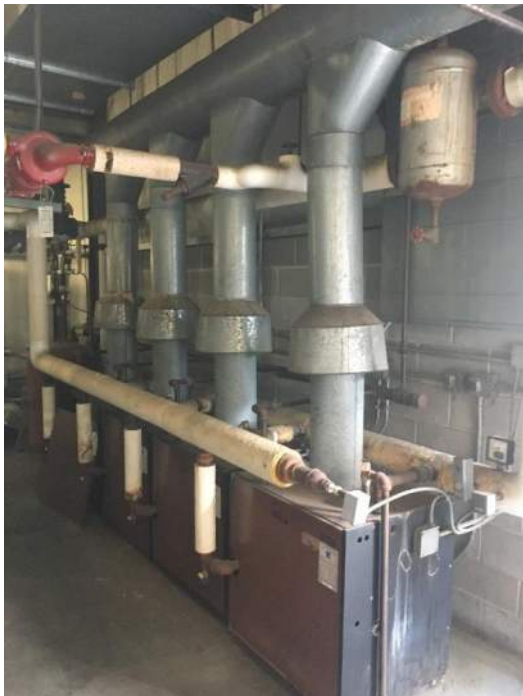
Existing Boiler Plant in Penthouse MER
