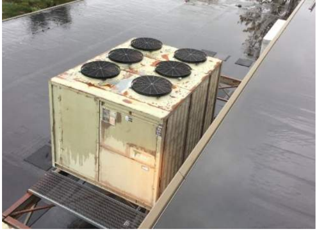
Existing ACCU-2 Serving Indoor Air Handler AC-2
