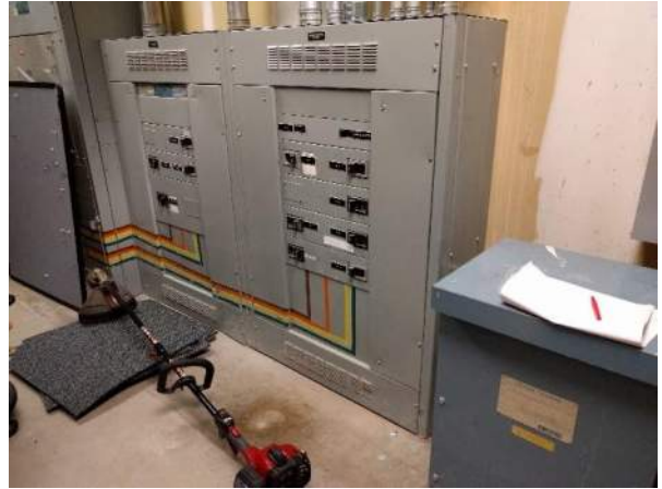
Existing First Floor Electrical Room
