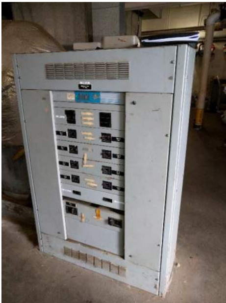
Existing Penthouse Electrical Equipment
