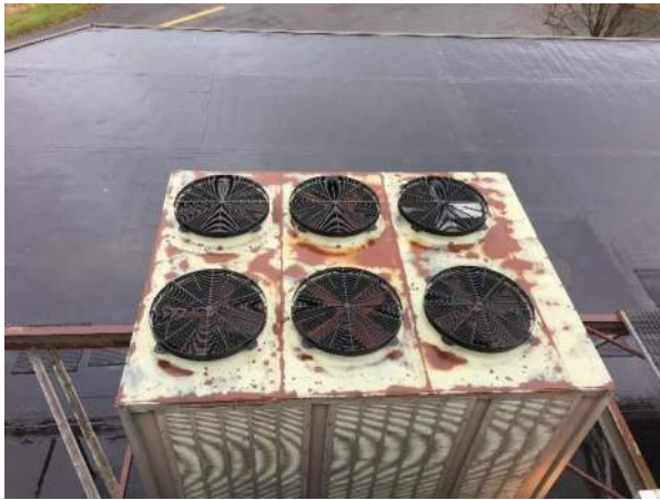
Existing ACCU-1 Serving Indoor Air Handler AC-1
