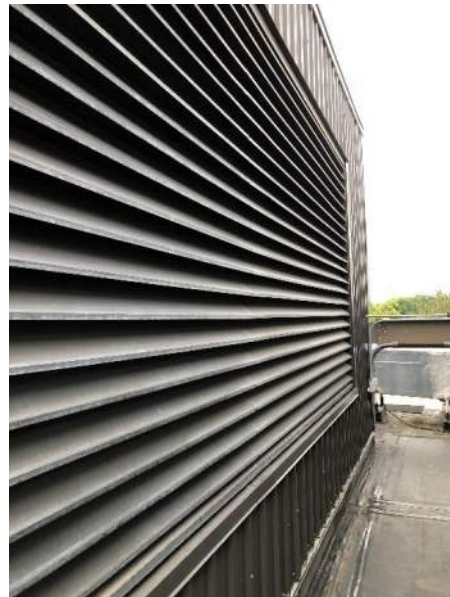
Existing Louver Serving AC-1 & AC-2
