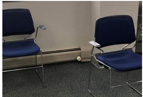
Existing Perimeter Finned Tube
