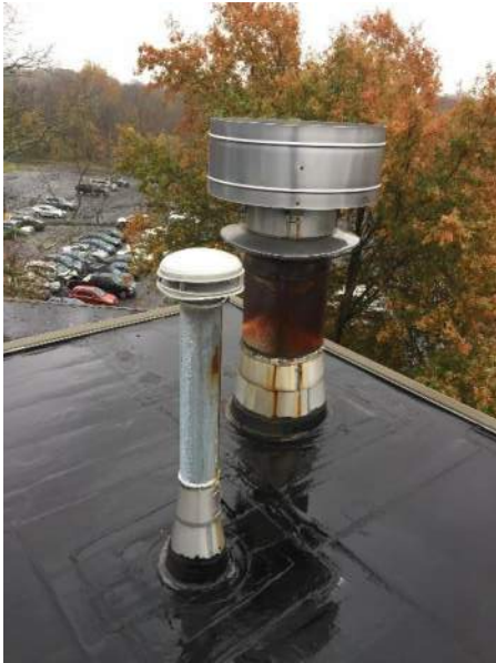
Existing Boiler Flue & UH Flue Termination
