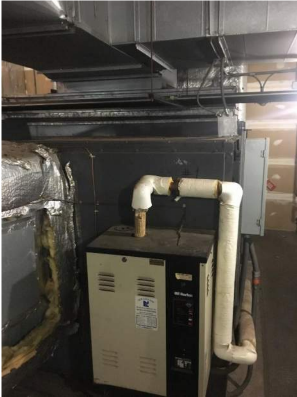
Existing Indoor AHU-1 in Penthouse MER
