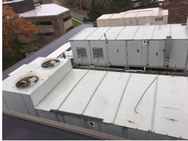
Existing RTU-3 & RTU-4
