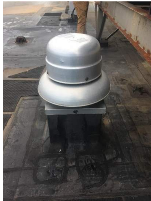
Existing Rooftop Exhaust Fan. Typical.
