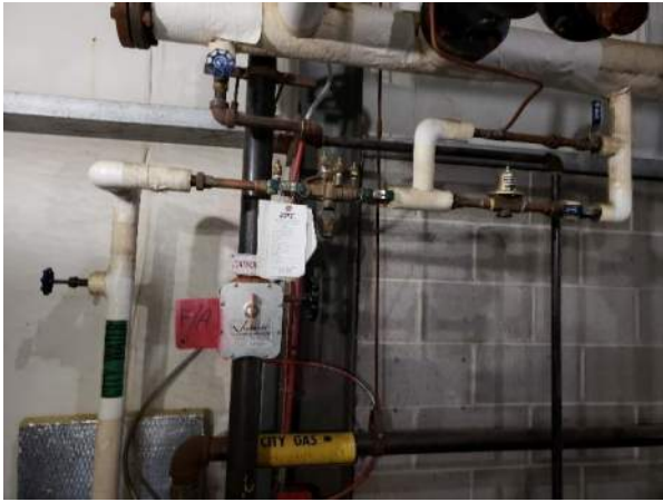
Existing Domestic Water & Gas Piping in Penthouse MER
