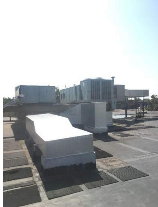
Existing Rooftop Units RTU-3 & RTU-4 & Associated Roof Mounted Ductwork
