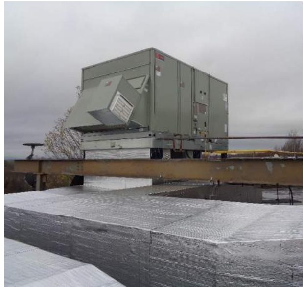
Recently Replaced RTU-5
