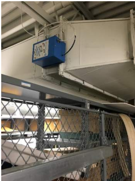
Existing Pressure Independent Module
