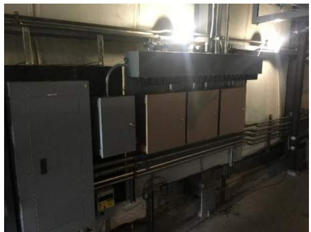
Existing BMS Controllers in BMS Penthouse
