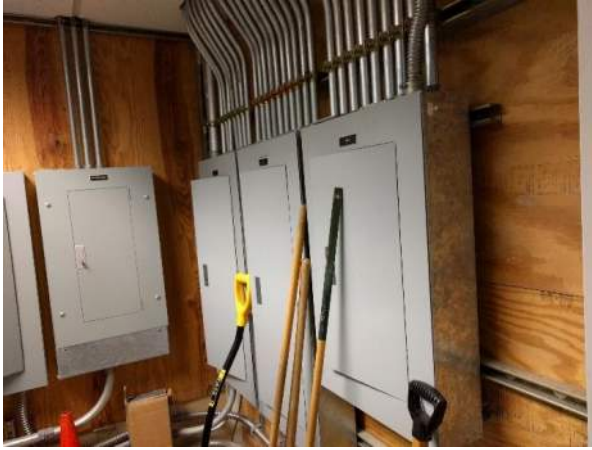
Existing First Floor Electrical Room
