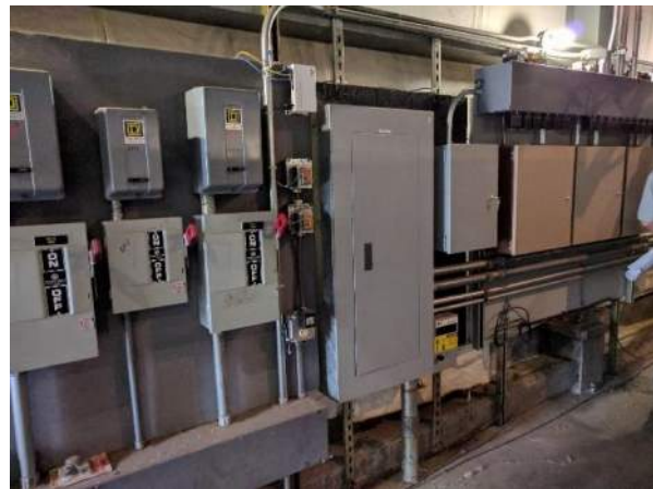
Existing Penthouse Electrical Equipment
