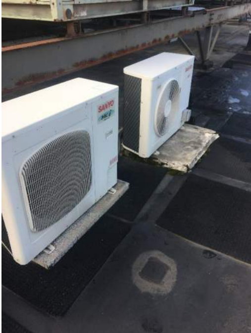
Existing Split A/C Condensing Units on Roof
