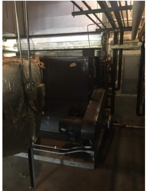
Existing Indoor AHU-2 in Penthouse MER
