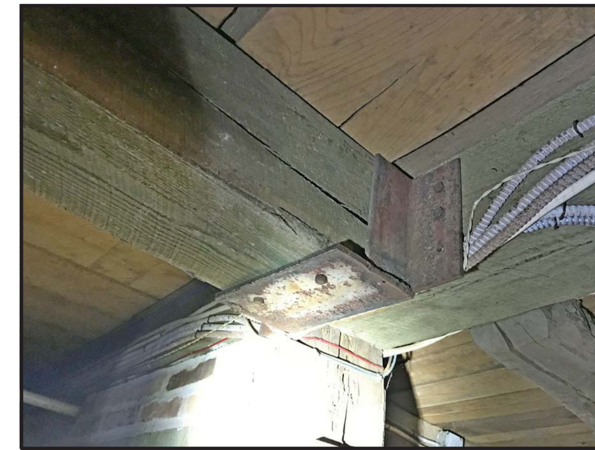
P04 WIRE BRUSH CLEAN EXISTING HANGER AND INSTALL (N) LAG SCREWS IN EMPTY HOLES. REMOVE AND REINSTALL WIRING AS NEEDED.
