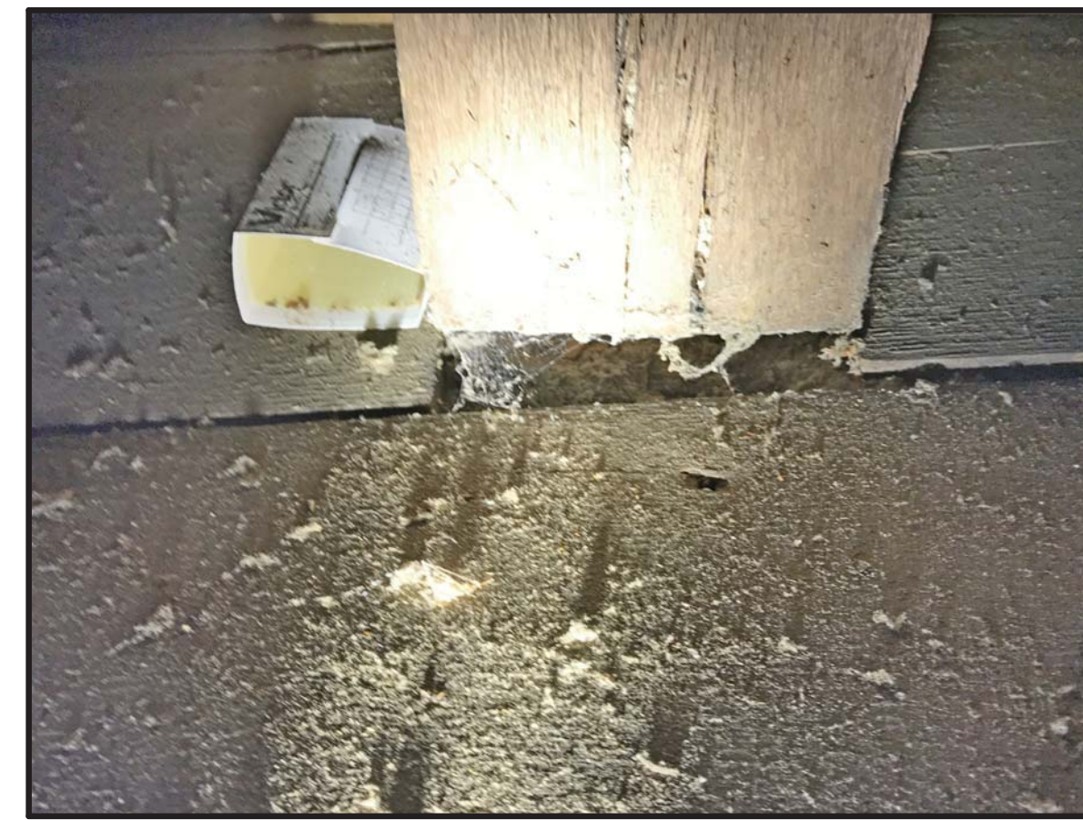
P08 SHIM POSTS IN ATTIC TIGHT TO ATTIC FLOOR FRAMING
