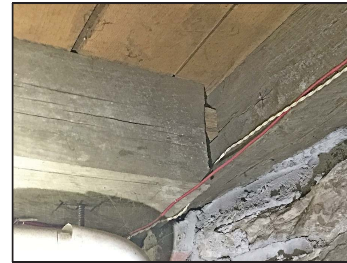
P07 ALL GIRDER END CONNECTIONS TO BE REINFORCED WITH NEW STEEL ANGLES.
