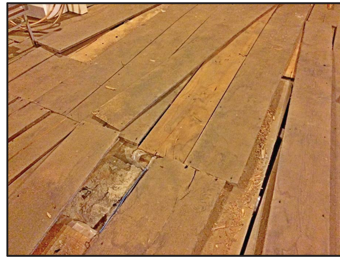
P09 LOOSE FLOOR BOARDS TO BE SHIMMED AND REATTACHED.
