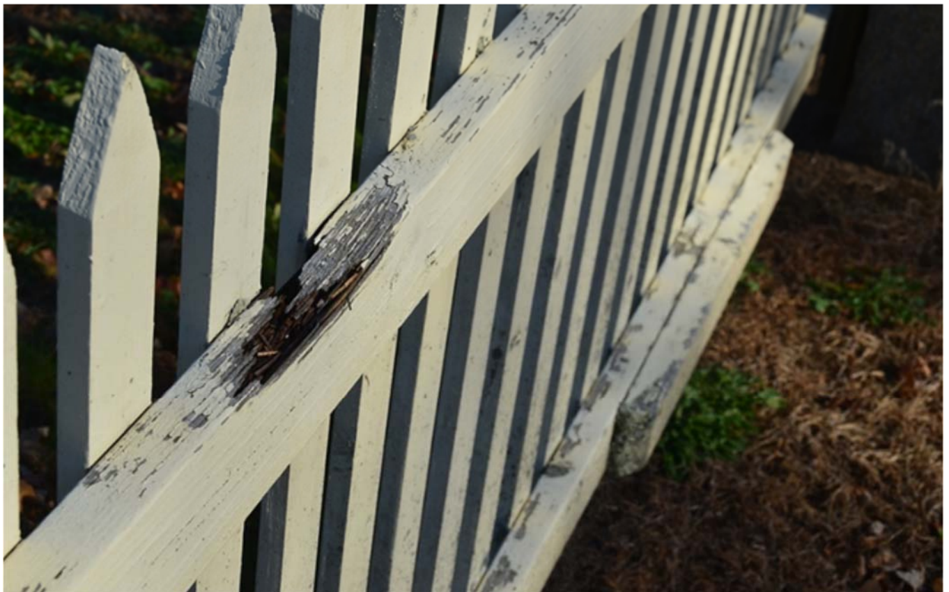
PHOTO 63 Open joints, splice, and isolated rot. Replacement may be less costly.
