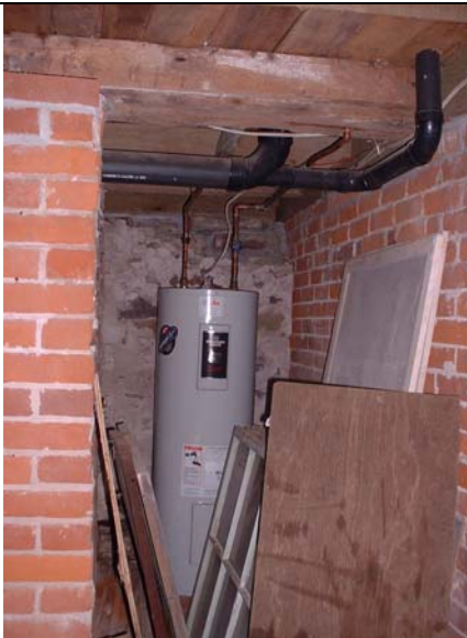
Photo C-1-3: Electric hot water heater
