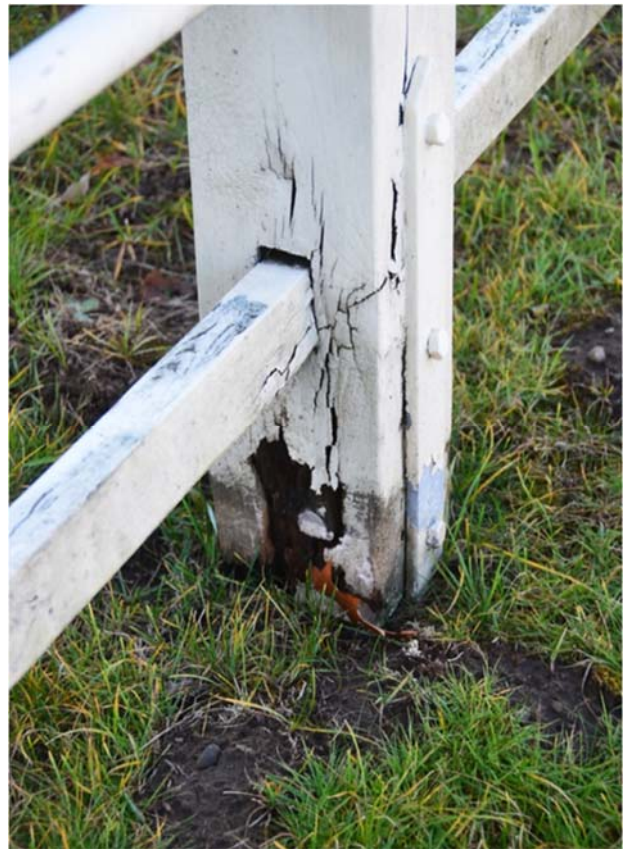
PHOTO 71 Rotted post bases.
