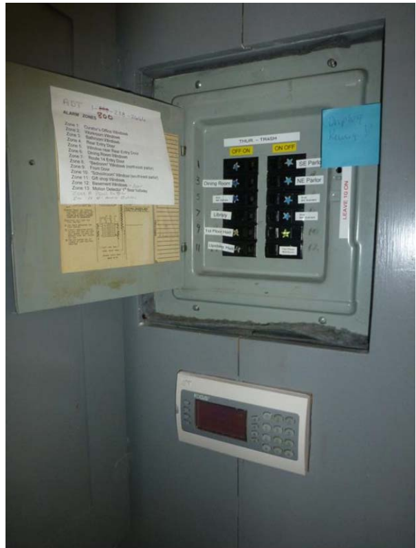
Photo C-2-17: Circuit breaker panel on 1st floor used as switch box.
