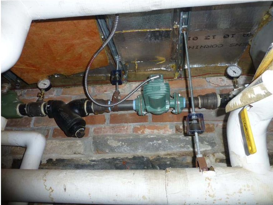
Photo C-2-7: Hot water pump
