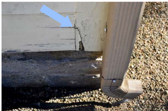
PHOTO 22 Dry cracks in trim.
