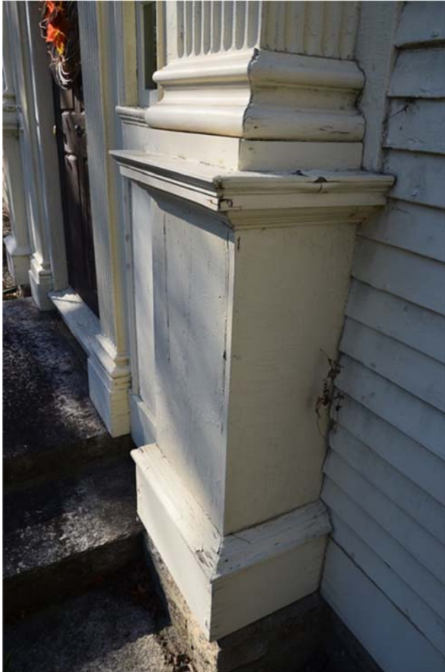
PHOTO 27 Engaged columns at E. Entry take on a roof-ful of rainwater.
