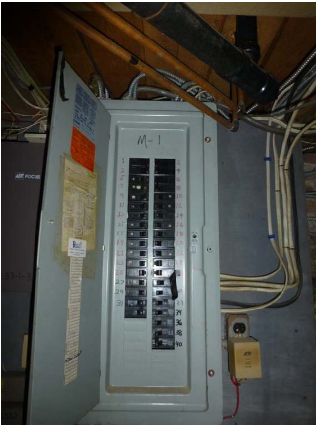
Photo C-2-9: Main Electric Panel
