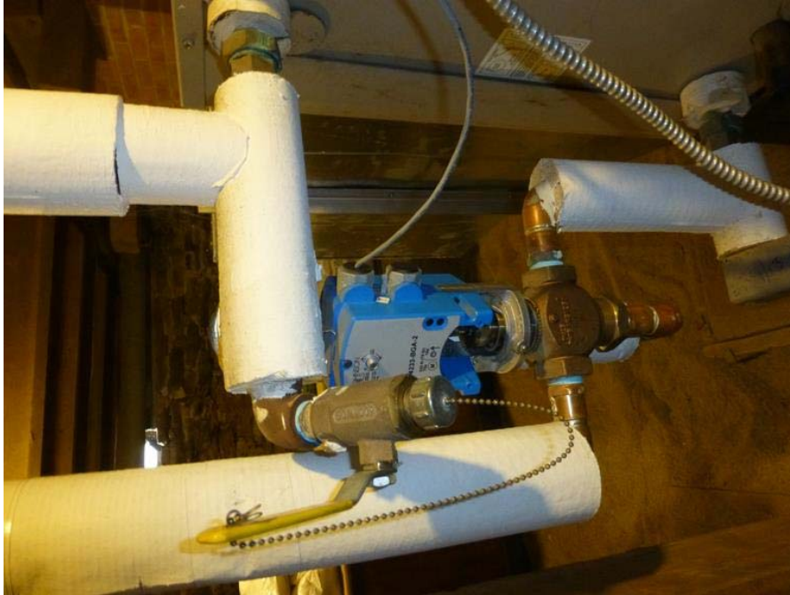
Photo C-2-3: Control valve for AHU-1
