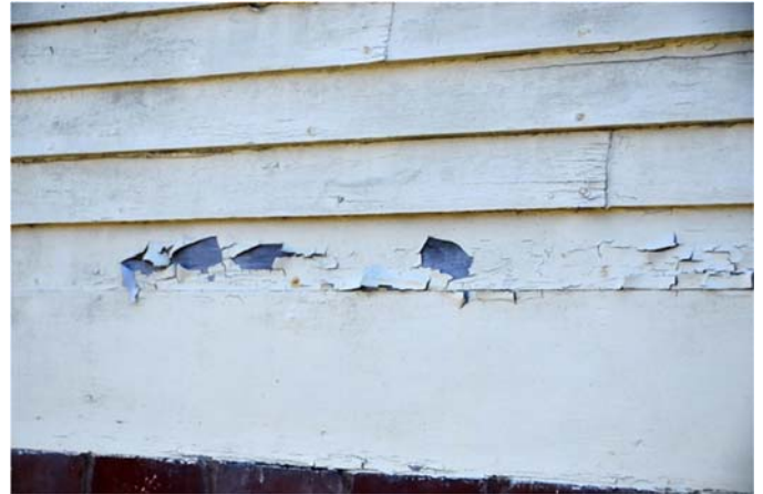
PHOTO 13 No flashing behind clap above skirt.
