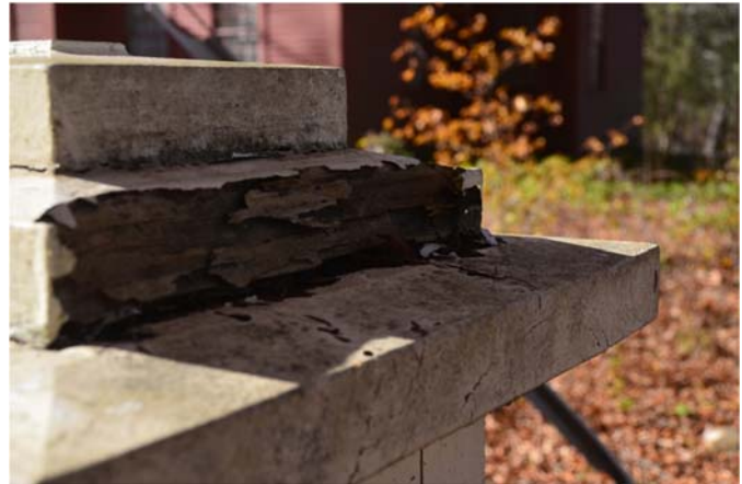
PHOTO 65 Rotted solid post caps.
