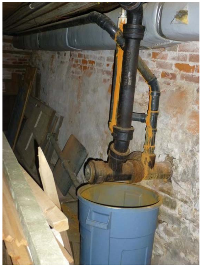
Photo C-2-10: Main Sanitary waste line
