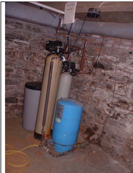
Photo C-1-7: Pressure tank and water softener
