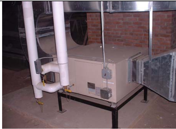
Photo C-1-4: Air handler serving the Ell
