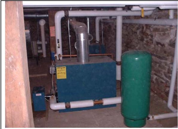
Photo C-1-1: Oil-fired hot water boilers in basement
