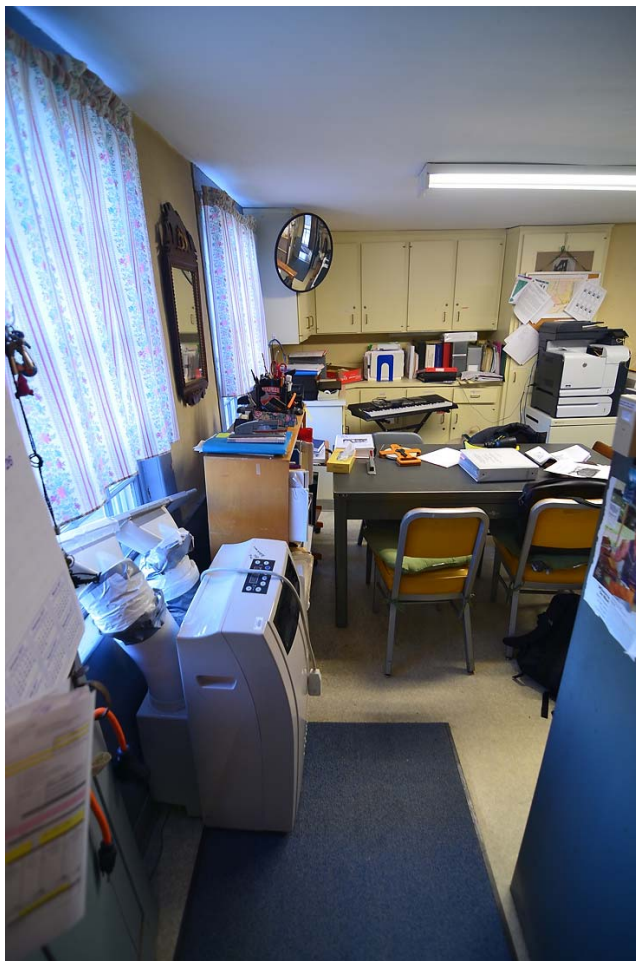
PHOTO 85 Portable air-conditioners are used.
