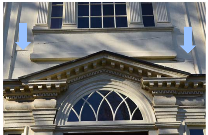
PHOTO 25 Water-damaged flat paneling in E. bay.
