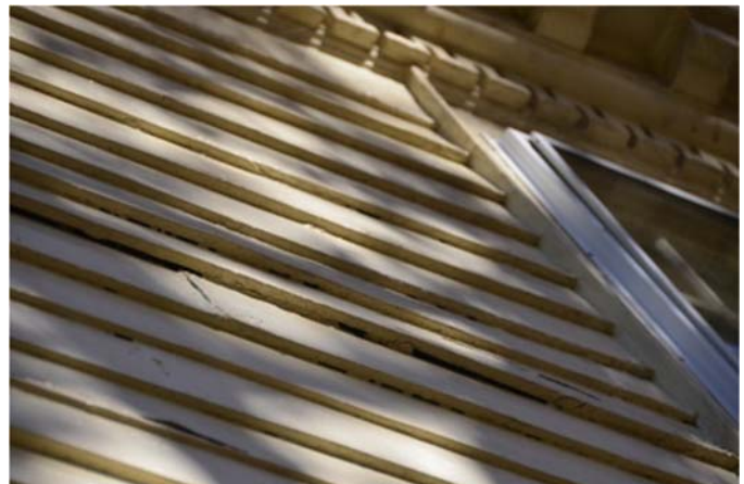
PHOTO 14 Open joints in clapboards.
