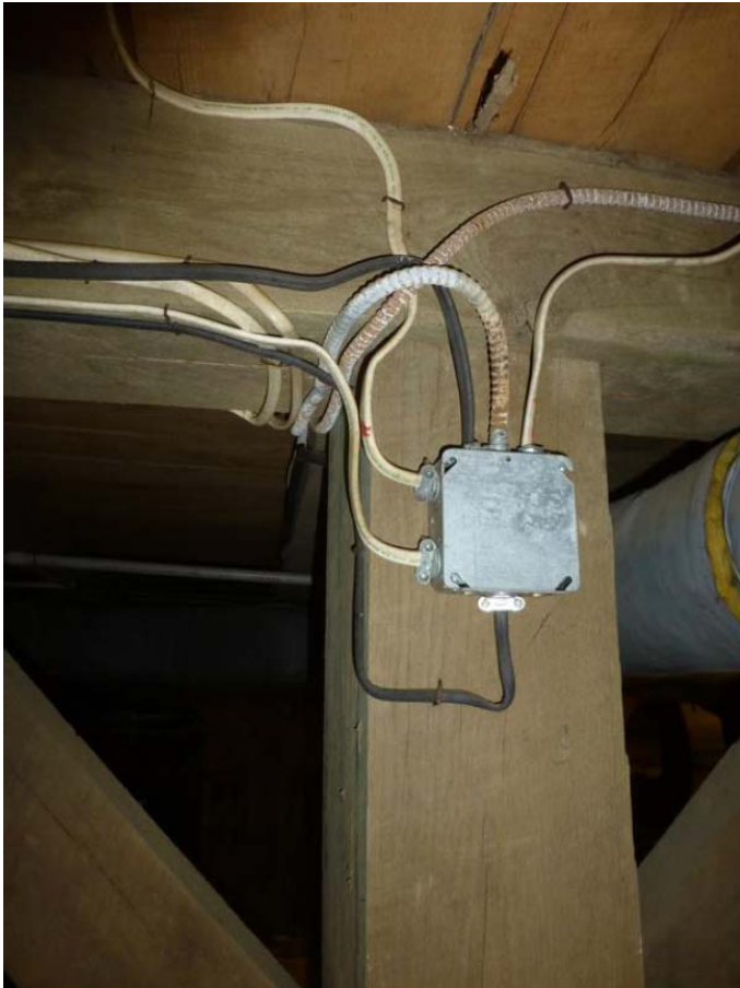
Photo C-2-12: Mixture of wiring types. Note corrosion on metallic sheathing
