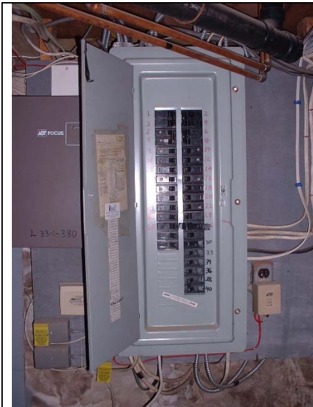
Photo C-1-5: Main electric panel
