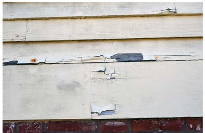
PHOTO 20 Moisture at top of skirt board.
