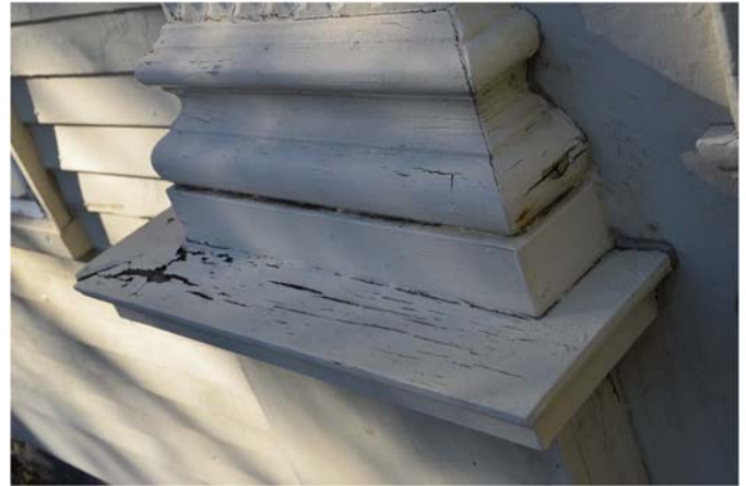
PHOTO 28 Rot at exposed trim, above and below.
