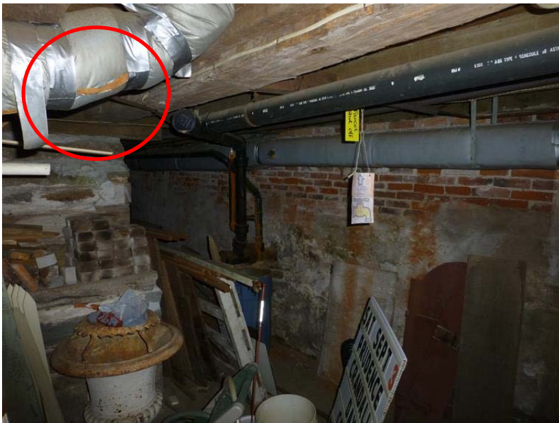
Photo C-2-8: Example of damaged vapor barrier on duct insulation
