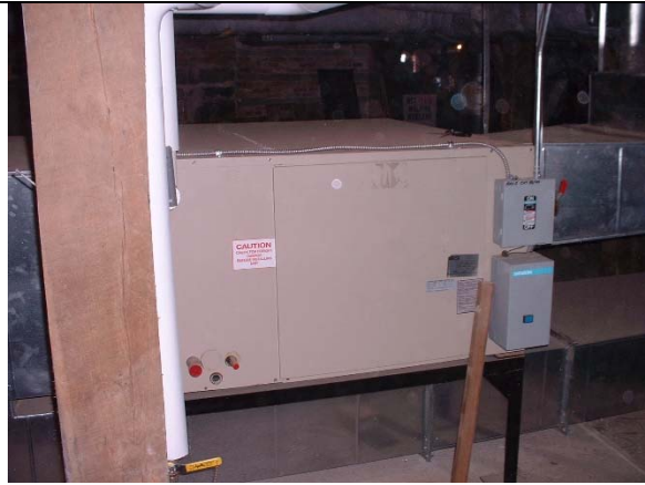
Photo C-1-2: Air handler serving the Main Block
