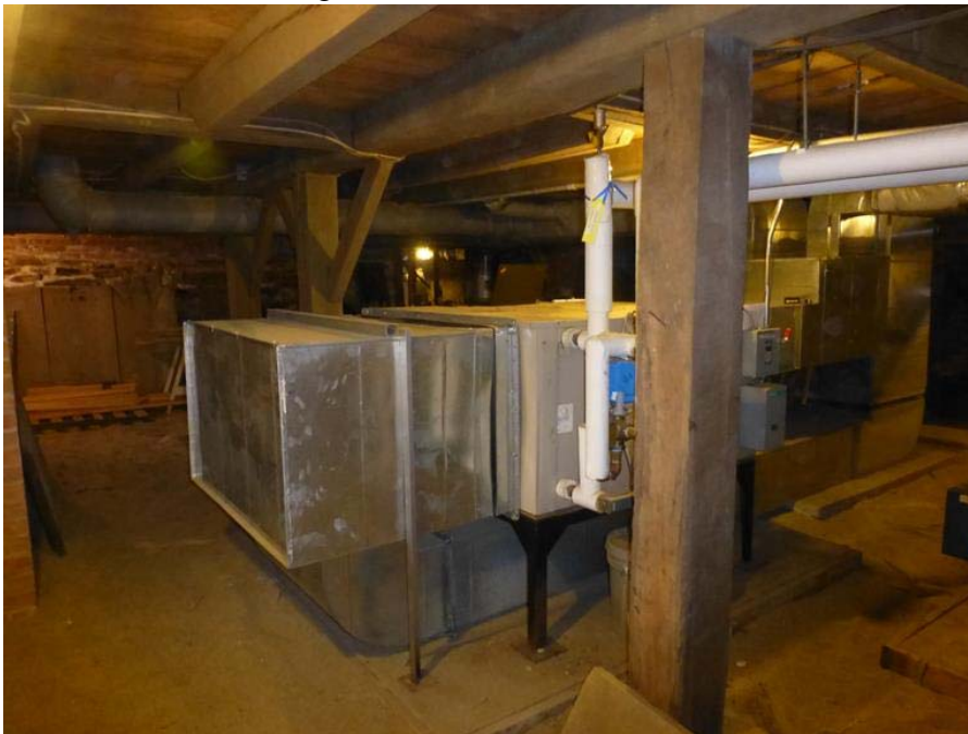
Photo C-2-2: Air Handler AHU-1
