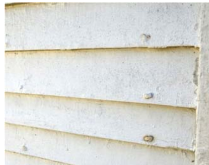
PHOTO 15 Exposed nail heads.
