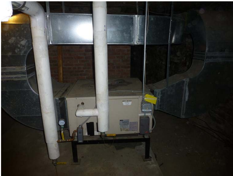
Photo C-2-6: Air Handler AHU-2
