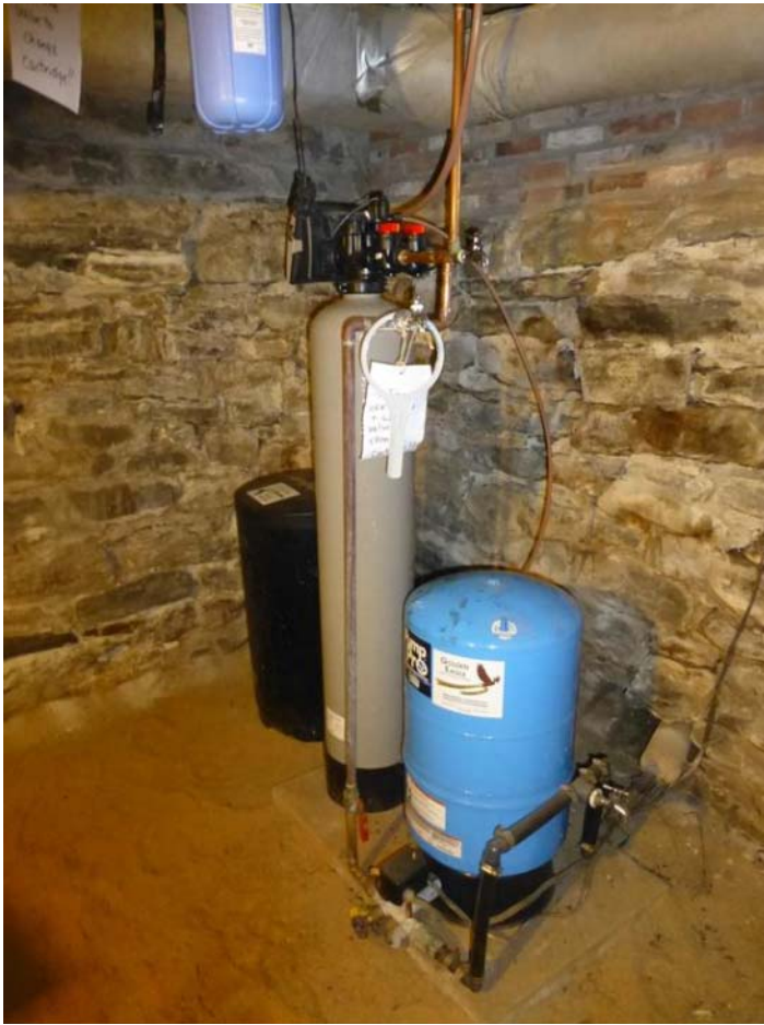
Photo C-2-1: Incoming water service and water softener
