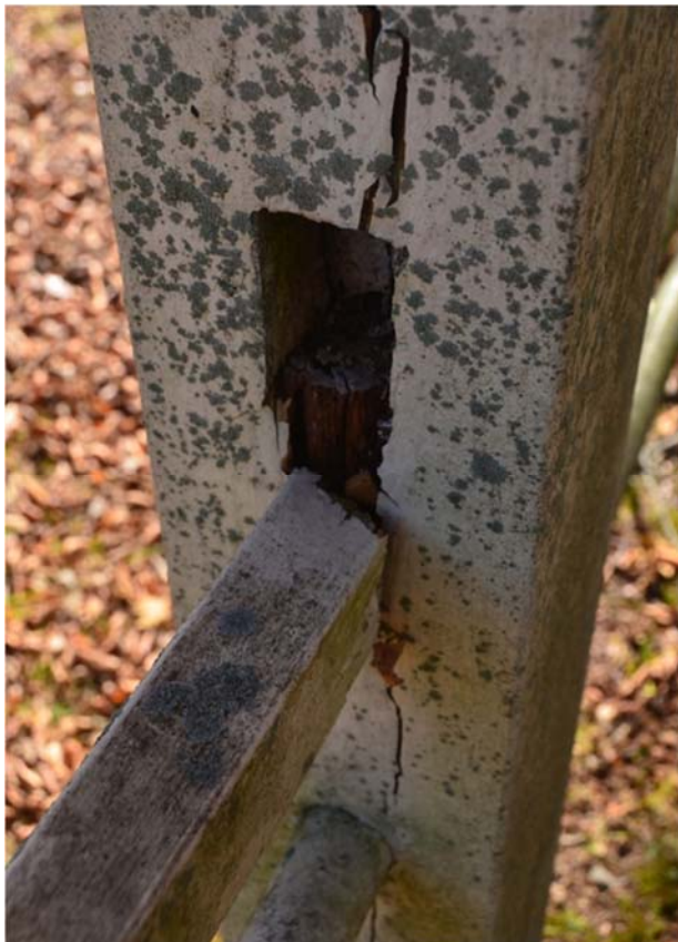
PHOTO 70 Rotted rail pockets.
