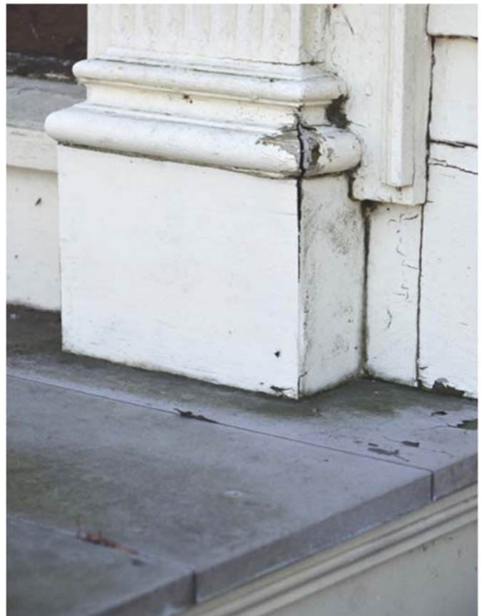
PHOTO 34 View of deterioration at N. Entry steps.
