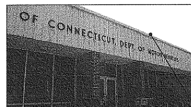
EXISTING FASCIA/D RIP EDGE TO BE REPLACED WITH NEW PREFAB ALUMINUM FASCIA/D RIP EDGE SEE DETAIL AT 3 / A-3. PAINTED TO MATCH EXISTING METAL FASCIA.
