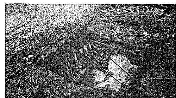
TEST CUT #1 - PLYWD & BLOCKING TO BE REMOVED. KEEP EXIST. BOTTOM BLOCKING. VERIFY SECURE ATTACHMENT. METAL DECK TO REMAIN. REPAIR, REPLACE, FASTEN AS REQUIRED. ALL EXIST BUR ROOFING AND INSULATION BOARDS TO BE REMOVED -SEE DETAIL AT 2/A-3.
