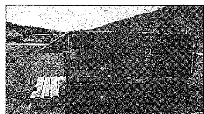
EXISTING AIR HANDLING UNIT TO REMAIN. DISCONNECT AND LIFT UNIT TO INSTALL NEW PREFABRICATED METAL CURB FROM CARRIER - MODEL # CRFCURB047A00. SEE DETAIL AT 1 / A-3. ADD METAL DECKING TO PATCH OPEN AREA. ROOF OVER.
