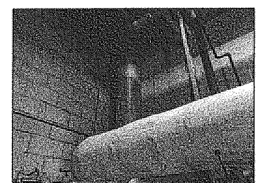
EXISTING PIPES AND FLUE TO BE REPLACED SEE MECHANICAL DRAWINGS - M-1 & M-2.
