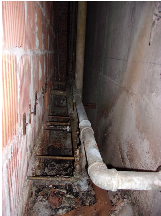
Building 2 – Basement woman's bathroom pipe chase with ACM pipe insulation
