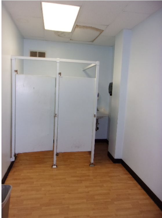
Building 2 - 2 nd floor men's bathroom with wood grain laminate flooring over 12" x12" tan ACM floor tile
