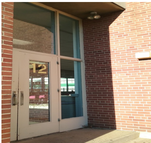
Student Center – Exterior Door with ACM Gray Exterior Door Caulking
