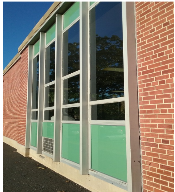
Student Center –Exterior Window System with ACM Interior/Exterior Window Glazing and Tan Window Caulking
