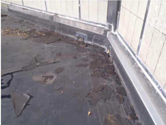
Theatre Roof – Loose ACM Black Roofing Paper Debris from Adjacent Roof System
