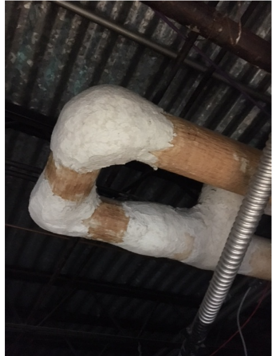
Student Center – ACM Mudded Pipe Fitting Insulation above Suspended Ceiling in Corridor Adjacent to Dining Hall
