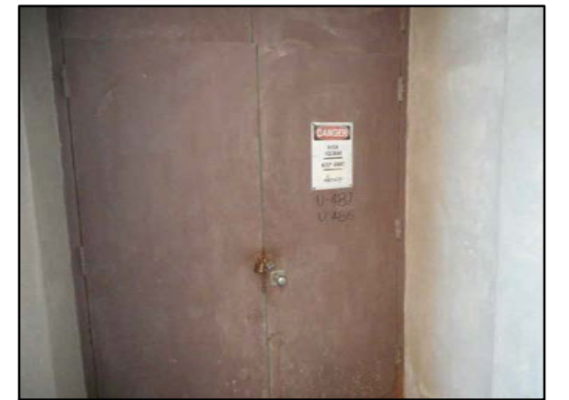
A TRANSFORMER ENTRANCE
