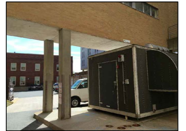
C EXTERIOR GENERATOR
