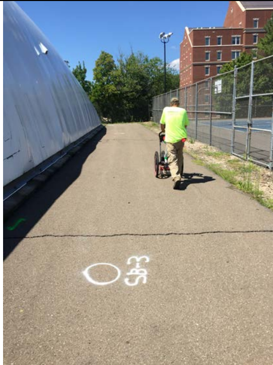
Photo 1: Underground Surveying performing underground utility mark-out near proposed locations for SB-3 and SB-4. Note the sanitary sewer line just south of the proposed borings.
