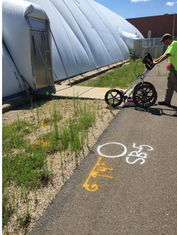
Photo 3: Underground Surveying performing underground utility mark-out near proposed location for SB-5. Note the sanitary sewer line and gas line east of the proposed borings.
