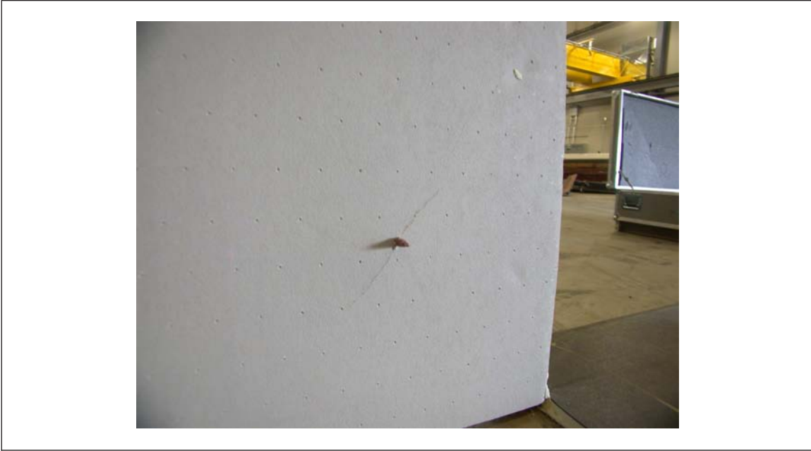
Fig. 4. Crack in underside of cover board at fastener and beneath where crease was visible in the single-ply roof cover
