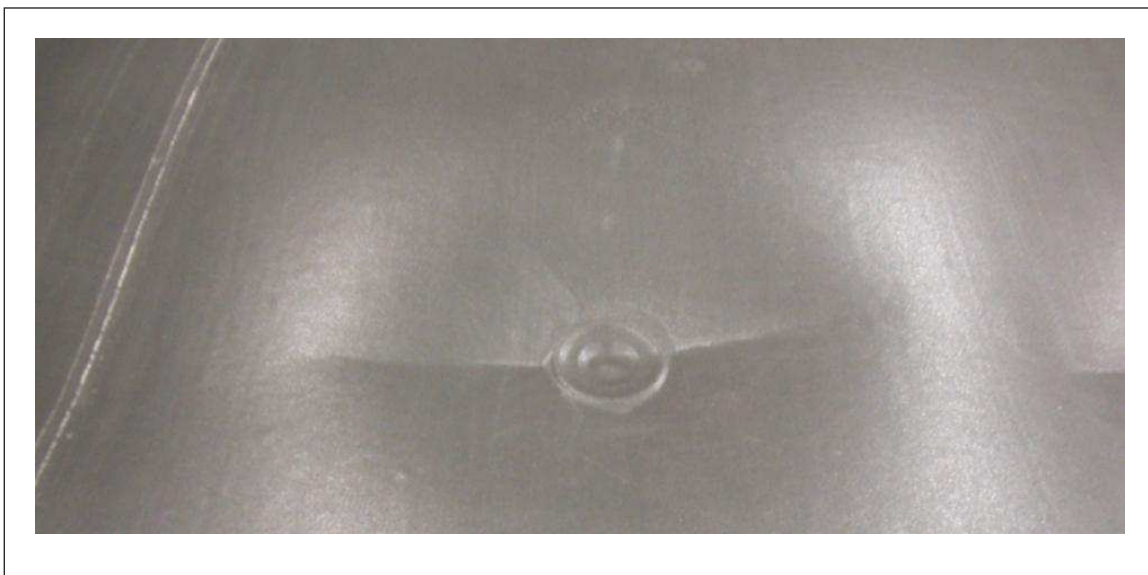
Fig. 3. Crease in single-ply roof cover while subjected to uplift pressure
